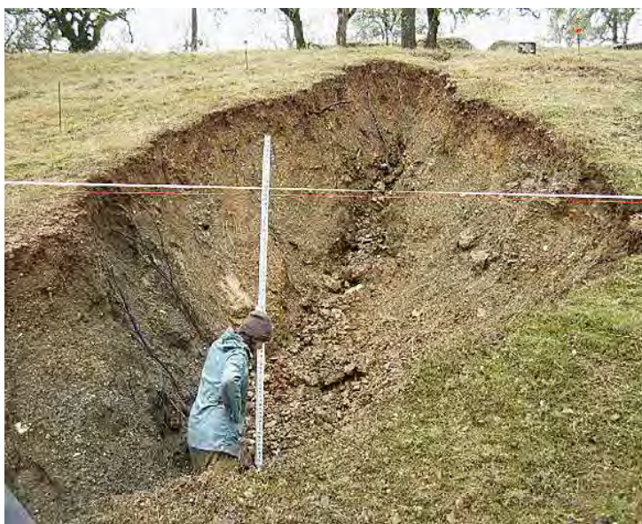
Figure 22. Gully caused by through-cut on road at base of steep road section. Photo: Jared Gerstein.
