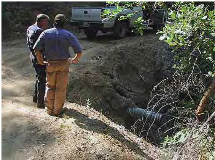
Figure 14. This fill slope erosion was caused by a plugged cross-drain inlet that diverted ditch flow over the road surface. Photo: Angela Wilson, Central Valley Regional Water Quality Control Board.
