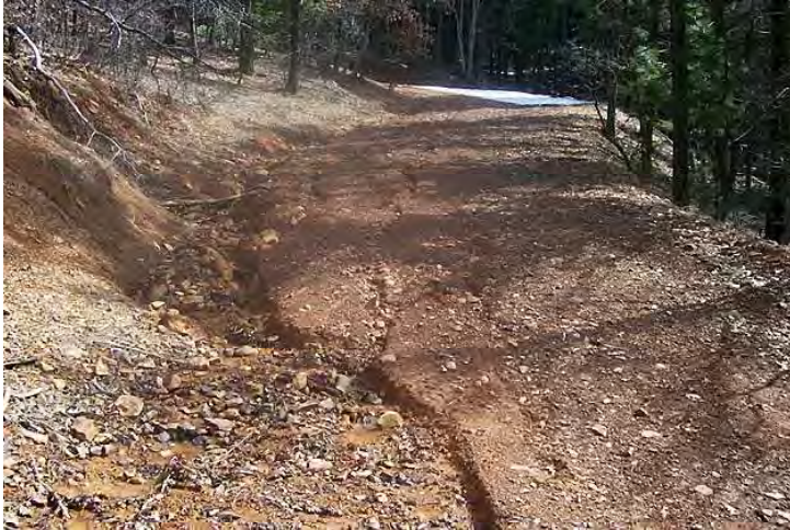
Figure 19. Erosion caused by ditch water leaving the ditch and traveling across the road. Photo: Susan Kocher.
