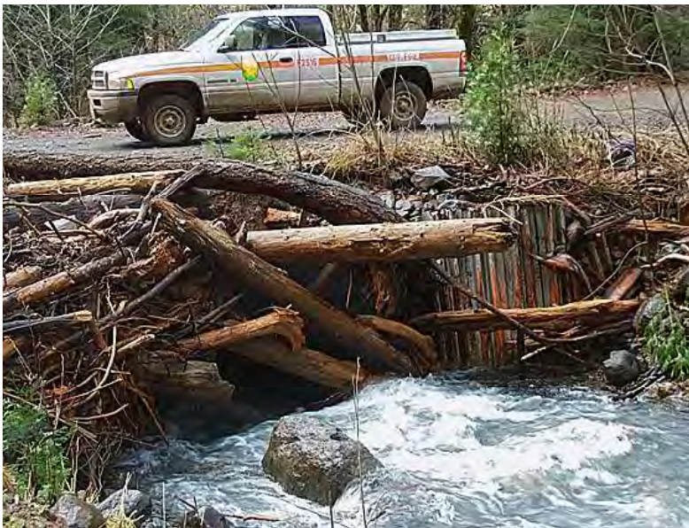
Figure 23. This culvert is nearly plugged by woody debris, endangering the road. Photo: Angela Wilson, Central Valley Regional Water Quality Control Board.
