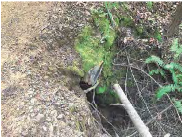
Photo #217, location 53 south side of road 18" cmp outlet.
