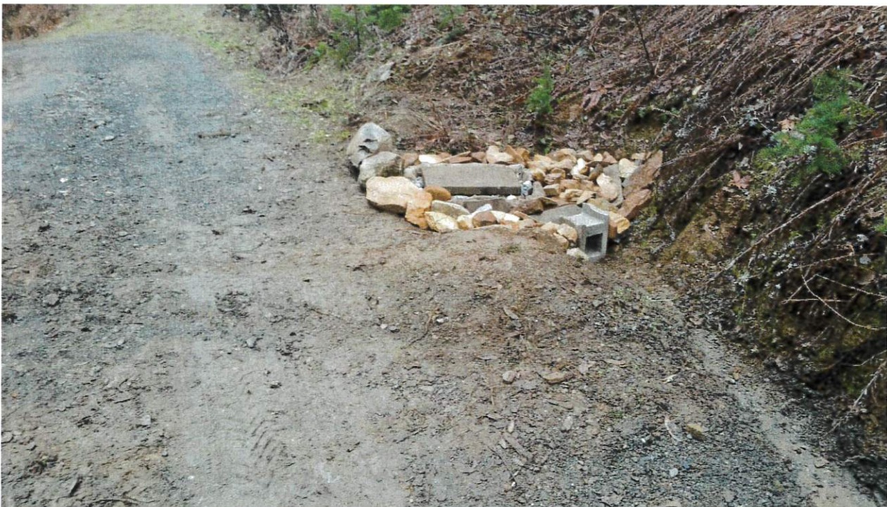
Ditch Relief Culvert 1: Plugged 12" diameter inside ditch relief culvert where surface flows are bypassing the inlet and running down the road resulting in erosion of the roads surface. Replace the ditch relief culvert with an 18" diameter ditch relief culvert and rock armor the inlet and outlet per attached specifications.
