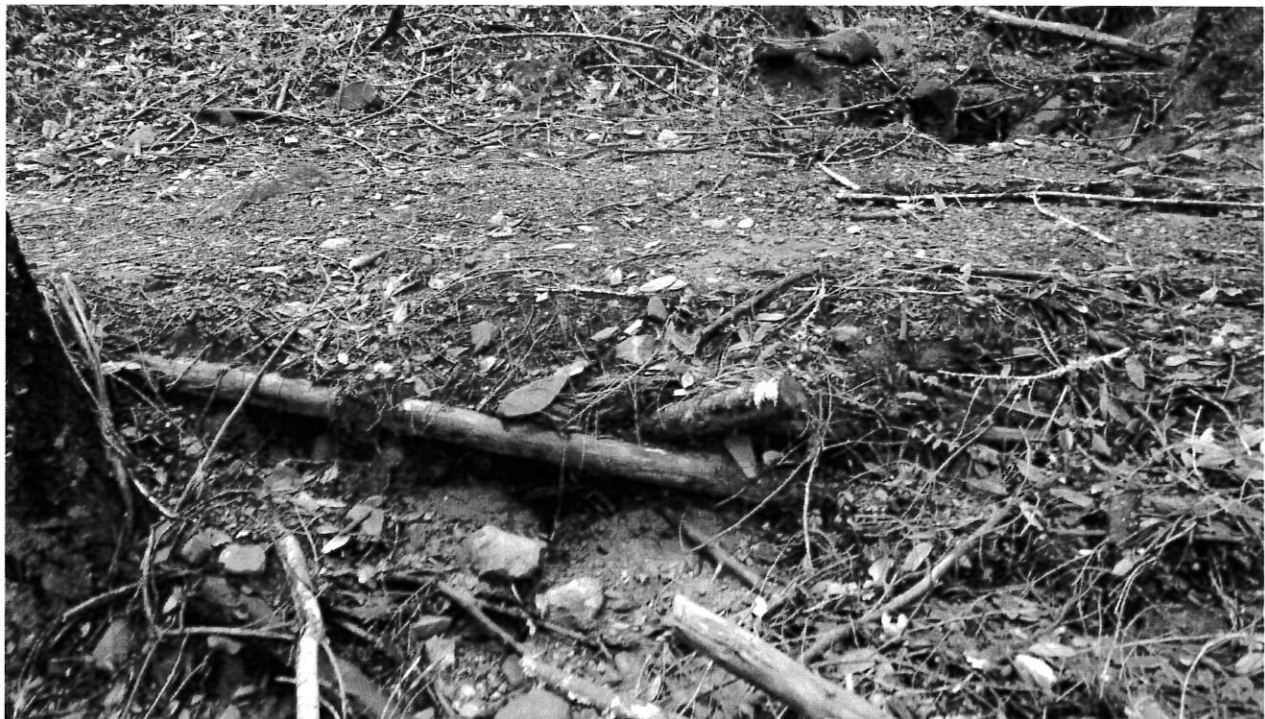
Road Point 2: Plugged 12" drainage ATV crossing that is no longer needed. Remove the crossing and any fill within the drainage.
