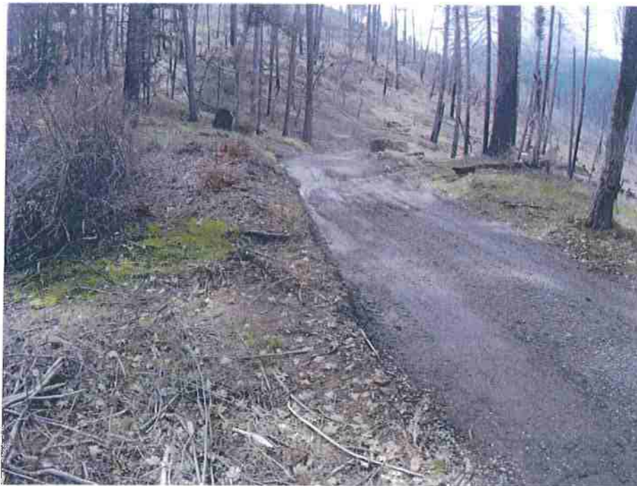
Site 06, Water bar is saturated and not functioning adequately. Proposed mitigation is to establish an inside ditch and install 40ft section of 12" DRC. Inlet will be rocked.
