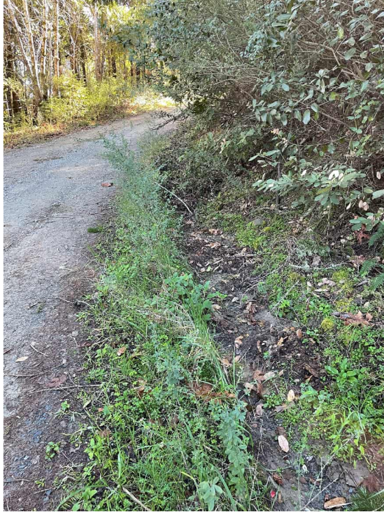
Figure 15: RP 7. Milky Way Loop – Inboard Ditch. Image shown facing south; towards the subject parcel.
