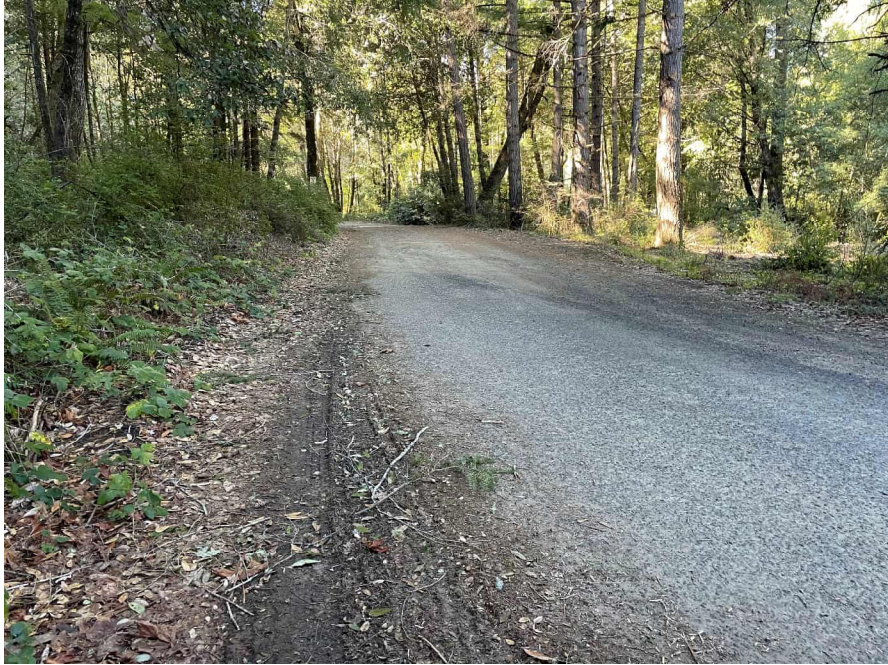
Figure 5: RP2: Milky Way Loop - 16' paved road width; location of 10' turnout. Image shown facing west.
