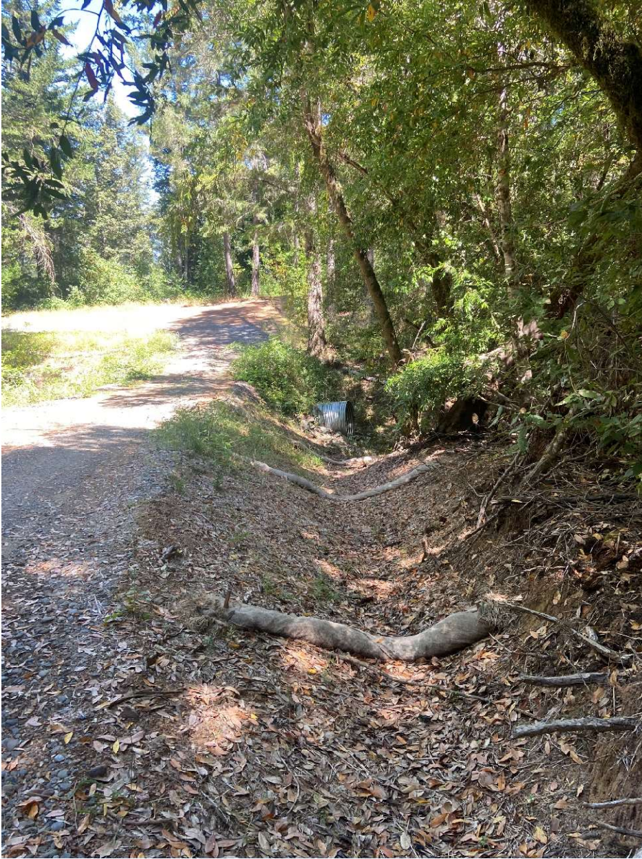
Photo 5 – Recently upgraded culvert on Class II watercourse approaching access road to project area.
