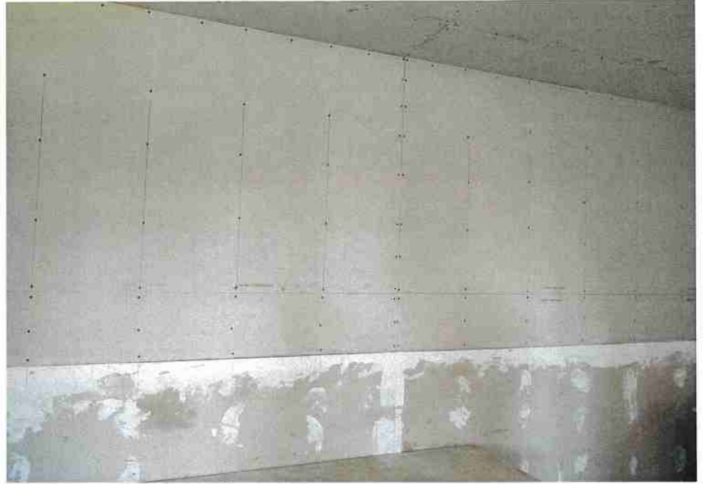
INSIDE PROCESSING AREA 3
