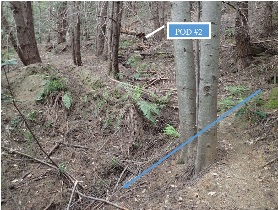
Photo 5 -SC #1; View of the fill crossing on a Class II watercourse (blue arrow) from the left road approach
