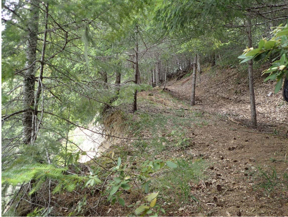
Photo 1 - View of landslide that previously delivered sediment to a Class III watercourse. Note the remaining perched road fill held by small tree roots. Although there is no current delivery, this slide needs to be monitored for movement.
