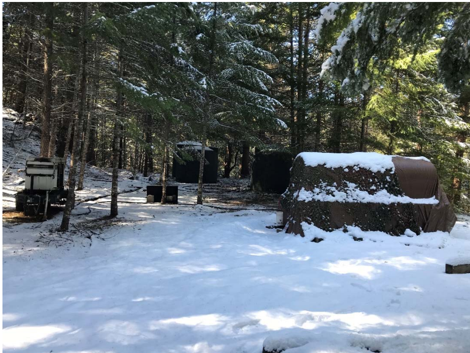
Photo 20 – 1,000 gallon fuel tank and 15,000 watt generator without proper storage or spill prevention measures.
