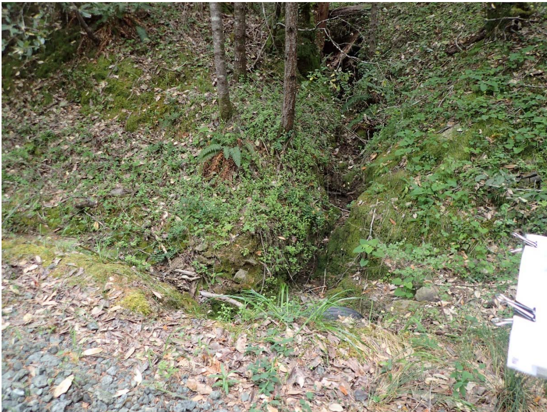
Photo 8 - SC #3; View looking upstream from the inlet of a 24-inch diameter, plastic culvert on a Class III watercourse
