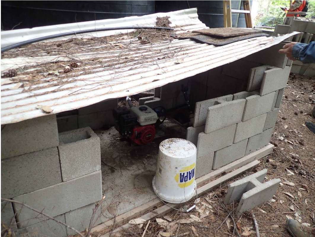
Photo 15 - View of the water pump within the 50 foot riparian buffer of the spring. Note that there is cover provided but no secondary containment.
