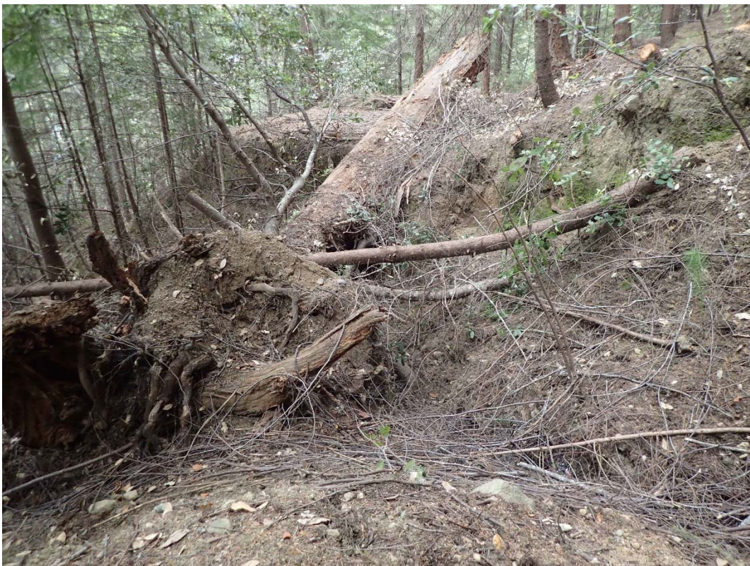
Photo 6 - SC #1; View of a partially washed out fill crossing on a Class II watercourse
