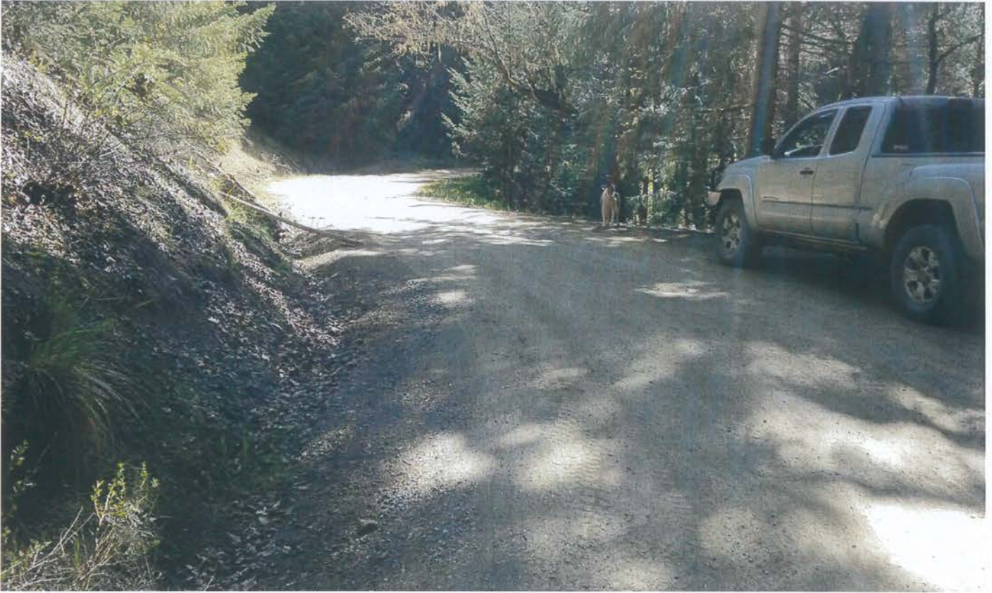
Road Segment 6 to 7: This photo shows the segment of crowned road with an inside ditch from Road Point 6C looking easterly towards Road Point 7. At Road Point 6C, install a rocked rolling dip approximately 30 feet west of the gully below the road. Photo date 4-24-2020.
