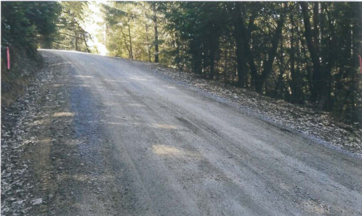
Road Segment 6 to 7: These photos show the lengthy segment of crowned road with an inside ditch from Road Point 6A looking southerly towards Road Point 6B. At Road Points 6A and 6B, install rocked rolling dips or ditch relief culverts to drain the lengthy inside ditch. Photo date 4-24-2020.
