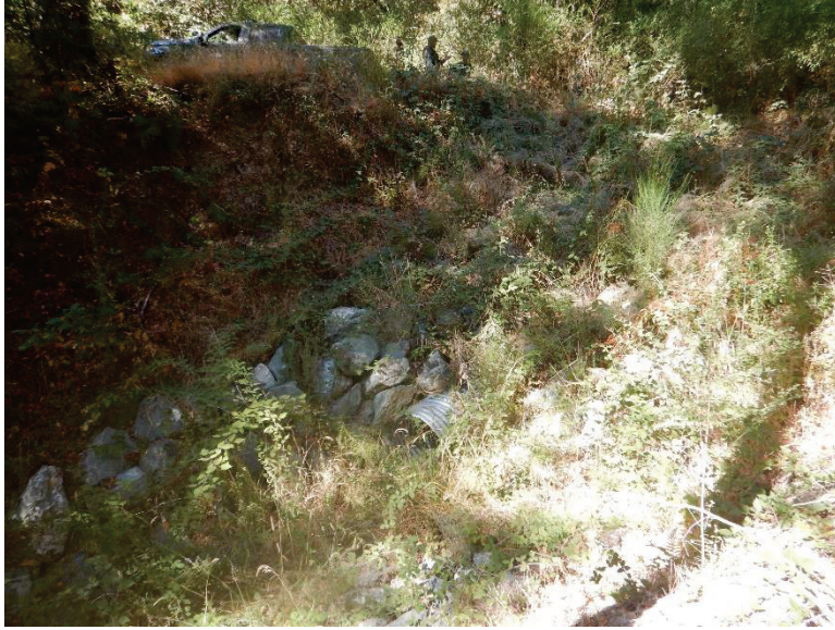
Photo 5 – Unstable Crossing (-123.8172, 40.1230): Sinking fill in foreground and steep cutbank in background. Culvert outlet visible near rocks
