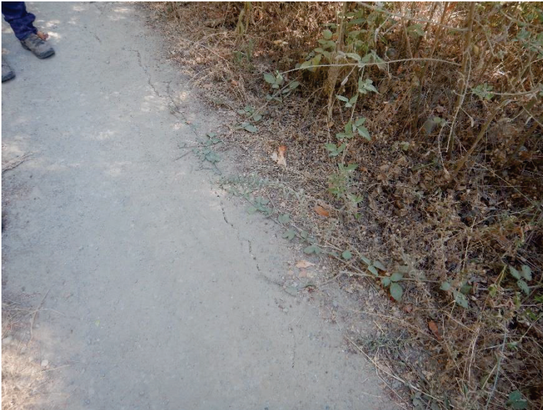
Photo 4 – Unstable Crossing (-123.8172, 40.1230): Crack along road fill surface of culvert stream crossing
