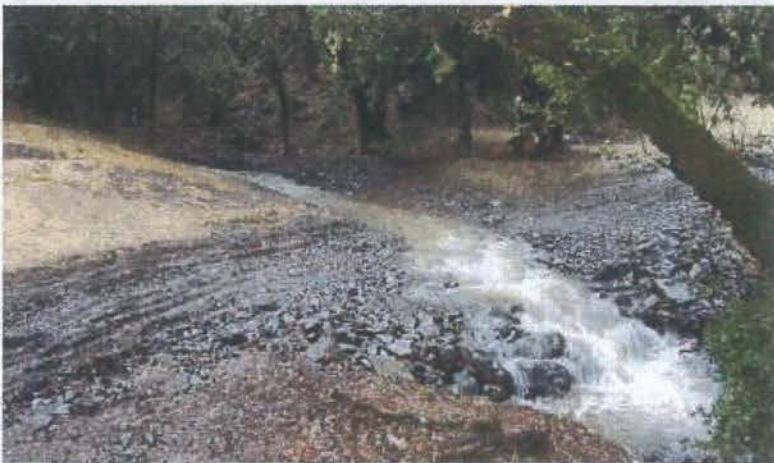
FIGURE 121E. Two weeks after this armored fill was constructed, a storm flow event occurred and the structure maintained its function and integrity. The road approaches had not yet been compacted or surfaced with road rock.
