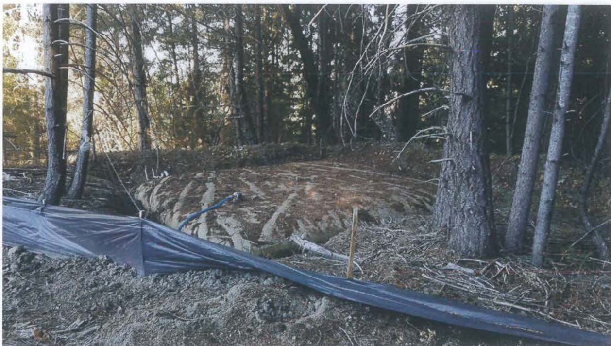
This is an example of a containment pit which will assist in mitigating the impacts if this storage bladder failed.
