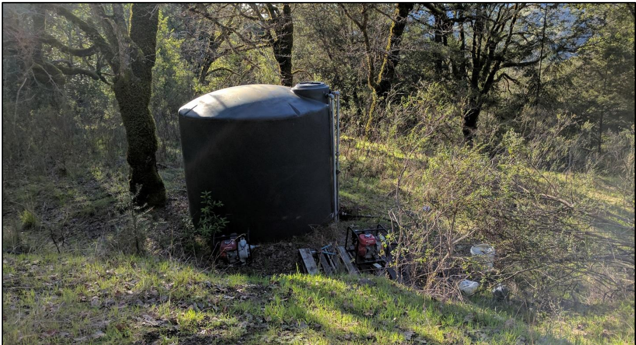
Figure 8: Pressure Pump & Tank
