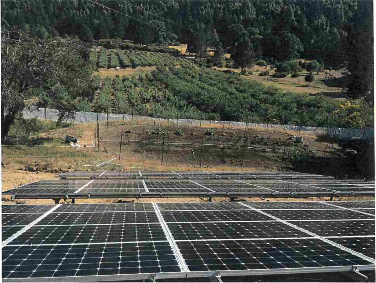
Whitethorn, CA: A 20 kW ground mount grid-tied system powering the home and operations of a local Quince farm.
