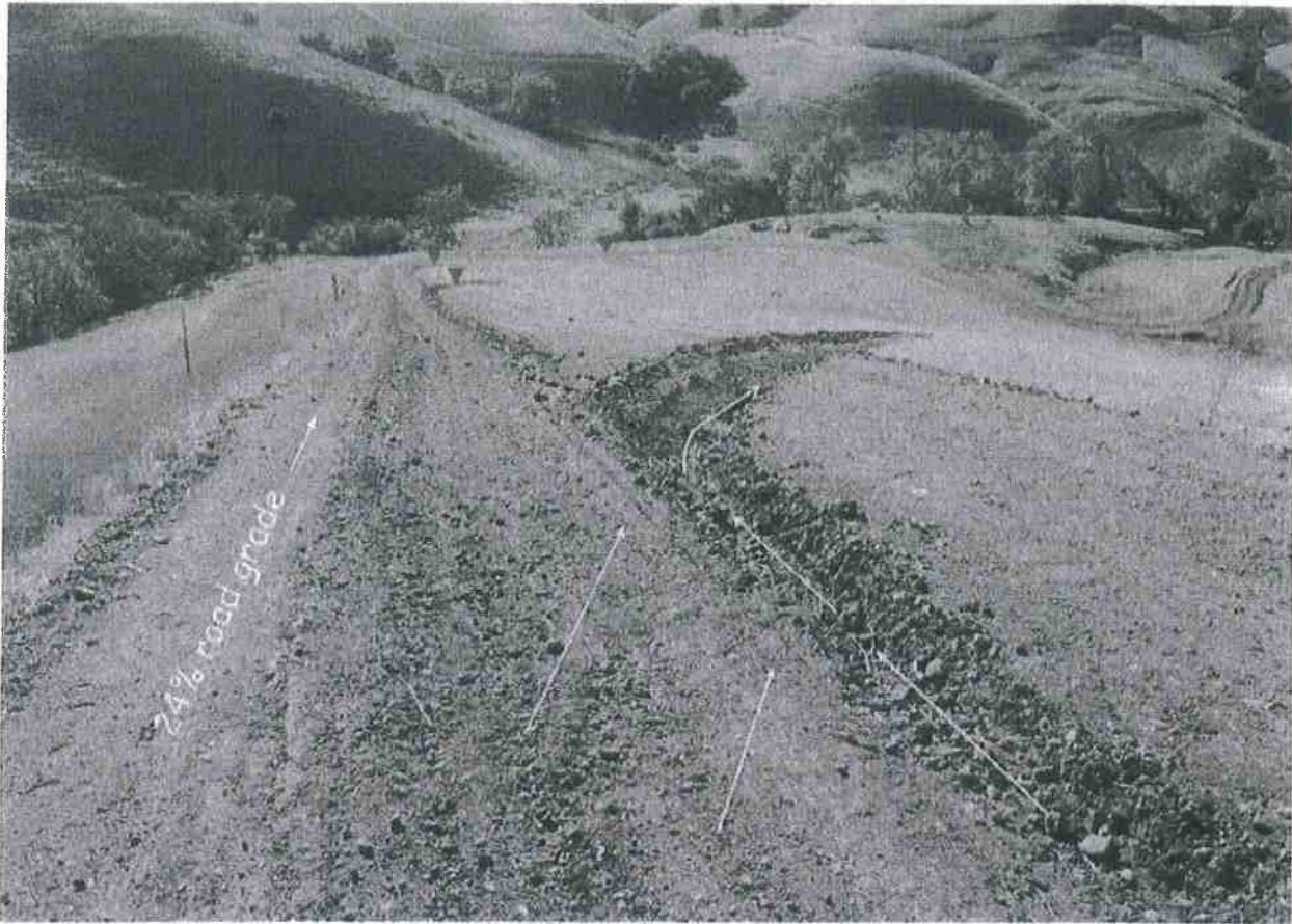
FIGURE 55. Steep roads that go straight up or down a hillside are very difficult to drain. This steep, fall line road developed a through cut cross section that was drained using lead out ditches to direct runoff off the road and onto the adjacent, vegetated hillside. The road was "outsloped" to drain runoff to the right side, and the lead out ditch was built slightly steeper than the road grade, to be self-cleaning. Four lead out ditches have been constructed at 100-foot intervals to the bottom of the hillside.
