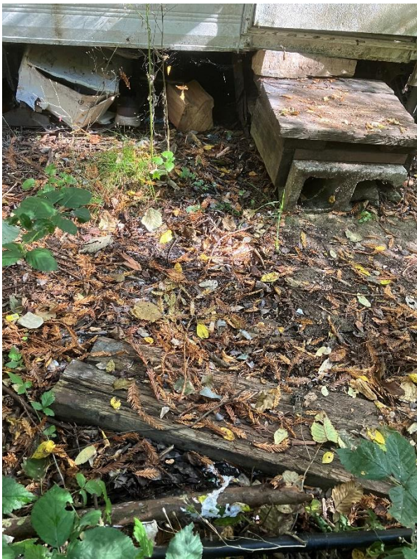
Toilet paper, wastewater and HDPE water distribution pipe
