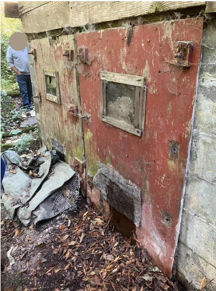
Effluent discharge from privy #91
