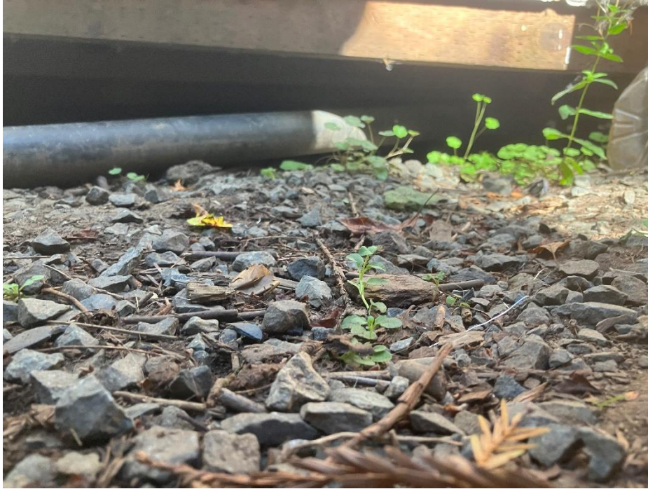
2" discharge pipe to subsurface disposal centrally located wood dwelling
