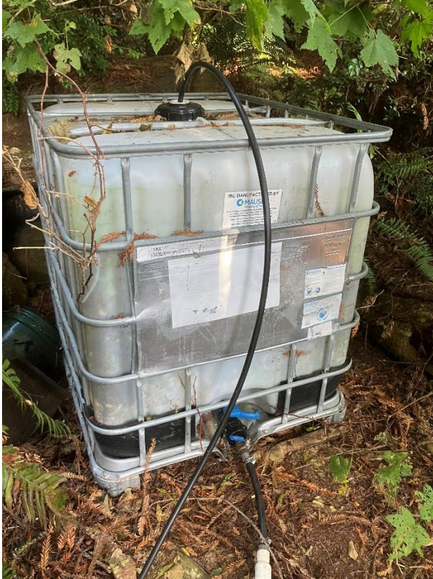
Water storage (~330gal) and HDPE pipe for irrigation or potable system
