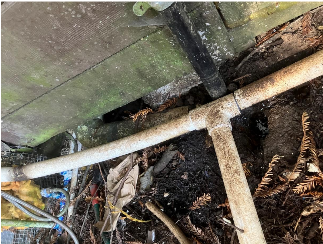
Disconnected 2" drain pipe behind #92
