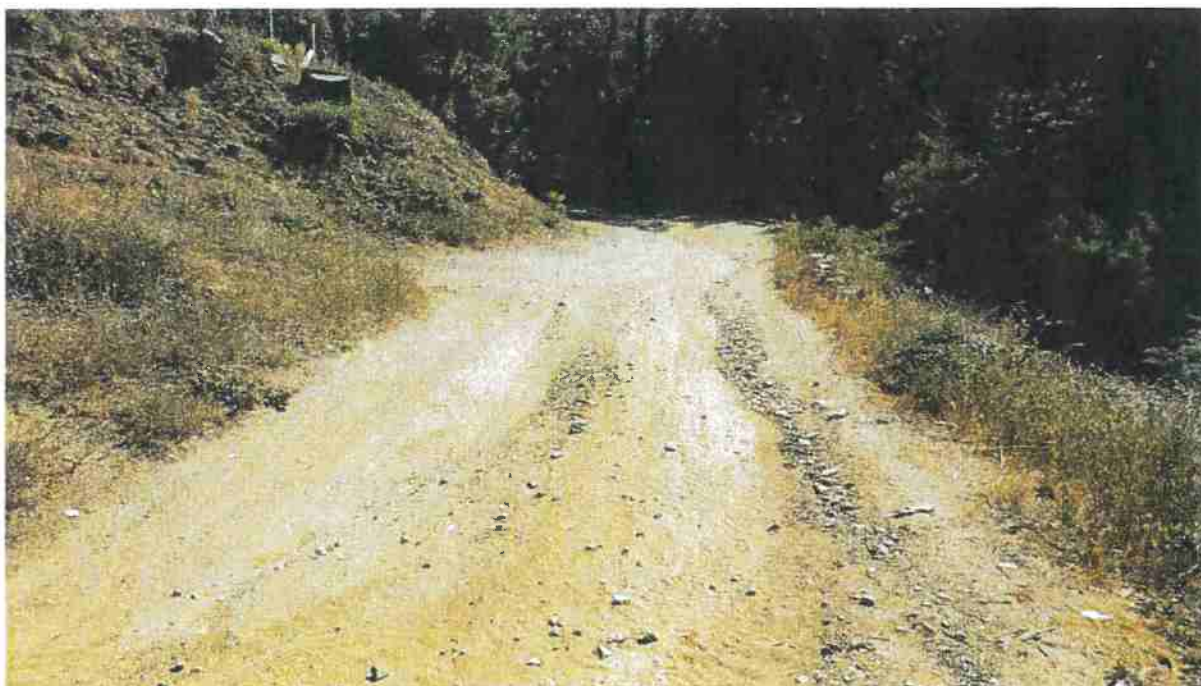
Photo looking up grade at the erosional gully at Site 02.
