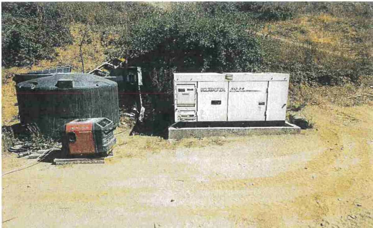
Photo looking at gasoline and diesel generators without proper containment at Site 01.
