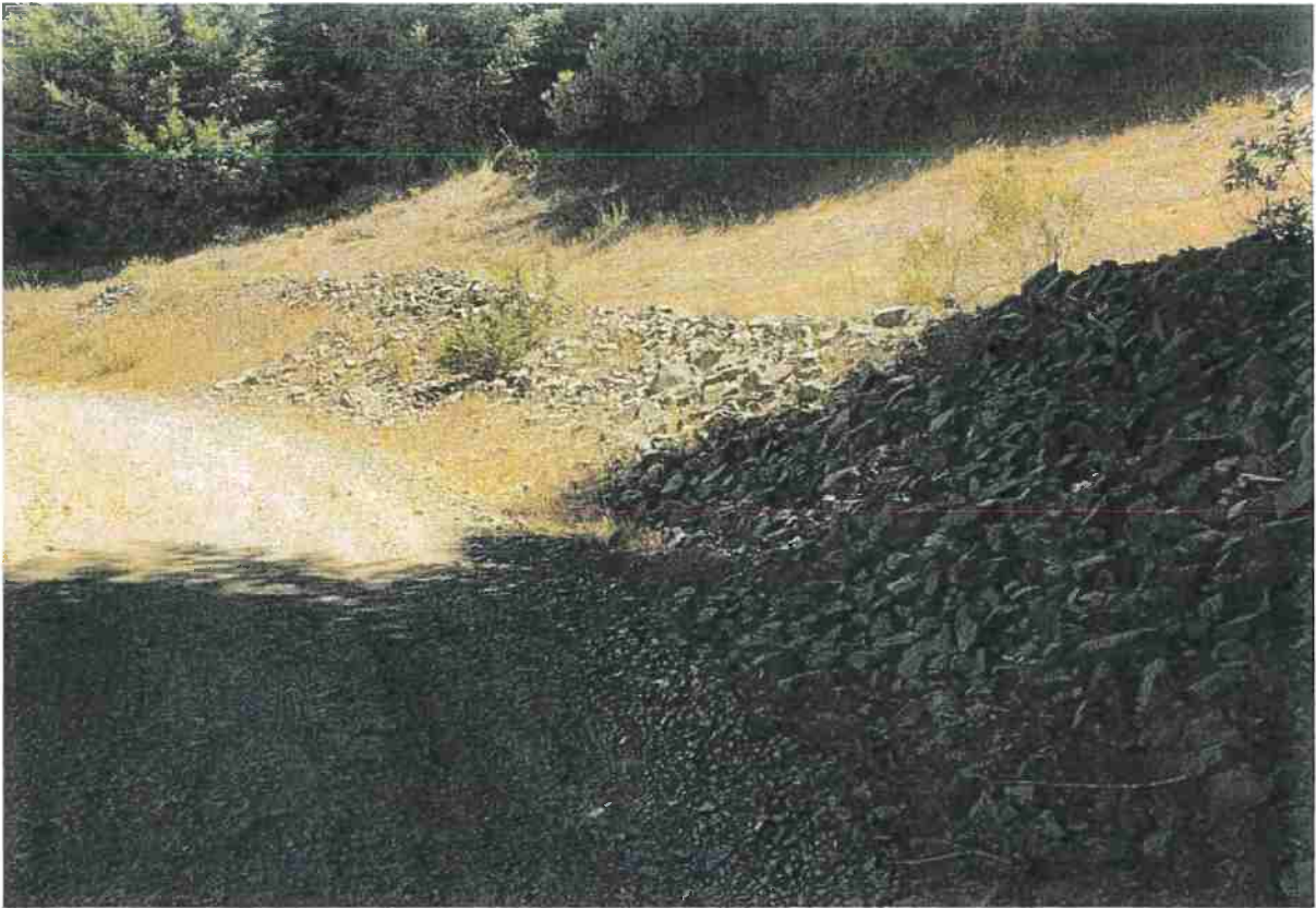
Photo looking at the French drain starting at Site 15 and extending to Site 16.
