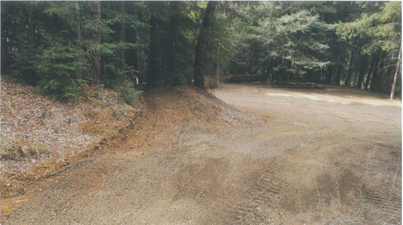
Photo looking down grade at one of several drainage features installed at Site 10. This drainage feature is a Kickout/inside ditch lead-out ditch. Two other drainage features are installed up grade of this site (not shown) that consist of rocked rolling dips/lead-outs.
