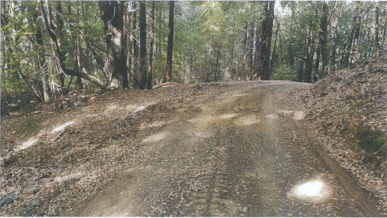
Photo looking down grade at a waterbar installed at Site 06. I advised the cultivator to touch up the waterbars recently installed on the roads around the property to increase their depth for proper function.
