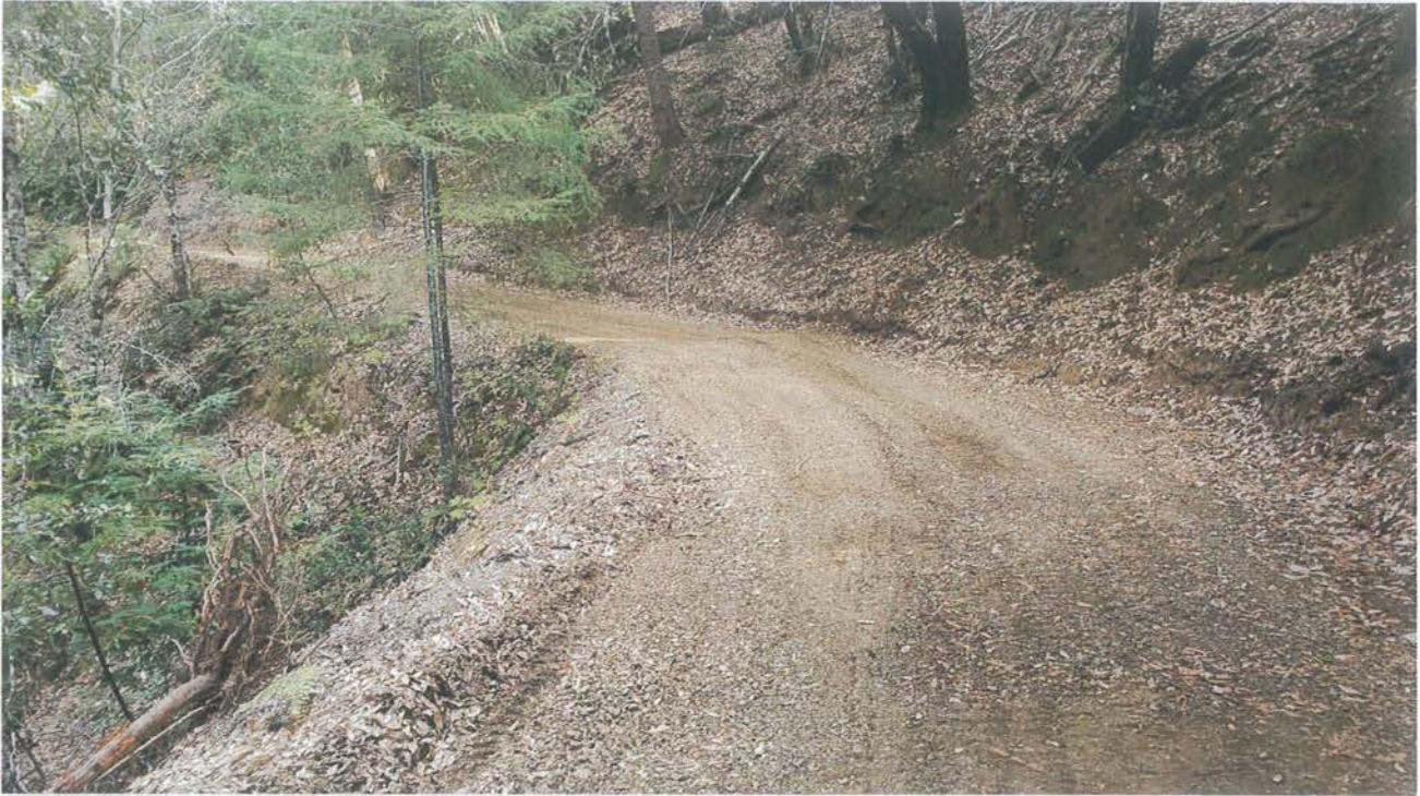
Photo looking up grade at a waterbar installed at Site 15.
