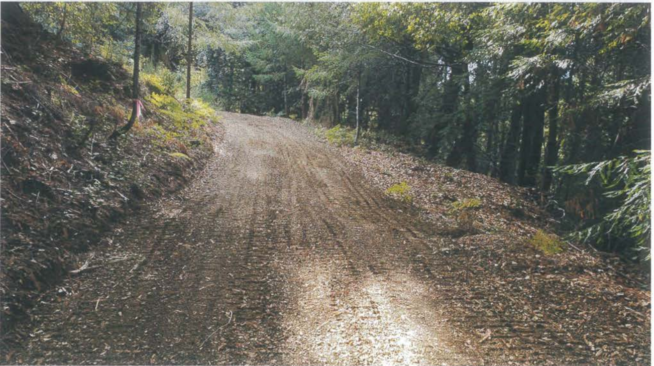
Photo looking up grade at a rolling dip installed on the lower legacy road below, to the west of, Site 15.
