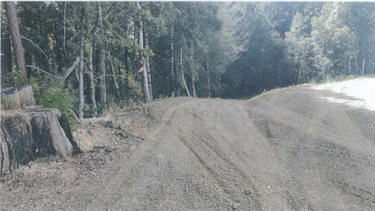
Photo look down grade at a rolling dip/outsloping installed to drain the adjacent greenhouse flat up grade of Site 07.
