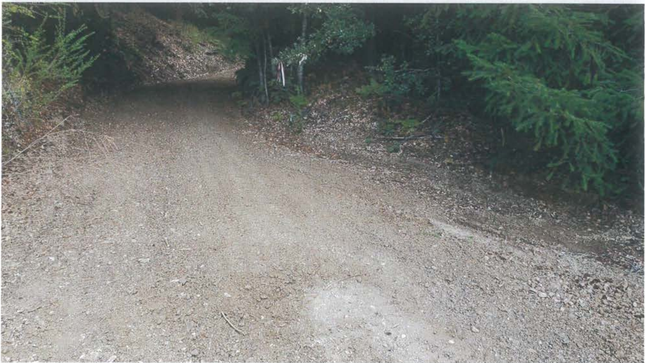
Photo looking up grade at a rolling dip installed on the lower legacy road below, to the west of, Site 15.
