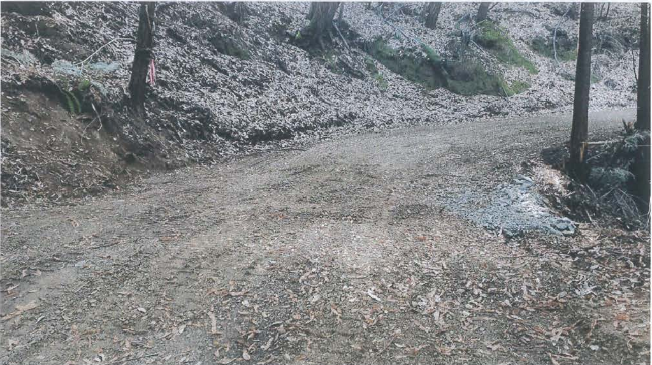
Photo looking up grade at a rolling dip installed on the lower legacy road below, to the west of, Site 15.
