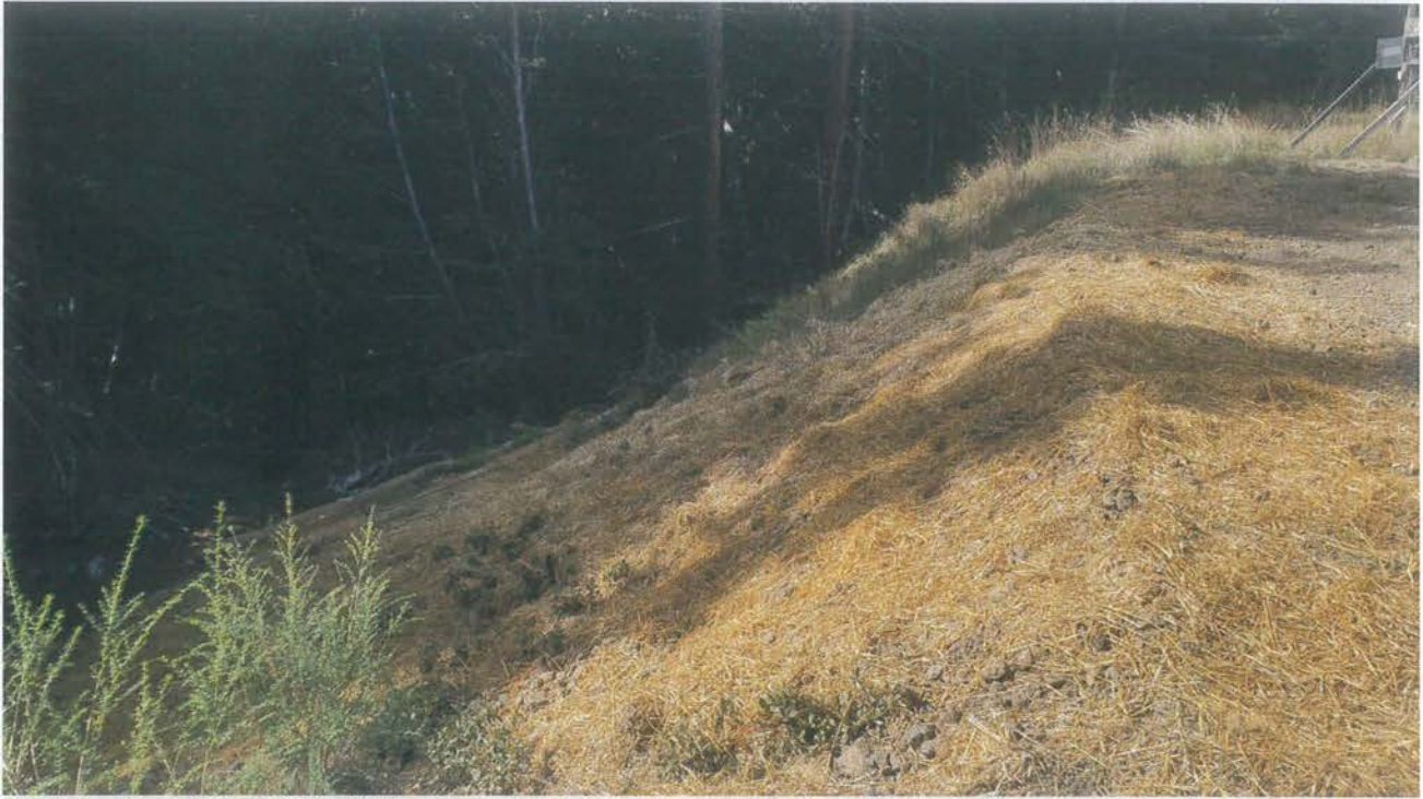
Photo looking at Site 08. The fillslope here was laid back, compacted, and treated with erosion control measures.
