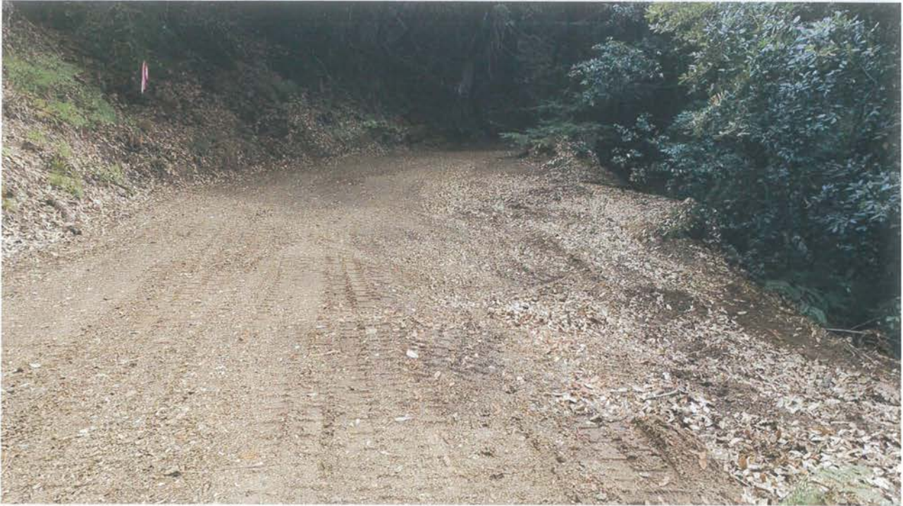
Photo looking up grade at a rolling dip installed on the lower legacy road below, to the west of, Site 15.
