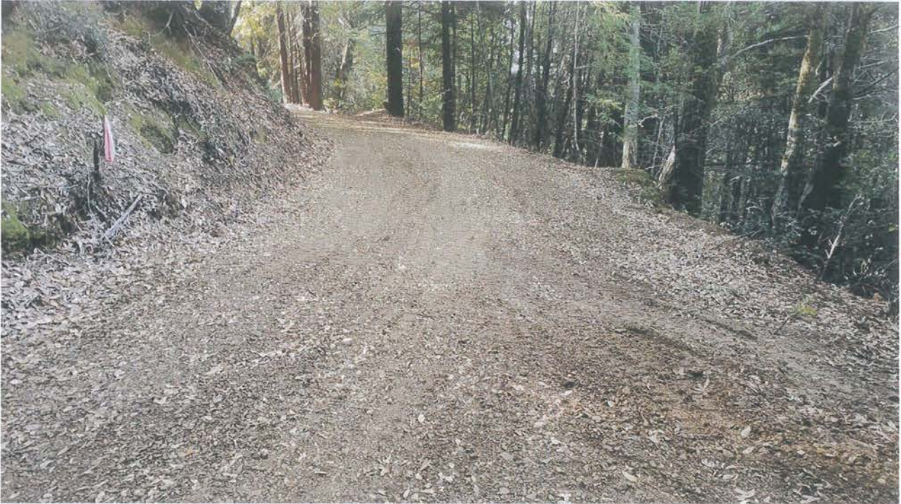
Photo looking up grade at a rolling dip installed on the lower legacy road below, to the west of, Site 15.
