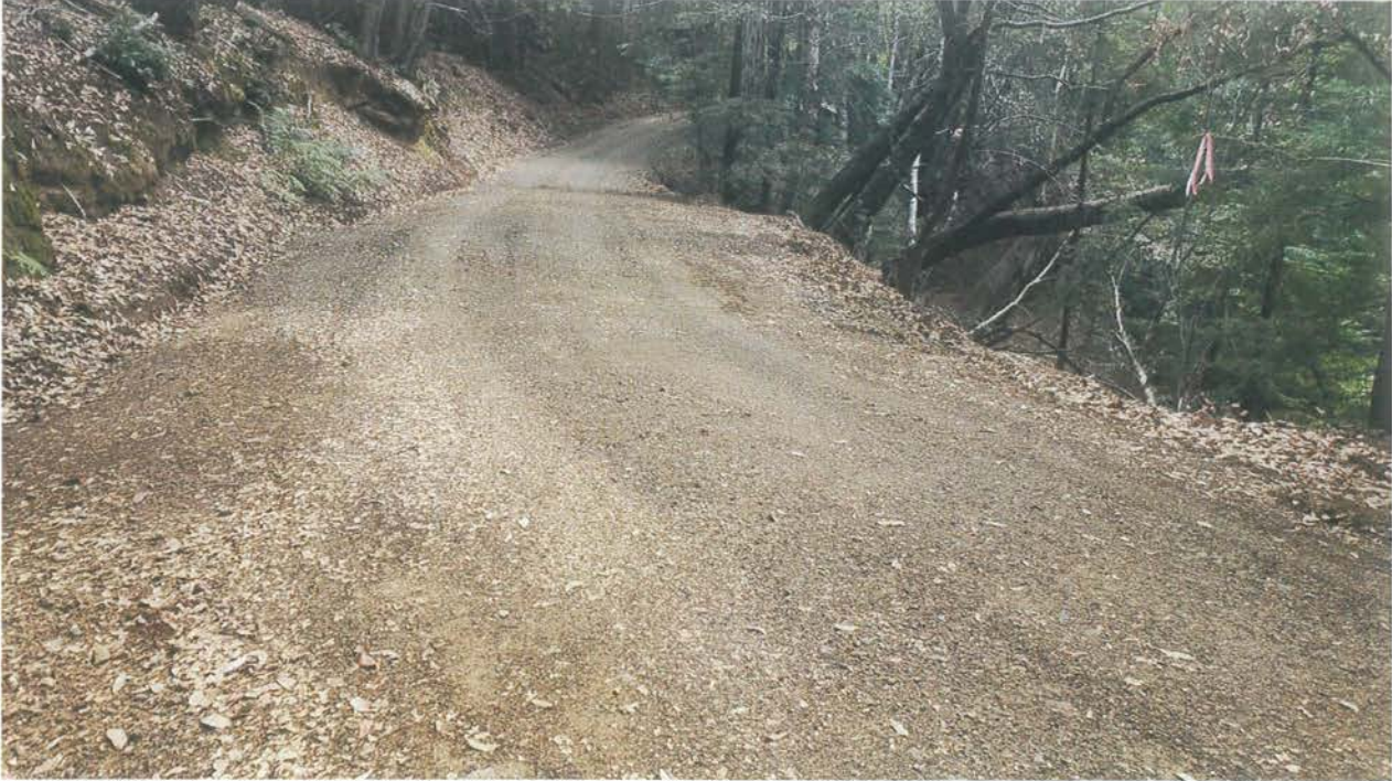
Photo looking up grade at Site 04 with Site 05 further down the road in the photo.
