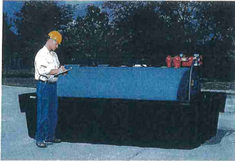
Example of secondary containment for a fuel tank. This container requires cover from precipitation.
