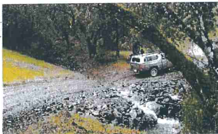
FIGURE 121F. The same armored fill as it appeared after the first winter flood flows. No maintenance was required to reopen the road. It is also clear that no stream diversion is possible at this stream crossing site, and the volume of fill within the crossing has been reduced to the minimum amount needed to maintain a relatively smooth driving surface on this low volume road.
