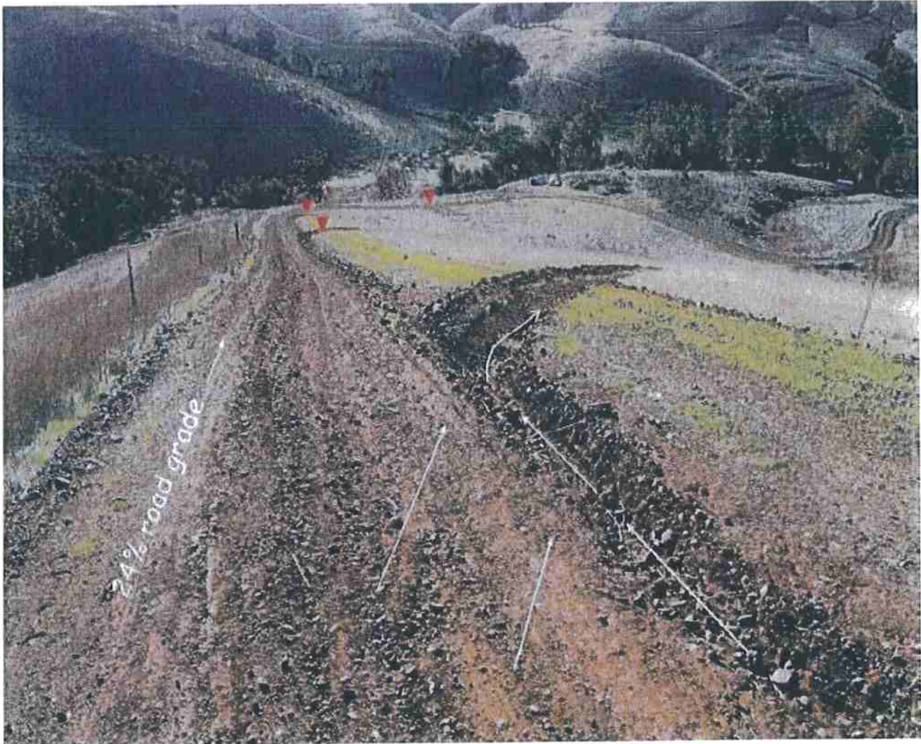
FIGURE 55. Steep roads that go straight up or down a hillside are very difficult to drain. This steep, fall line road developed a through cut cross section that was drained using lead out ditches to direct runoff off the road and onto the adjacent, vegetated hillside. The road was "outsloped" to drain runoff to the right side, and the lead out ditch was built slightly steeper than the road grade, to be self-cleaning. Four lead out ditches have been constructed at 100-foot intervals to the bottom of the hillside.
