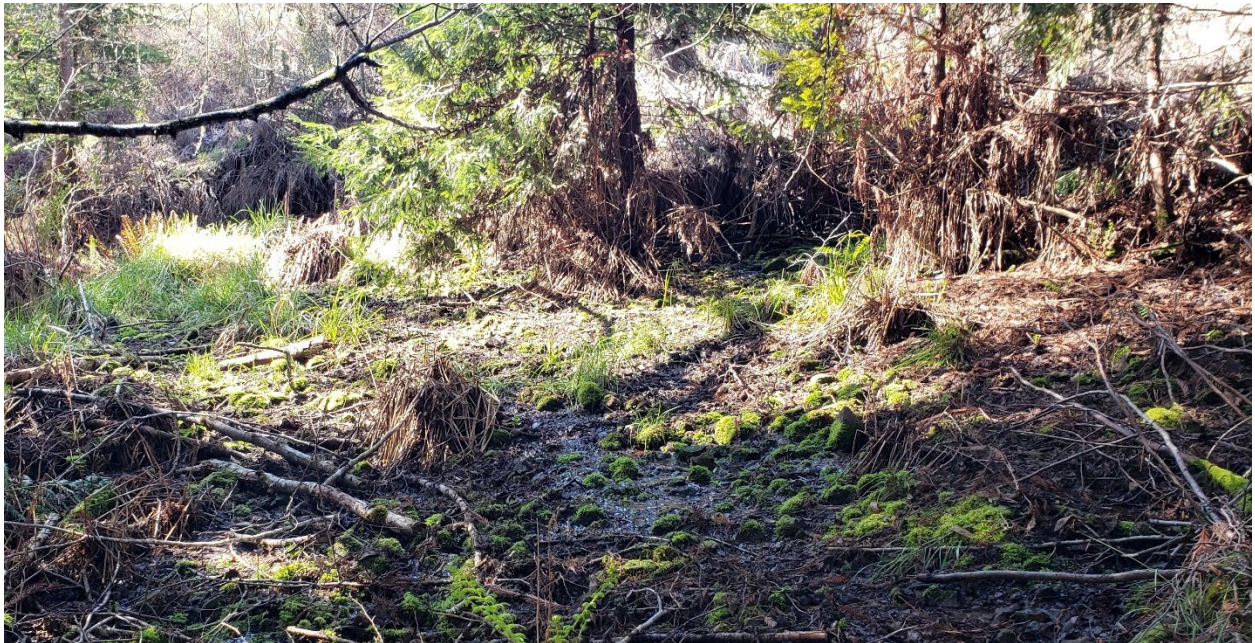
Photo looking southwest toward the impoundment overflow structure outlet and downhill fillslope toe of the impoundment at WQ-5, which is behind the redwood trees to the right, from PM 11. March 2 nd , 2021
