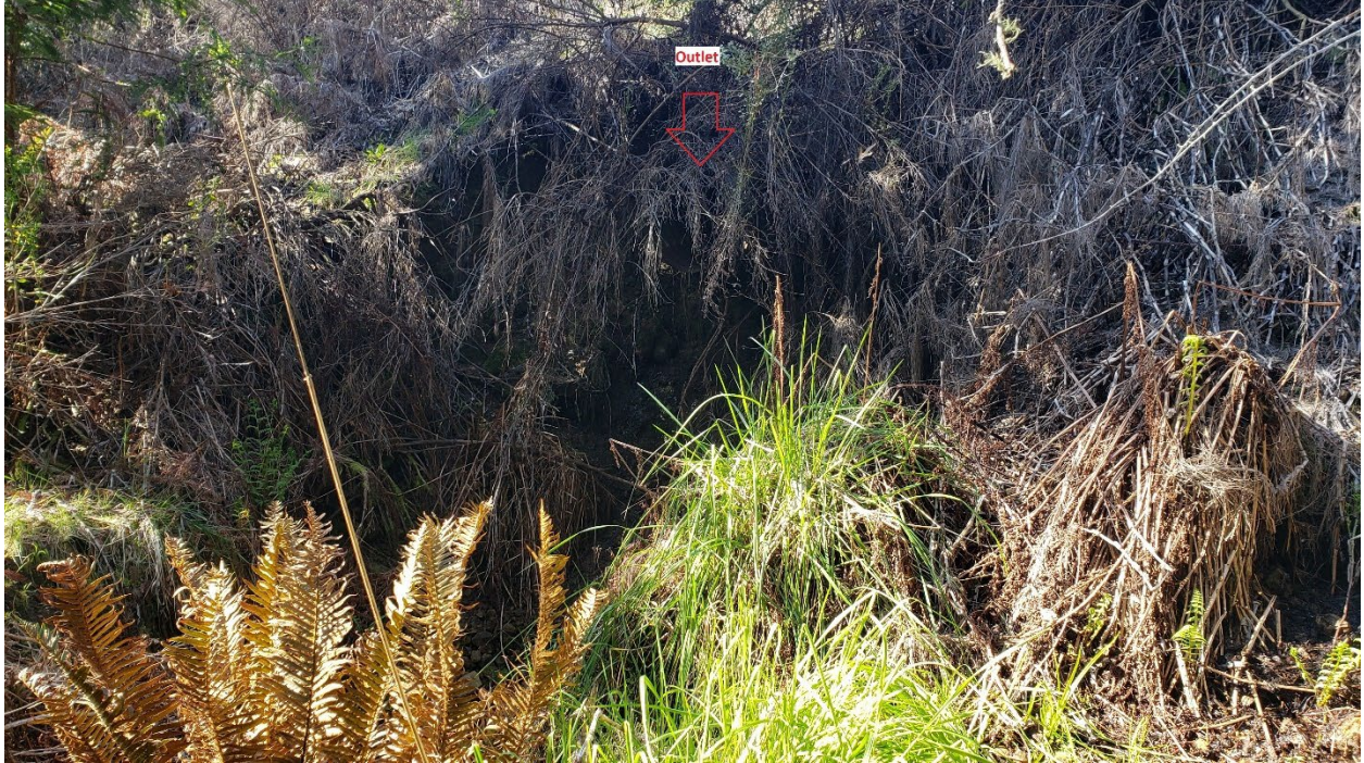
Photo looking southwest directly at the impoundment overflow structure outlet and downhill fillslope toe of the impoundment at WQ-5 from PM 11. March 2 nd , 2021
