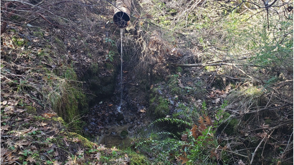
Photo looking west at the impoundment overflow structure outlet at WQ-9. March 2 nd , 2021
