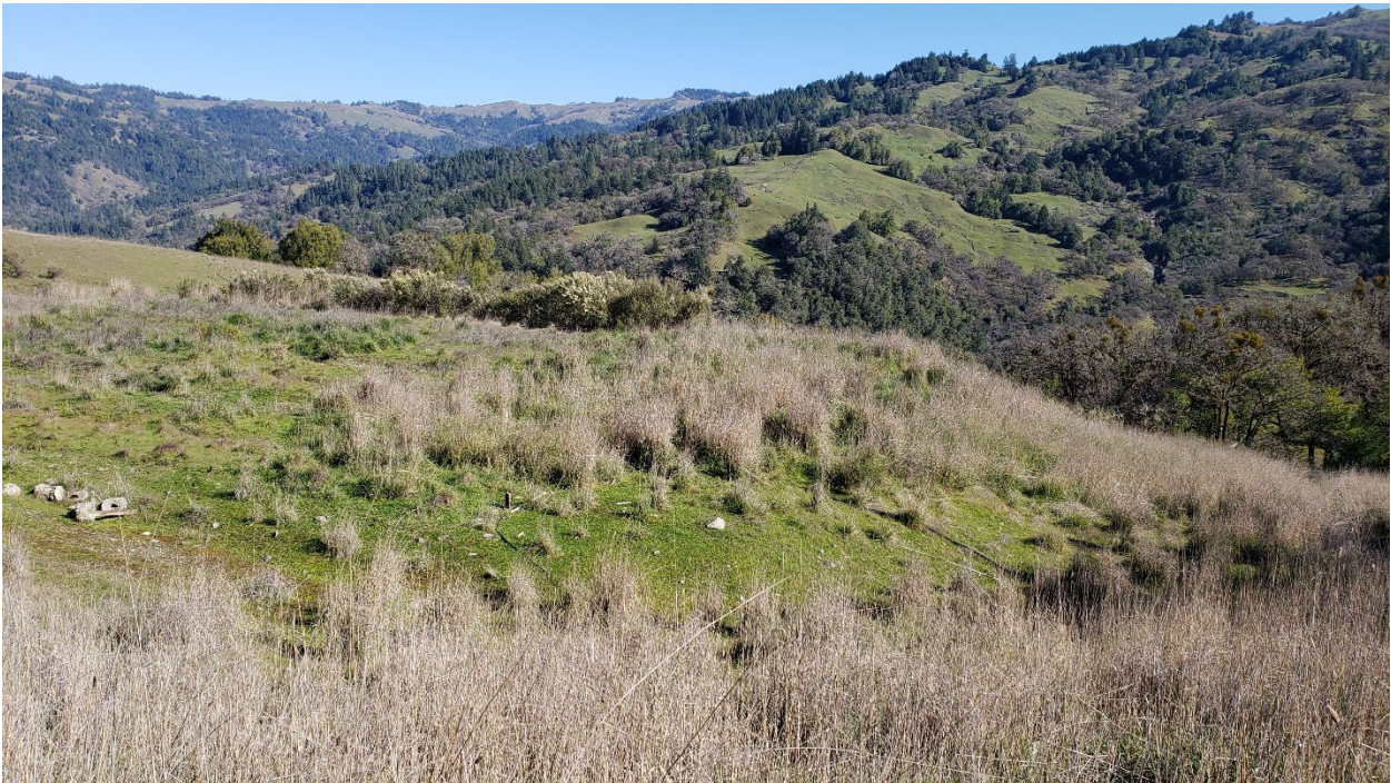
Looking east at the southern edge of the graded area at Site E. This southern edge will be removed (fill pulled back and contoured into the graded area) and the watercourse restored that is underneath it.
