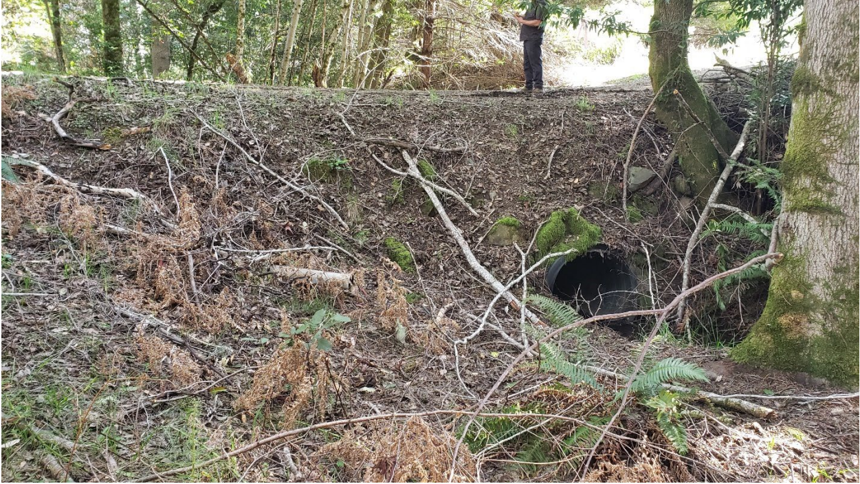
Photo looking southeast at the inlet of the watercourse crossing at WQ-7 from PM 14.
