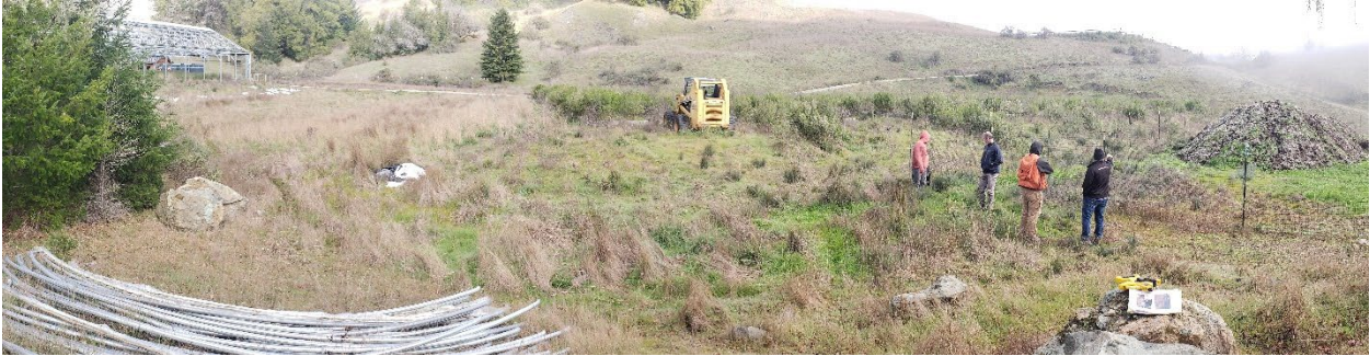
Panorama photo looking northwest to the northeast at the entire WQ-1 work area from PM 3. March 2 nd , 2021
