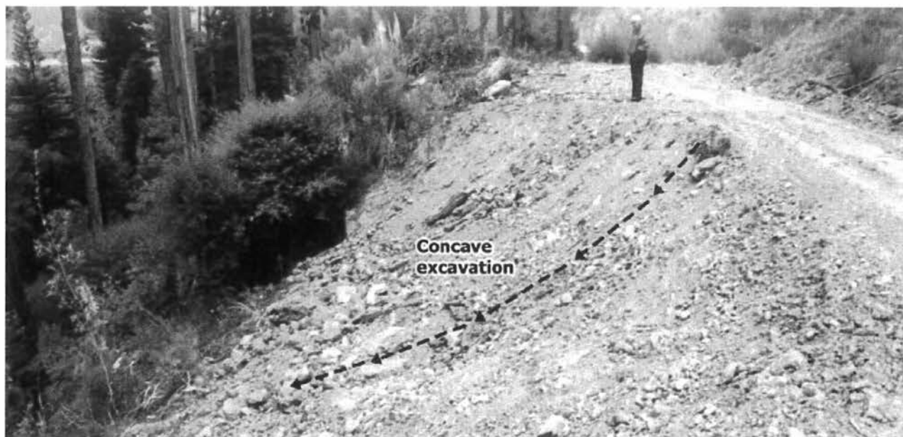
FIGURE 230. The most cost-effective treatment for unstable fills along the outside of a forest, ranch or rural road is simply the direct excavation of the unstable material. If road width is too narrow, additional width can often be derived from cutting into the bank. The excavation should encompass the unstable fill materials, beginning at the inside crack or scarp, and extending out and down the fill slope as far as possible. For proper surface drainage, and to retrieve most of the unstable fill, the excavation should have a concave profile when completed. Typically, the bulk of the fill is within 20 to 25 feet of the outside edge of the road and is easily reached by a midsized excavator. Any remaining fill is likely to be small enough that it will not fail or travel far enough to reach the stream.
