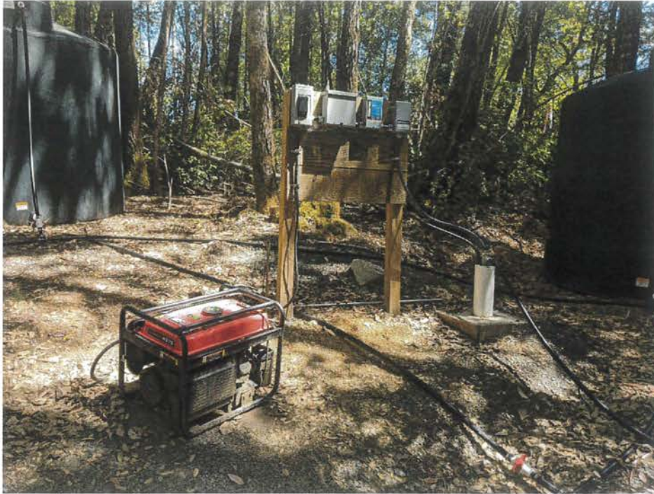
Groundwater well located on the north portion of the property.
