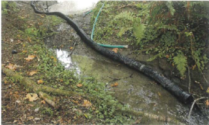
FIGURE 197. Flex pipe stream diversion around a road construction site. The inlet to this 6 inch diameter flex pipe inlet collects clear streamflow from a retention dam above the project site and gravity feeds it around the project area and back into the natural channel downstream from construction work (see photo).
