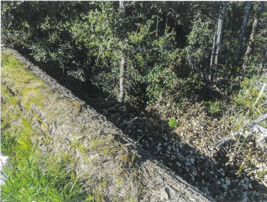
Fill slope of the lower terrace of Cultivation Area C. Minor surface cracking was identified and shall be monitored regularly.
