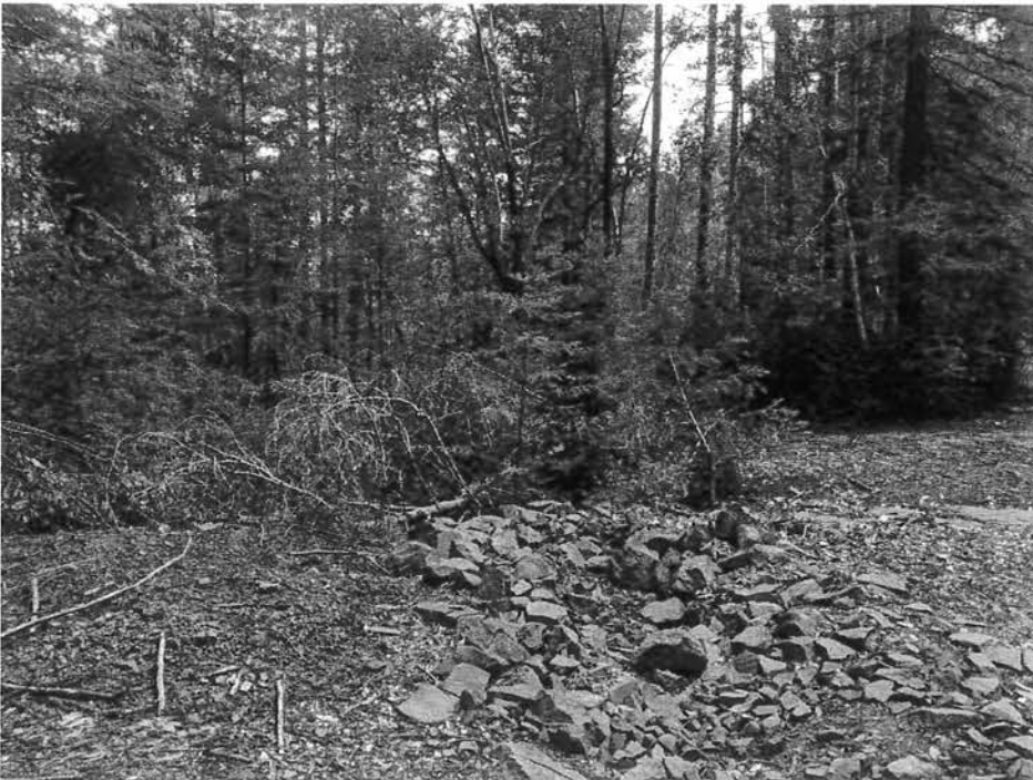
Existing rocked ford crossing that shall be upgraded to a rock armored fill crossing.
