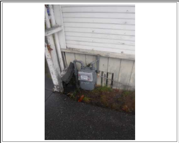
Gas Meter Utility
