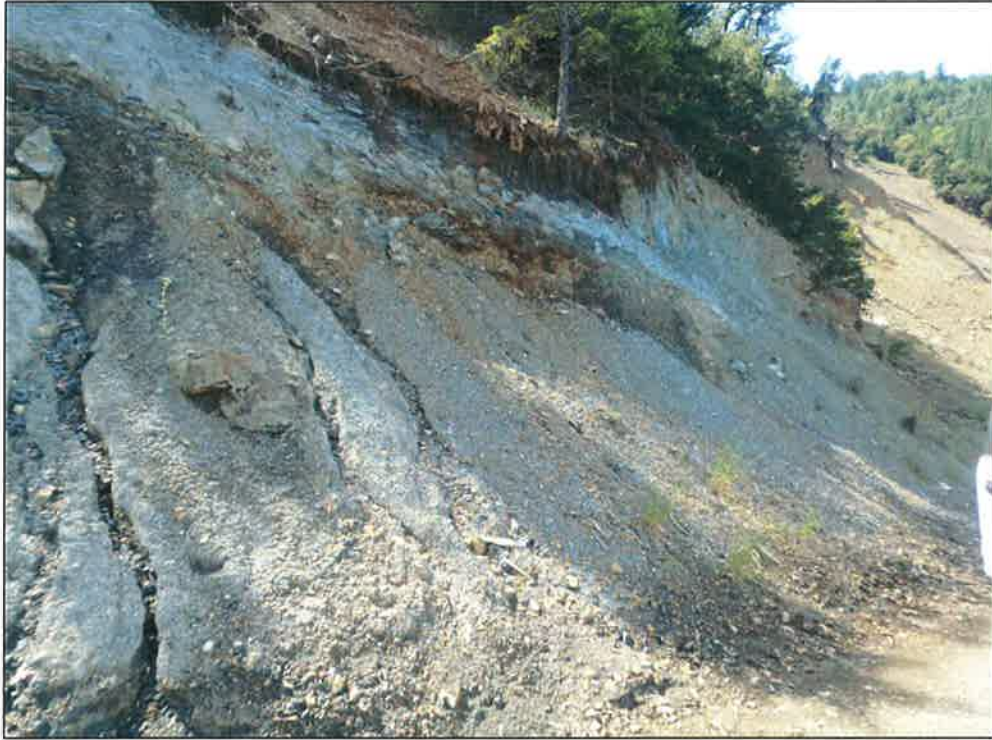
Deeply weathered serpentinite and overlying colluvium along haul road
