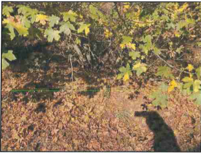
Photo #301 River Rd Looking @ Partially Clogged 24" Culvert In
