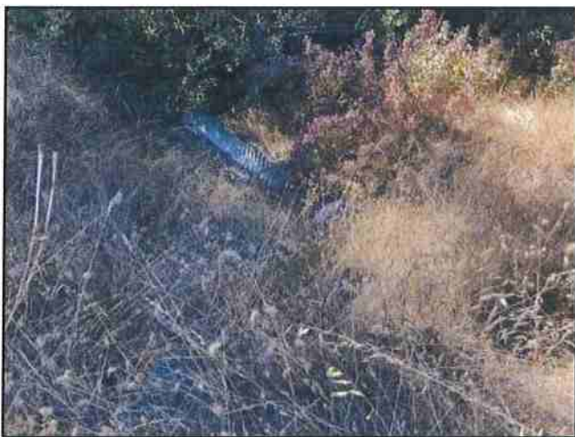
Photo #389 River Rd 24" Culvert Out
