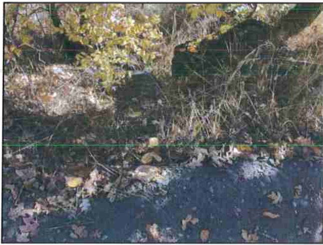
Photo #49 River Rd 12" Culvert Out
