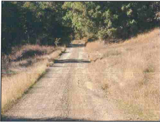
Photo #325 River Rd Looking NE @ Hillside Slip Creating Drainage Issue and Rutting
