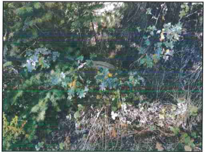
Photo #176 River Rd Looking @ Partially Clogged 36" Culvert In
