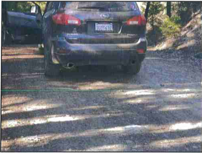
Photo #319 River Rd Looking NE @ Curve w/ Pullout & Tire Rutting
