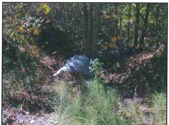
Photo #354 River Rd 36" Culvert Out
