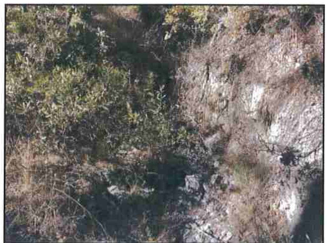
Photo #90 River Rd Looking @ Clogged 24" Culvert In
