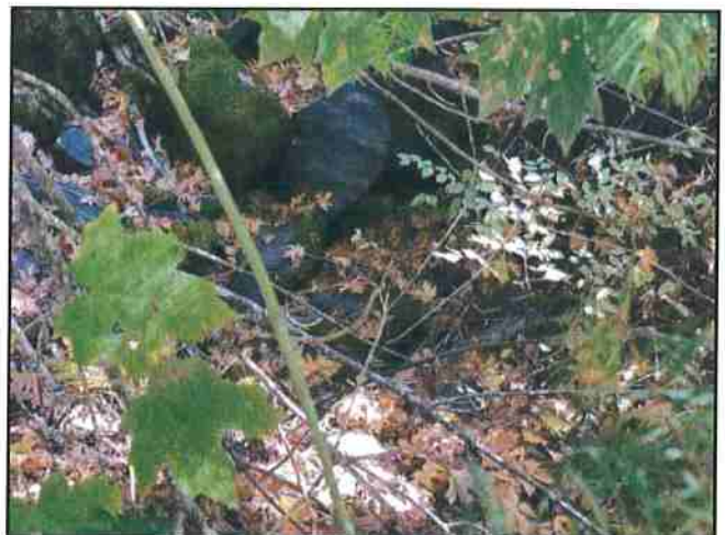
Photo #268 River Rd Looking @ Clogged Culvert In (Size Unknown)
