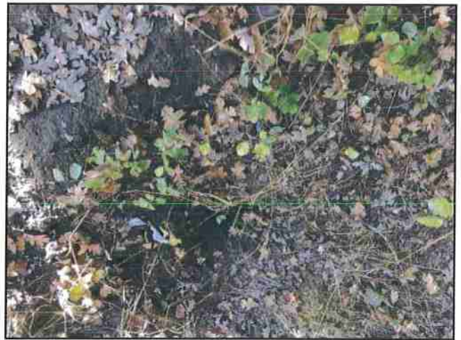
Photo #26 River Rd Looking @ Clogged 12" Culvert Out
