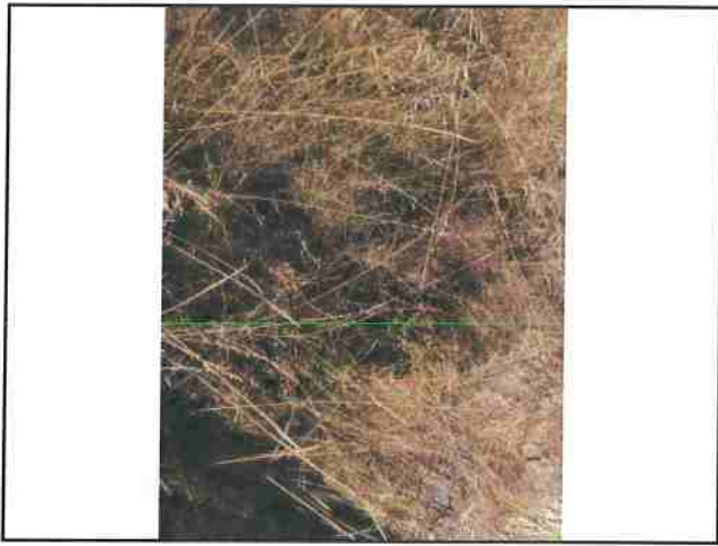
Photo #409 River Rd Looking @ Partially Clogged 24" Culvert In
