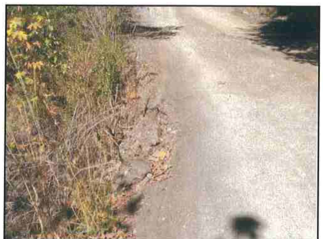
Photo #270 River Rd Looking @ Drainage & Erosion Issue
