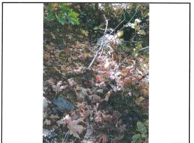
Photo #324 River Rd 24" Culvert Out
