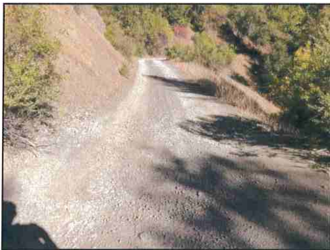
Photo #365 River Rd Looking NE @ Drainage & Erosion Issue
