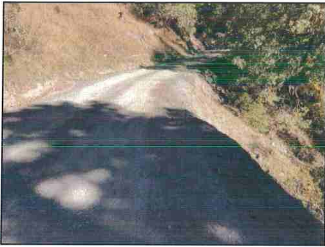
Photo #115 River Rd Looking East @ Narrowed Curve Area w/ Tire Tracks Over Eroded Area
