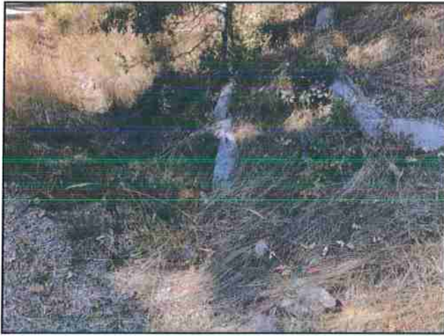
Photo #169 River Rd Looking @ Partially Clogged 24" Culvert Under Approach Running E to W
