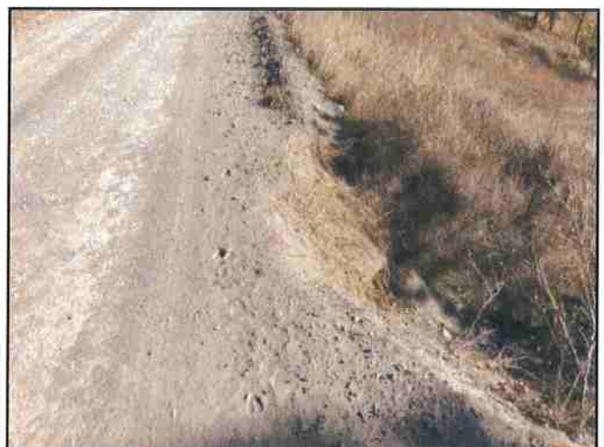
Photo #30 River Rd Looking SE @ Erosion
