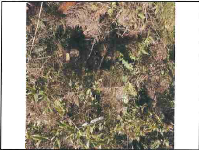
Photo #297 River Rd Looking @ Partially Clogged Out (Size Unknown)
