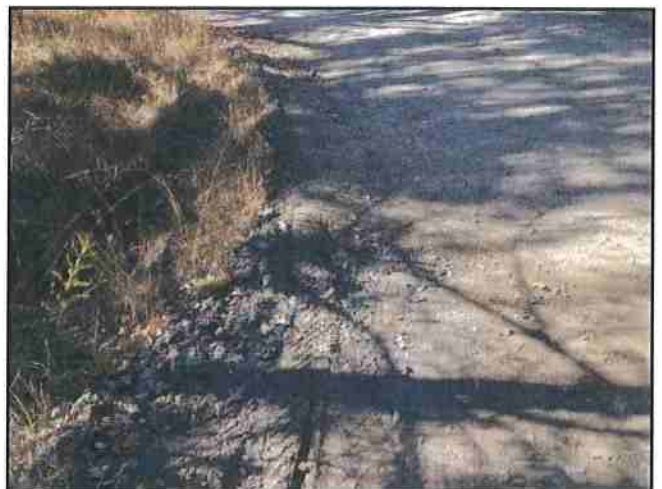
Photo #60 River Rd Looking @ Erosion and Tire Tracks through Erosion Area
