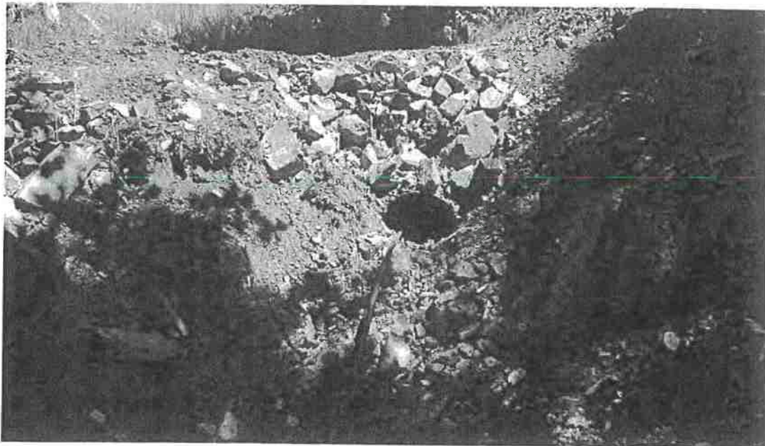
Picture 19: Outlet of SC #3. This crossing is a 24" diameter CPP located on an unnamed Class III watercourse. This culvert shall be upgraded to a minimum 42" diameter culvert per attached specifications. Photo date: 07/14/2016
