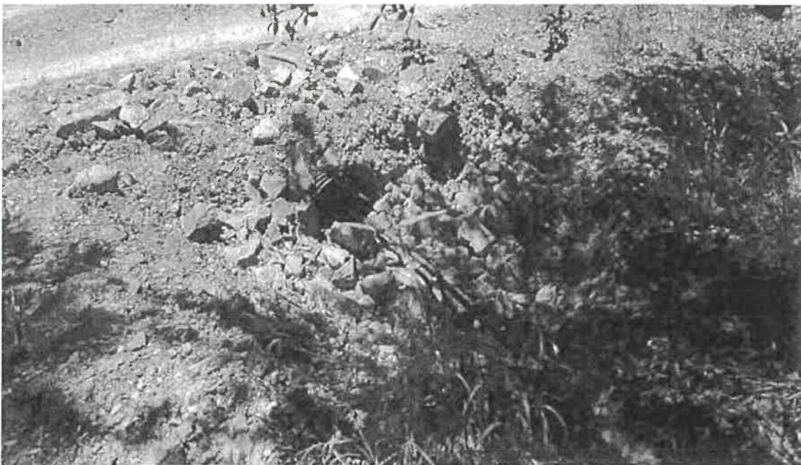
Picture 20 + 21: Inlet (top) and outlet (bottom) of SC #4. This crossing consists of a 24" diameter CPP located on an unnamed Class III watercourse. This culvert shall be upgraded to a minimum 42" diameter culvert per attached specifications. Photo date: 07/14/2016
