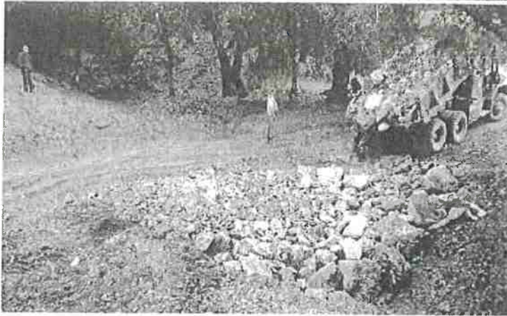
FIGURE 121D. Well graded rock armor is then backfilled into the structure and spread across the breadth of the U-shaped stream crossing, and about one-third the way up the roadbed, so that streamflow will only flow over or come in contact with resistant armor material. The armor must be spread and compacted across the design width of the expected flood flow channel width so peak flows will not flank the armored structure.
