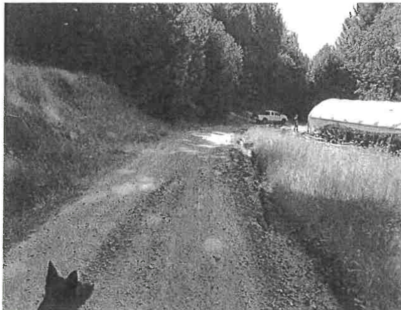
Picture 14: MP #2 is where storm runoff is concentrating along the outboard edge of the road and has eroded the road surface. The Discharger shall repair the drainage feature located behind the photographer in this picture. Photo date: 08/03/2017
