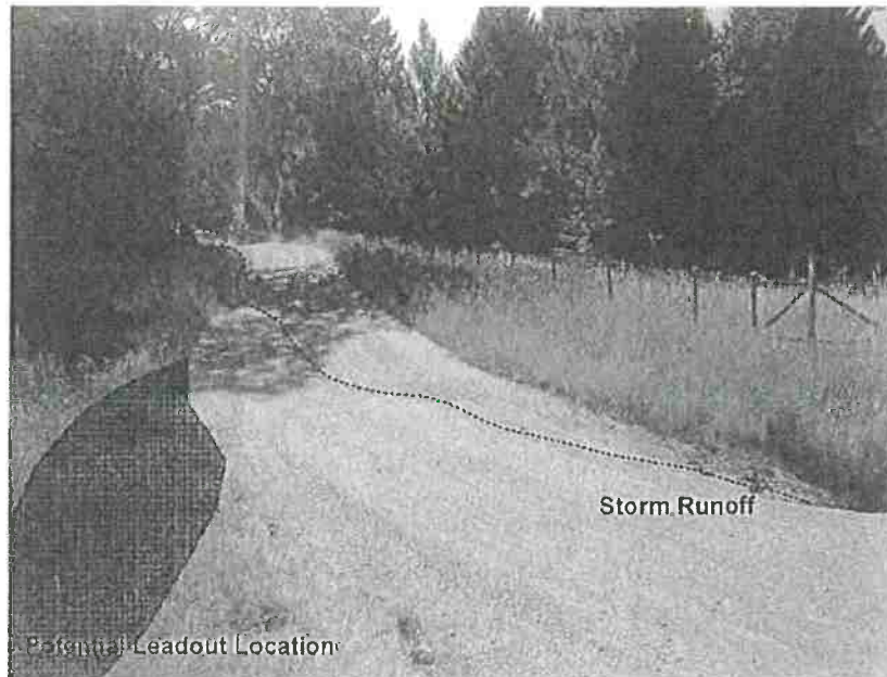
Picture 13: MP #1 is where storm runoff is concentrating along a road resulting in sediment delivery to a Class III watercourse. The Discharger shall install a drainage structure at this location. A lead out along the inboard edge of the road at this location is recommended. Photo date: 08/03/2017
