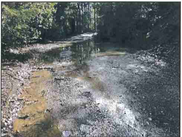
Photo #72 Kings Peak Rd @ Curve w/ Pullout Looking SE @ Drainage Issue From Clogged Culv.
