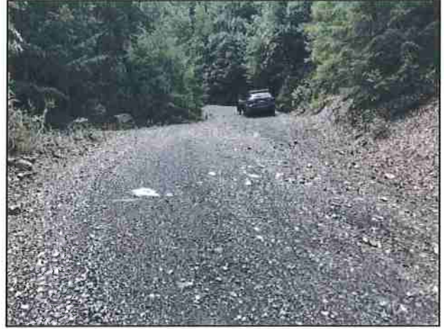
Photo #134 Kings Peak Rd @ Curve w/ Pullout Looking SW
