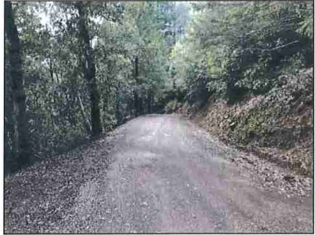
Photo #206 Kings Peak Rd @ Curve w/ Pullout Looking SW
