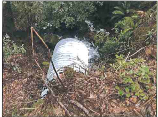
Photo #130 Kings Peak Rd Looking @ 18" Culvert Out
