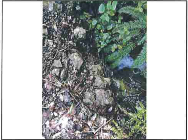
Photo #70 Kings Peak Rd Looking @ Partially Clogged 12" Culvert In
