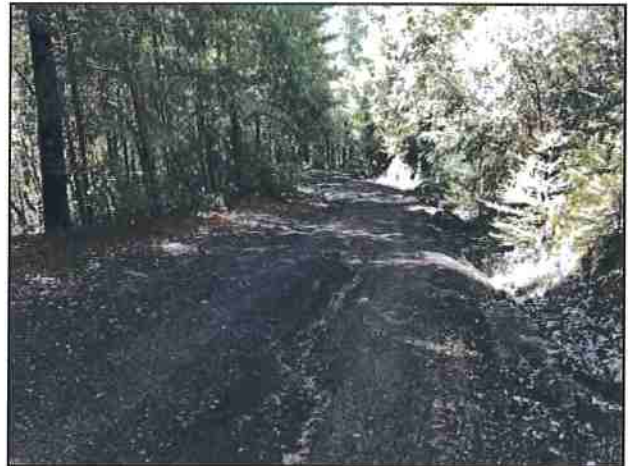
Photo #184 Kings Peak Rd @ Curve w/ Pullout Looking SW @ Drainage Issue
