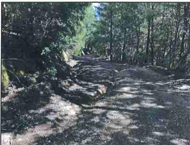
Photo #185 Kings Peak Rd @ Curve w/ Pullout Looking NE @ Drainage Issue
