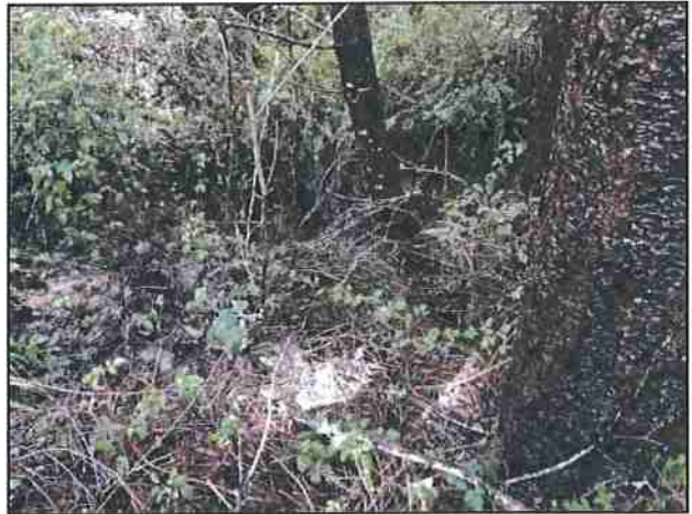
Photo #88 Kings Peak Rd Looking @ Clogged Culvert Out (Size Unknown)
