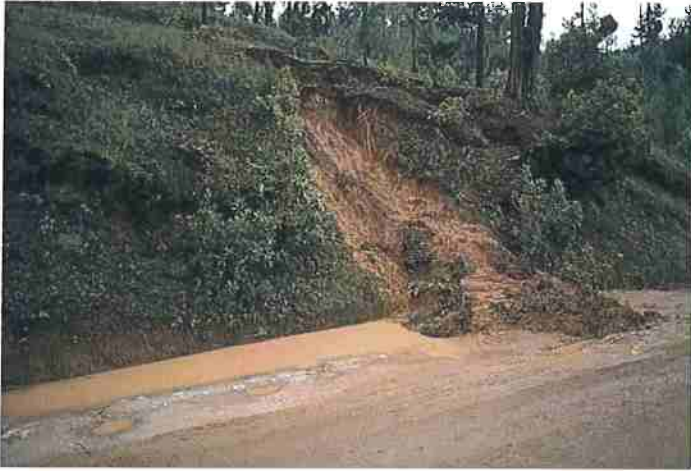
Figure 21. Cut bank failure blocking inboard ditch. Cut bank failures cause operational and maintenance problems, especially when chronic. Source: Keller and Sherar 2003.
