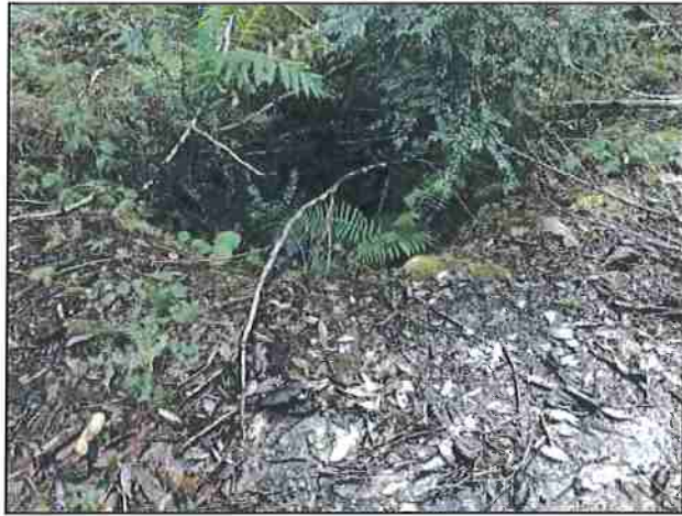
Photo #121 Kings Peak Rd Looking @ Clogged Culvert Out (Size Unknown)
