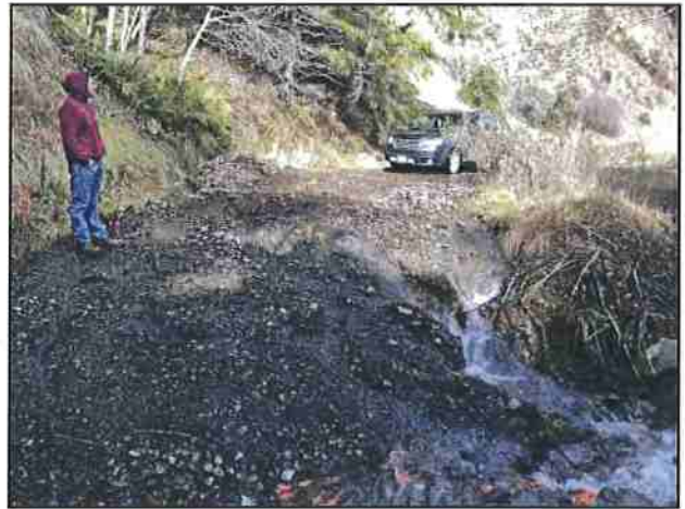
Photo #172 Kings Peak Rd @ Curve w/ Pullout Looking NE (Culvert Needed)
