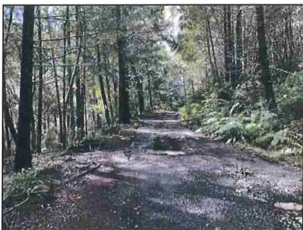
Photo #119 Kings Peak Rd @ Pullout Looking SW @ Drainage Issue
