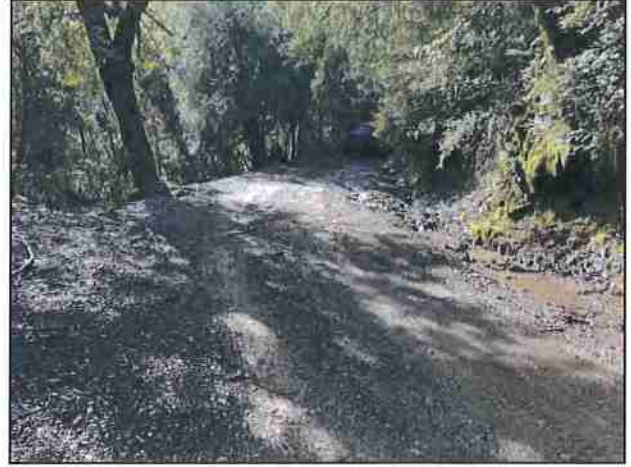
Photo #74 Kings Peak Rd @ Curve w/ Pullout Looking SW @ Drainage Issue
