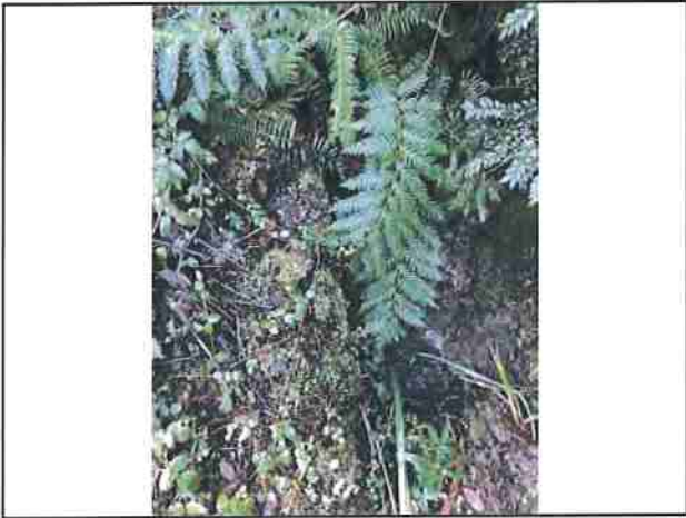
Photo #87 Kings Peak Rd Looking @ Clogged Culvert In (Size Unknown)
