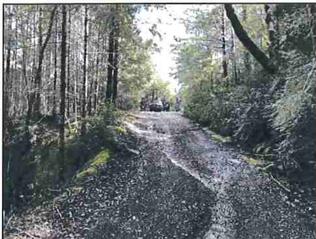
Photo #59 Kings Peak Rd @ Curve w/ Pullout Looking SE @ Drainage Issue
