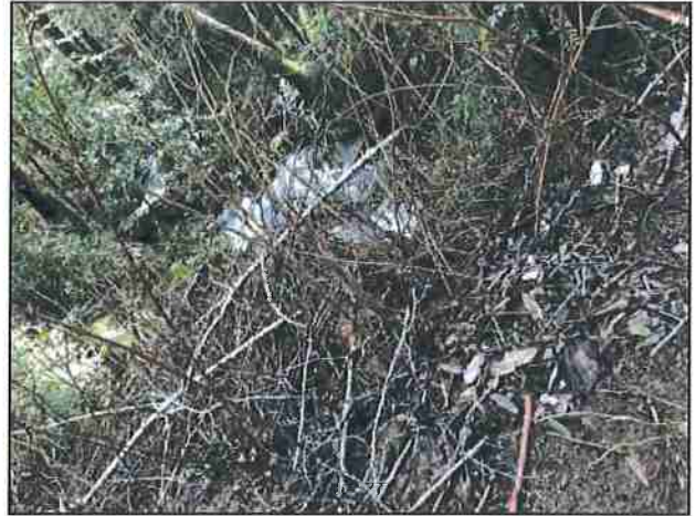
Photo #128 Kings Peak Rd Looking @ 18" Culvert Out
