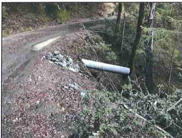
Photo #161 Kings Peak Rd 18" Culvert Out
