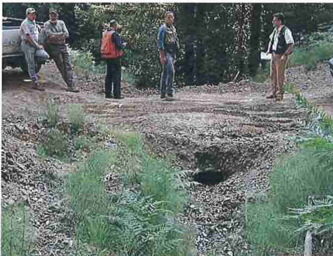
Figure 16. Culvert plugged with sediment at inlet. Photo: Angela Wilson, Central Valley Regional Water Quality Control Board.
