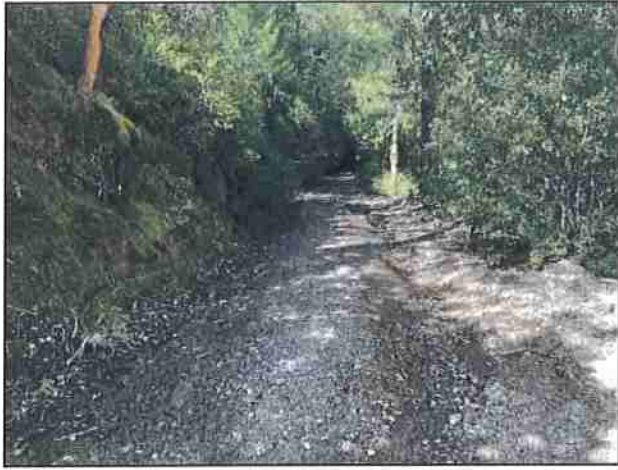
Photo #49 Kings Peak Rd @ Curve w/ Pullout Looking NW @ Rutting Caused By No Water Bars
