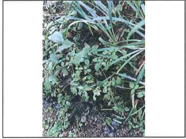
Photo #104 Kings Peak Rd Looking @ Clogged Culvert In (Size Unknown)
