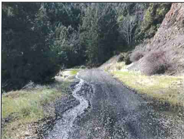
Photo #167 Kings Peak Rd Looking SW @ Curve w/ Pullout & Drainage Issue
