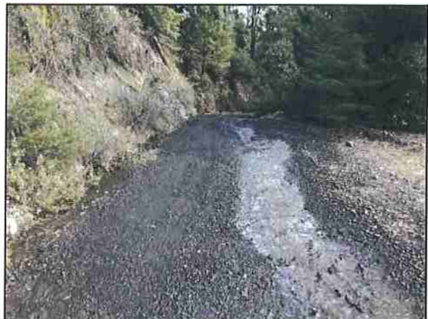
Photo #166 Kings Peak Rd Looking NE @ Curve w/ Pullout & Drainage Issue
