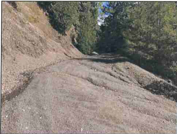
Photo #177 Kings Peak Rd @ Curve w/ Pullout Looking NE @ Drainage Issue
