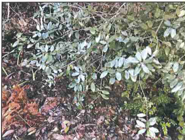
Photo #71 Kings Peak Rd Looking @ Clogged 12" Culvert Out
