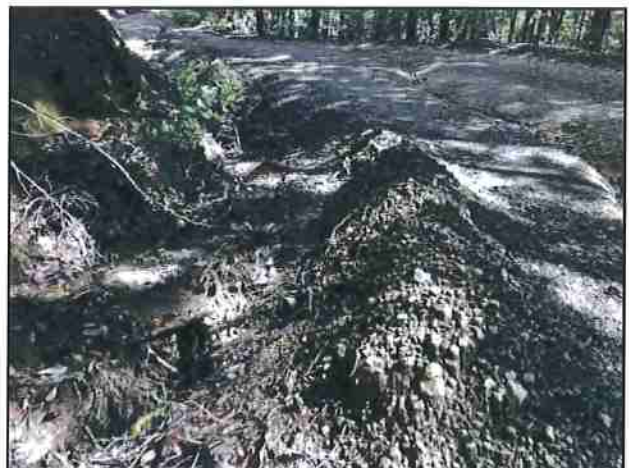
Photo #186 Kings Peak Rd Looking at Clogged 18" Culvert In & Dirt Pile Causing Drainage Issue
