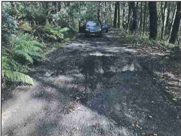
Photo #123 Kings Peak Rd @ Curve w/ Pullout Looking NE Looking @ Drainage Issue
