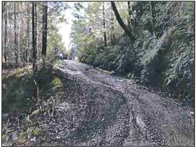
Photo #58 Kings Peak Rd @ Curve w/ Pullout Looking SE @ Drainage Issue
