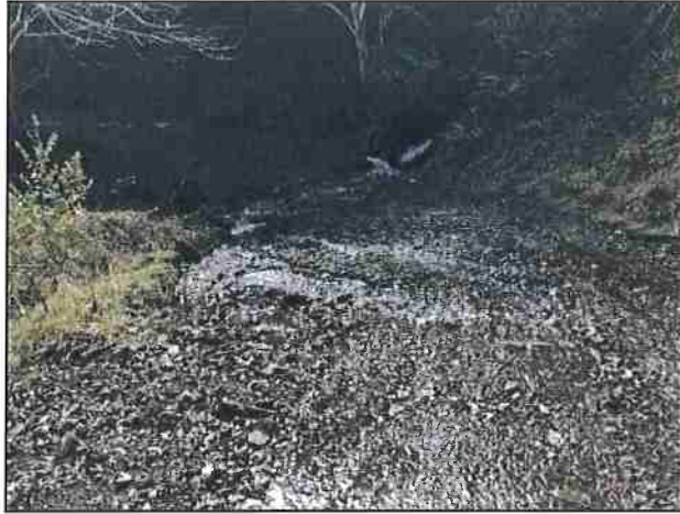
Photo #169 Kings Peak Rd @ Curve w/ Pullout Looking SW (Culvert Needed)
