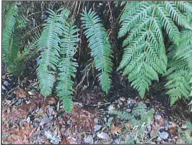
Photo #193 Kings Peak Rd Looking @ Clogged Culvert In (Size Unknown, Out Not Located)
