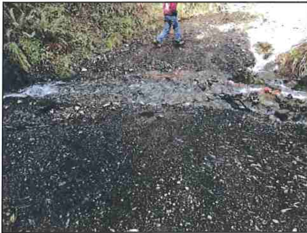
Photo #171 Kings Peak Rd @ Curve w/ Pullout Looking NE (Culvert Needed)
