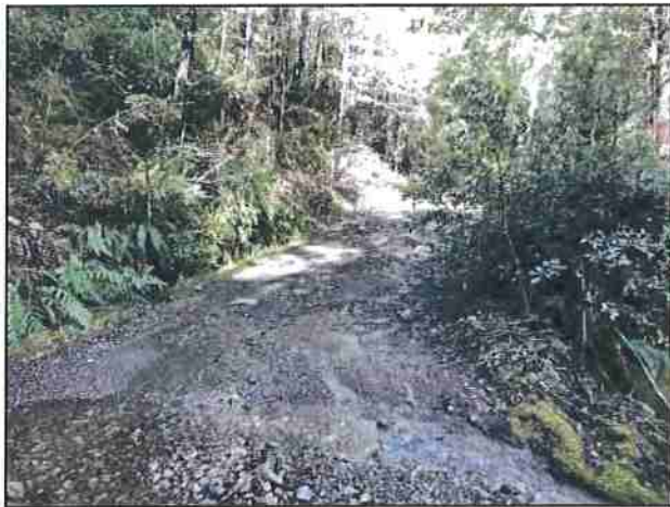
Photo #57 Kings Peak Rd @ Curve w/ Pullout Looking NE @ Drainage Issue
