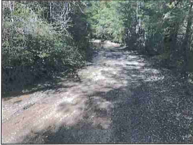
Photo #73 Kings Peak Rd @ Curve w/ Pullout Looking NE @ Drainage Issue
