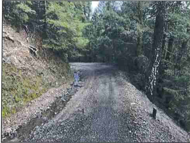
Photo #163 Kings Peak Rd Looking NE @ Curve w/ Pullout & Drainage Issue
