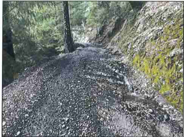
Photo #164 Kings Peak Rd Looking SW @ Drainage Issue
