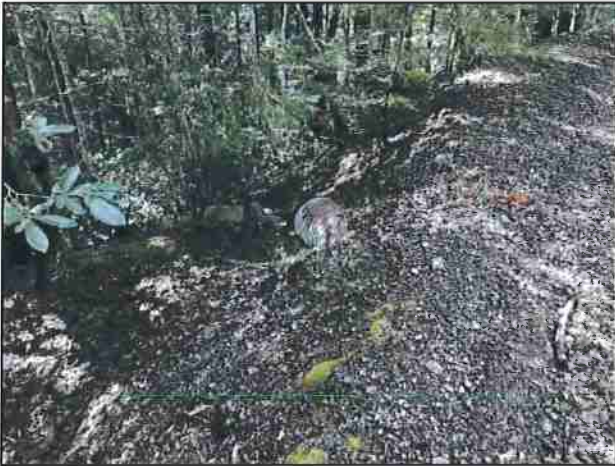
Photo #189 Kings Peak Rd Looking @ 18" Culvert Out
