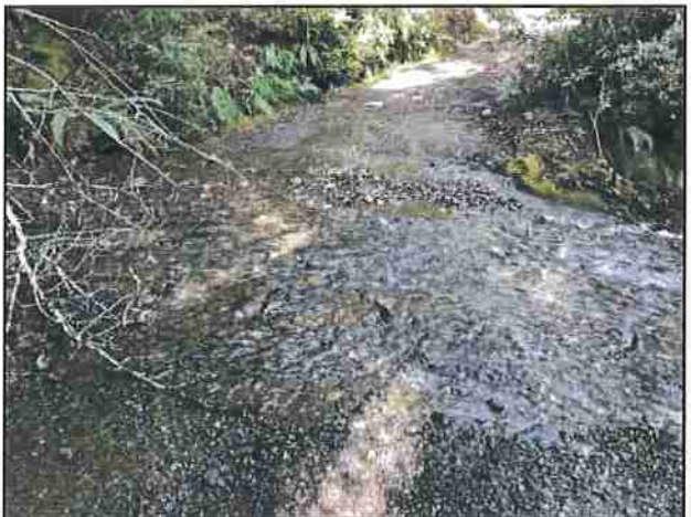
Photo #60 Kings Peak Rd @ Curve w/ Pullout Looking @ Stream Crossing Rd Needs Culvert
