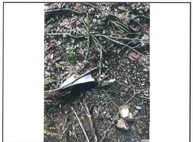
Photo #162 Kings Peak Rd Clogged 18" Culvert In
