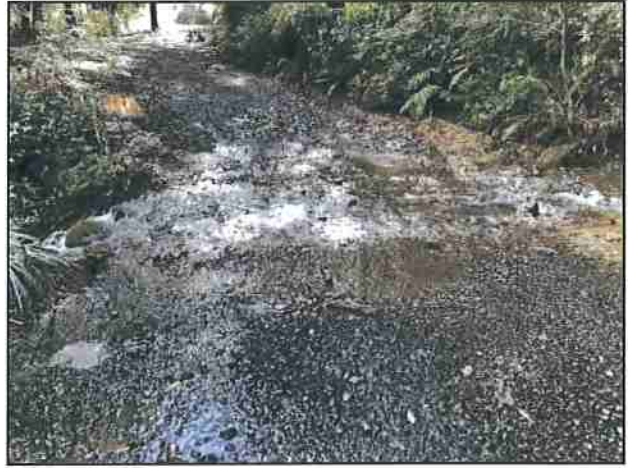
Photo #106 Kings Peak Rd @ Curve w/ Pullout Looking SE @ Drainage Issue from Culvert
