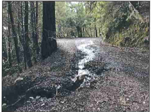
Photo #160 Kings Peak Rd @ Drainage Issue Caused by Clogged Culvert (162) Looking NE
