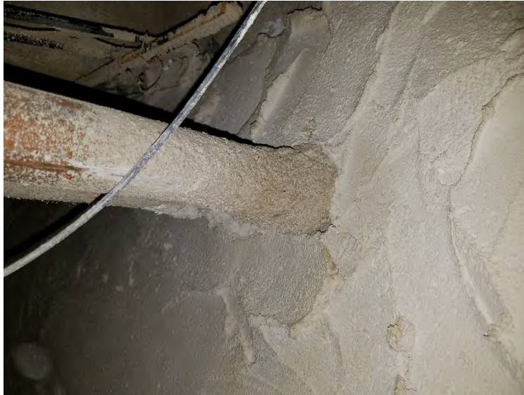
Above ceiling in Rm. 229 & RR 230, ACM spray on fireproofing on pipe at wall penetration
