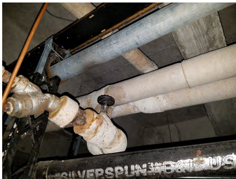
Above ceiling in Rm. 229 & RR 230, ACM pipe insulation on pipe elbows & tees
