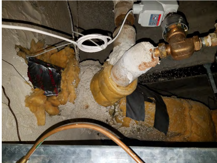
Above ceiling in Rm. 229 & RR 230, ACM pipe insulation on pipe elbows & tees, and ACM spray on fireproofing as overspray on fiberglass duct insulation
