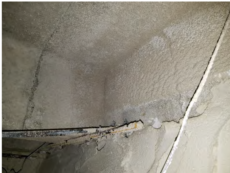
Above ceiling in Rm. 229 & RR 230, ACM spray on fireproofing on concrete ceiling & beams
