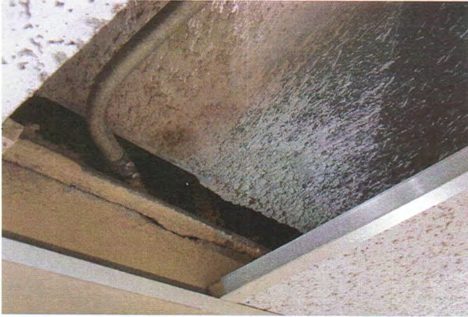
Top—Over-spray of ACM insulation above drop ceiling, 1st floor, east side of west corridor.1
