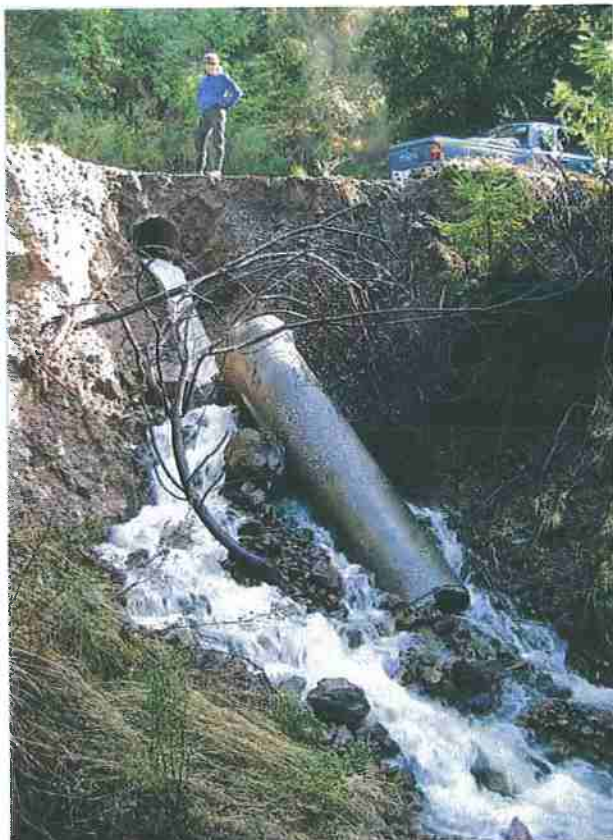
Figure 34. Outlet of a concrete culvert (30 inches in diameter) before the project. The culvert was placed too high in the fill, resulting in a 10-foot drop to the channel at the outlet. This caused erosion of the road fill and stream banks, eventually undermining the outer section of the culvert. Photo: Jared Gerstein.
