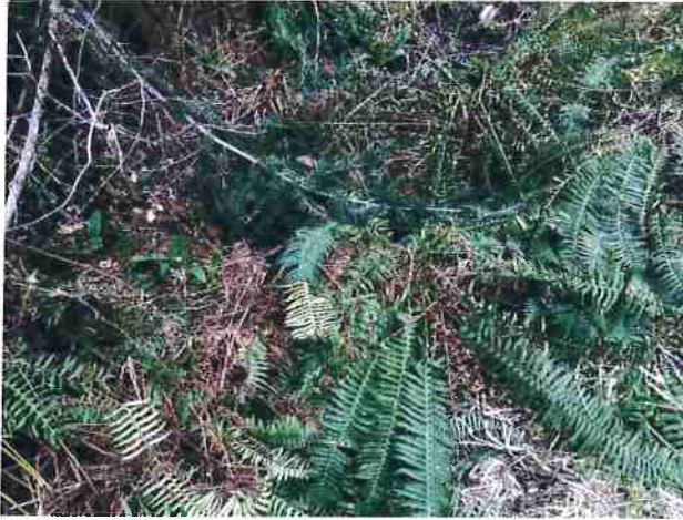
Photo #123 @ Unnamed Rd Looking @ 12" Clogged Culvert In
