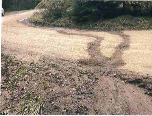
Photo #151 @ Unnamed Rd Looking @ Drainage & Erosion
