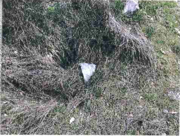
Photo #188 Unnamed Rd @ Crushed 12" Culvert In
