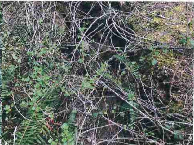
Photo #124 @ Unnamed Rd Looking @ 12" Clogged Culvert Out
