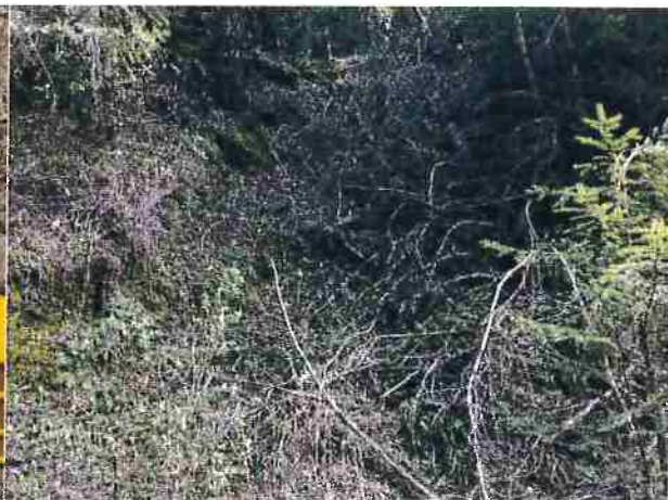
Photo #96 @ Unnamed Rd @ Clogged Culvert
