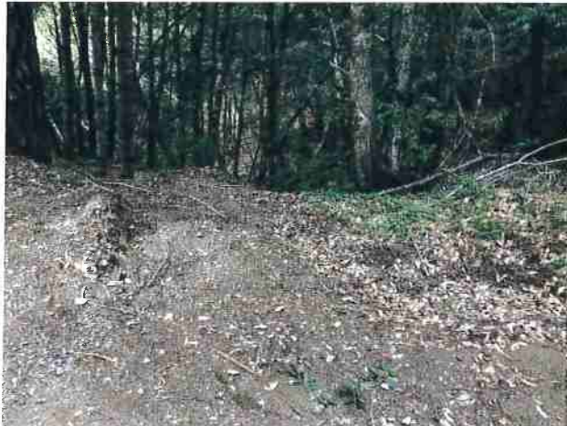
Photo #105 @ Unnamed Rd Looking @ Road Erosion
