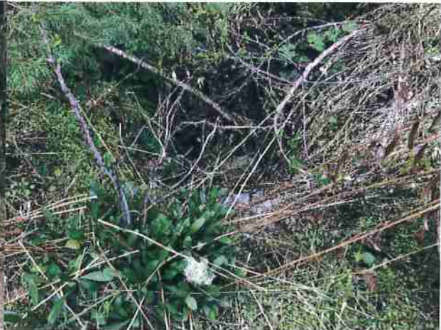
Photo #218 Unnamed Rd Looking @ Clogged 12" Culvert In
