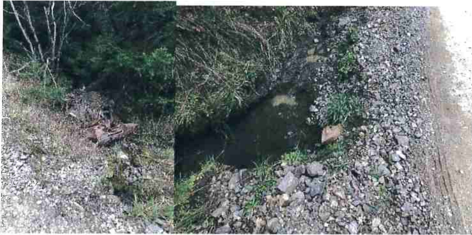
Photo #199 Looking @ Crushed Car In SMA Photo #200 Crushed Culvert
