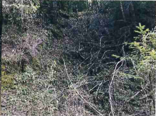
Photo #100 @ Unnamed Rd Looking @ Clogged Culvert
