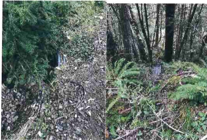
Photo #163 @ Unnamed Rd Looking @ 12" Culvert In Photo #164 @ Unnamed Rd Looking @12" Culvert In
