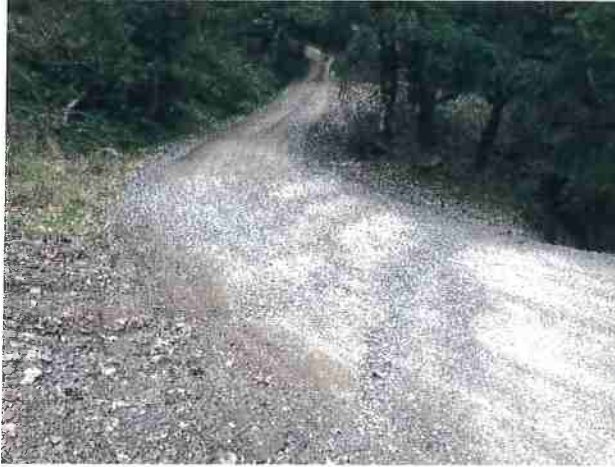
Photo #211 Unnamed Rd Looking South (Erosion - No Culvert)
