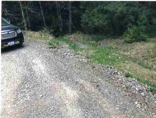
Photo #179 Unnamed Rd Looking West @ Drainage & Erosion
