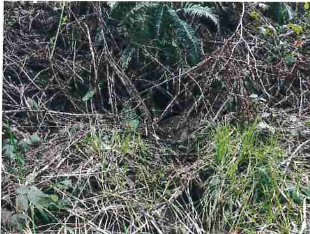
Photo #125 @ Unnamed Rd Looking @ 12" Clogged Culvert Out
