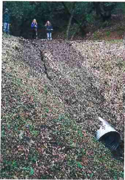
Figure 41. Fill surface erosion occurring after a road upgrading project. Photo: Bill Weaver, Pacific Watershed Associates.
