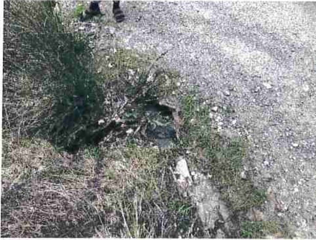
Photo #187 Unnamed Rd @ Crushed 12" Culvert Out
