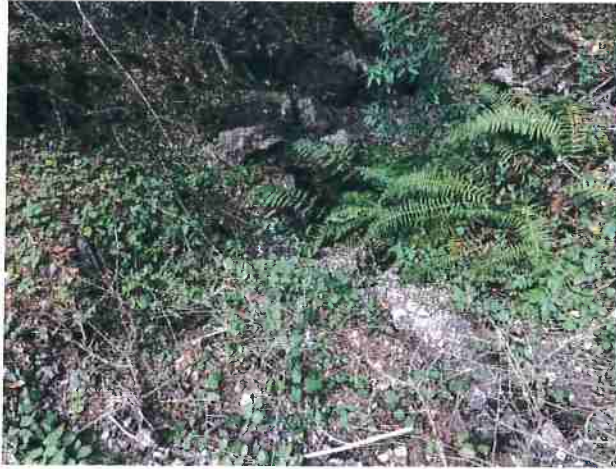
Photo #97 @ Unnamed Rd Looking @ Clogged Culvert
