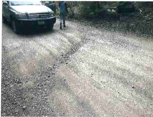
Photo #157 @ Unnamed Rd Looking @ Drainage & Erosion
