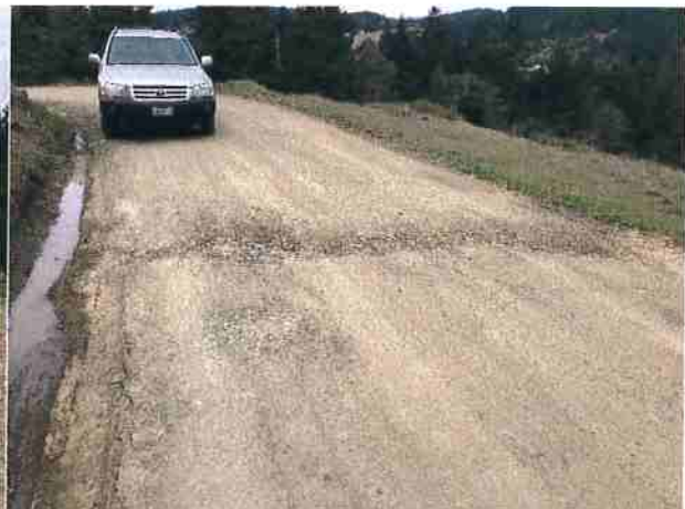
Photo #132 @ Unnamed Rd Looking North @ Drainage & Erosion
