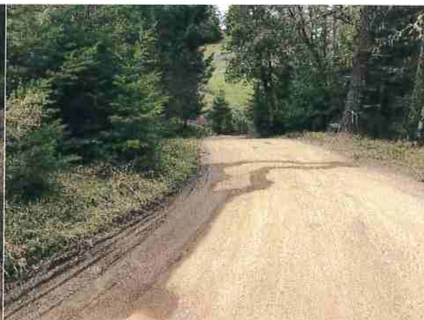
Photo #150 @ Unnamed Rd Looking North @ Drainage & Erosion
