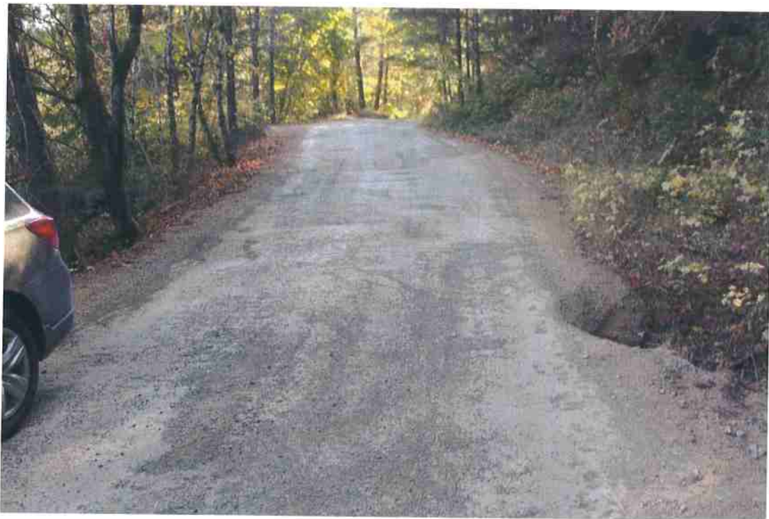
Photo 2. Mile 0.2: 16-ft road width with no shoulder at culvert crossing. The road could be widened at the culvert but there is decent visibility at the site so widening is not necessary.
