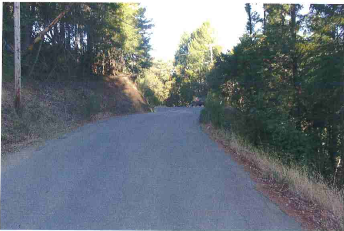
Photo 28. Mile 2.4: 16-ft road width with 1-ft shoulders at blind corner. Potential spot to widen corner on the inside to improve width and visibility.
