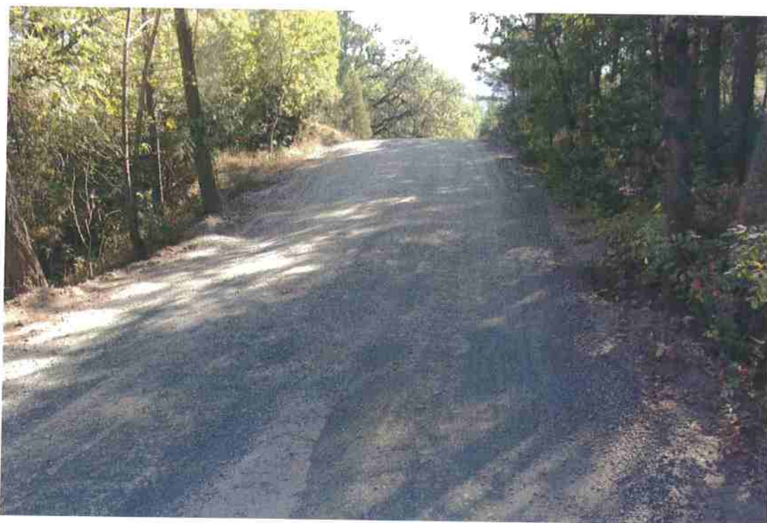
Photo 8. Mile 0.55: Pinch point at culvert; 16-ft road width with no shoulder. The road could be widened at the culvert location but there is decent visibility.
