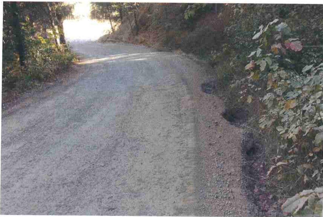
Photo 4. Mile 0.35: Inboard ditch eroding into road.
