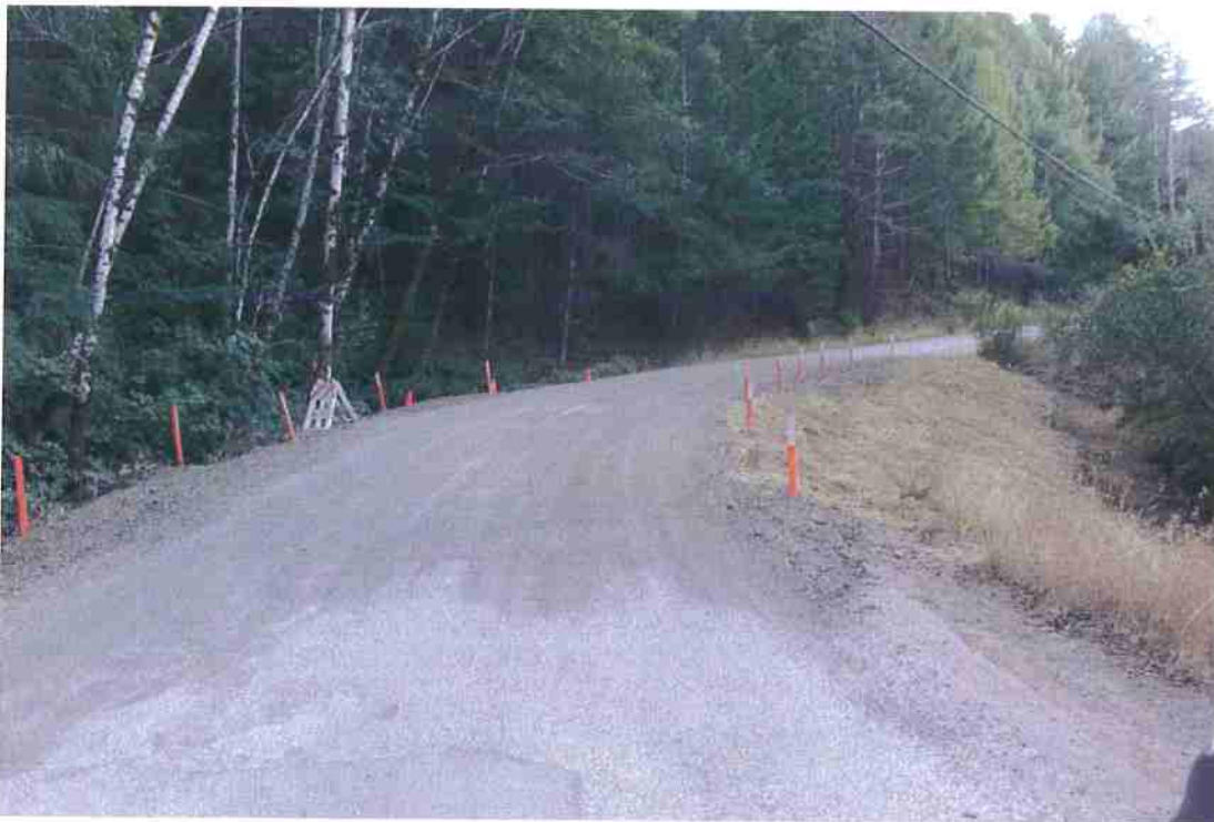
Photo 30. Mile 12.6: Recent culver repair, short gravel segment. 18-ft road width with 2-ft shoulders.
