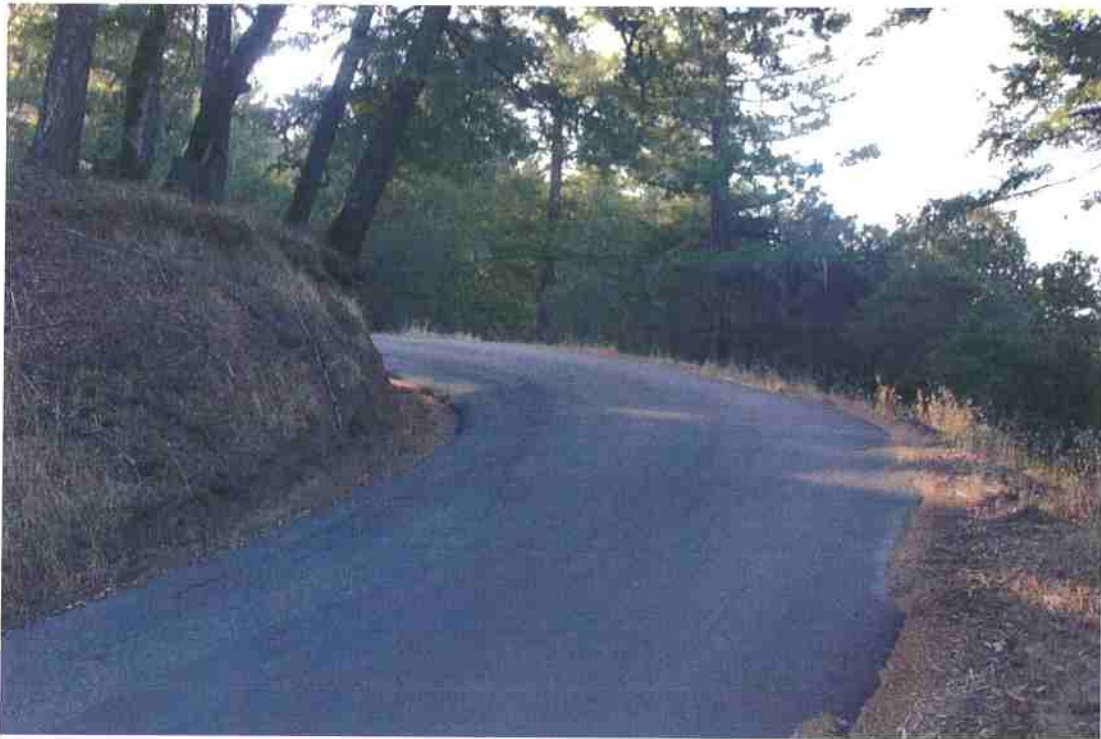
Photo 36. Mile 3.15: Dangerous pinch point at blind corner. 15-ft road width with 1-ft shoulders. Potential spot to widen corner on inside to improve width and visibility.
