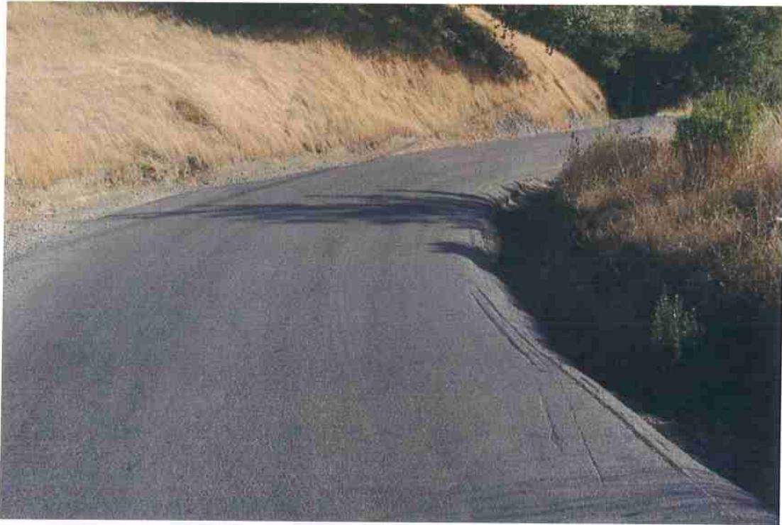
Photo 43. Mile 3.7: 12-ft road width with 1-ft shoulder. Partially blind corner with deep ditch. Potential spot to widen corner on inside to improve width and visibility.
