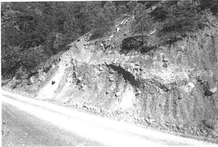
Figure 5: View southeasterly across haul road at road cut exposing colluvium developed over deeply weathered serpentinite. Note layers of dominantly serpentinite (gray) mixed with layers of dominantly other rock types (iron oxide stained).
