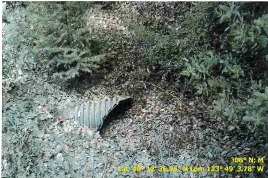
Figure 12. Photograph showing Road Point 42 which is 18" drainage relief culvert with debris in the inlet that needs to be cleared.
