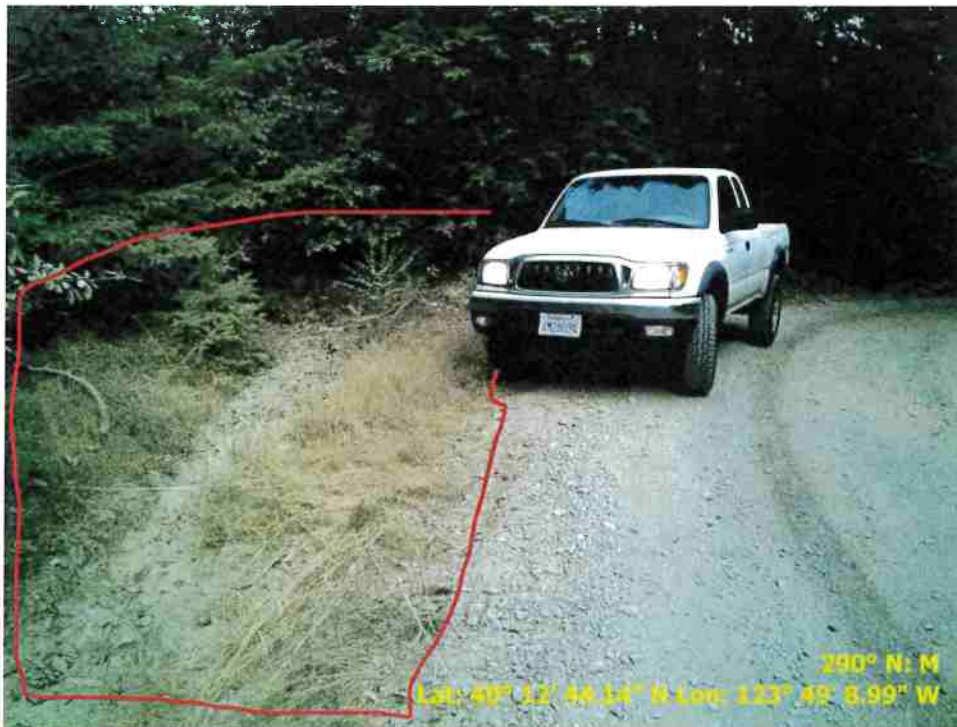
Figure 10. Photograph showing Road Point 31 which is a pullout that need to be regraded.
