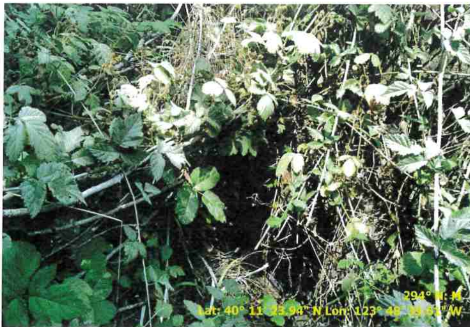
Figure 35. Photo of Road Point 115 showing the inlet of a 36" onstream culvert that needs the inlet cleared.
