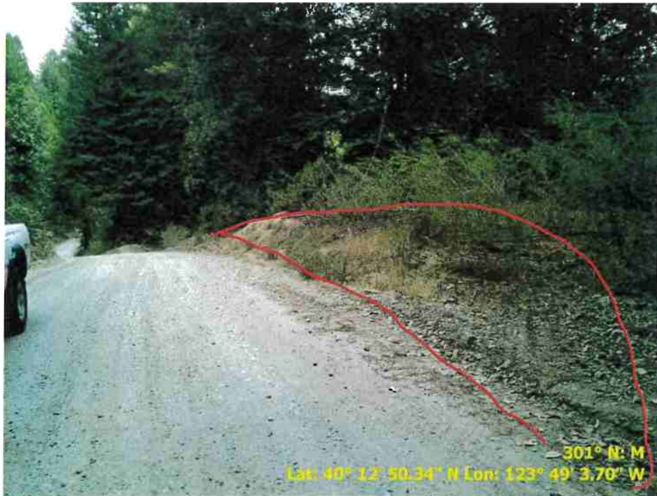
Figure 8. Photograph showing Road Point 16 which is a pullout that need to be regraded.
