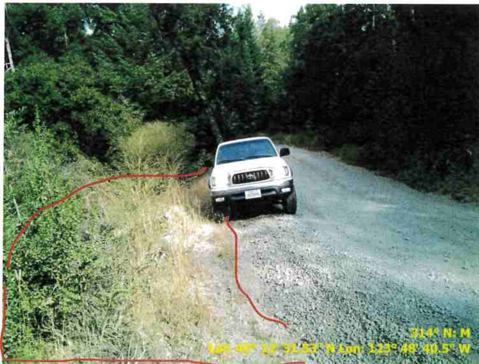
Figure 14. Photo of Road Point 67 showing a pullout that needs to be regraded and vegetation cleared.
