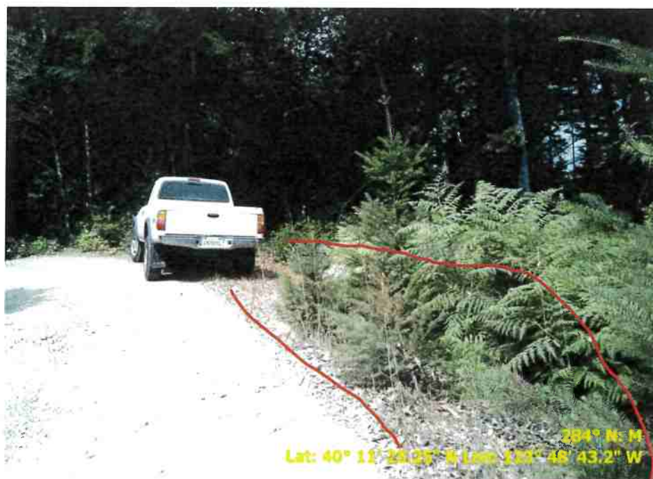
Figure 36. Photo of Road Point 118 showing a pullout that needs to be cleared of vegetation and regrading.
