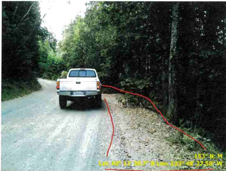
Figure 18. Photo of Road Point 77 showing a pullout that needs to have a stump cleared and regraded.
