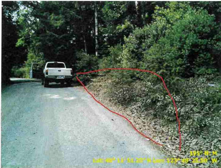
Figure 24. Photo of Road Point 89 showing a pullout that needs to be regraded and vegetation cleared.
