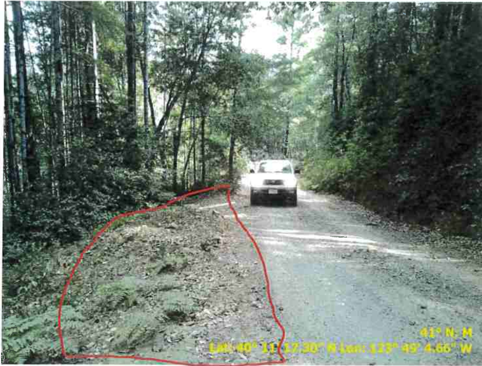
Figure 39. Photo of Road Point 127 showing a pullout that needs to be cleared of vegetation and regrading.
