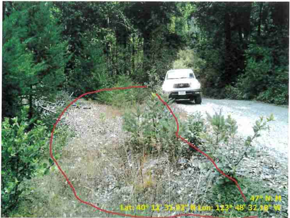
Figure 33.. Photo of Road Point 110 showing a pullout that needs to be cleared of vegetation and regrading.
