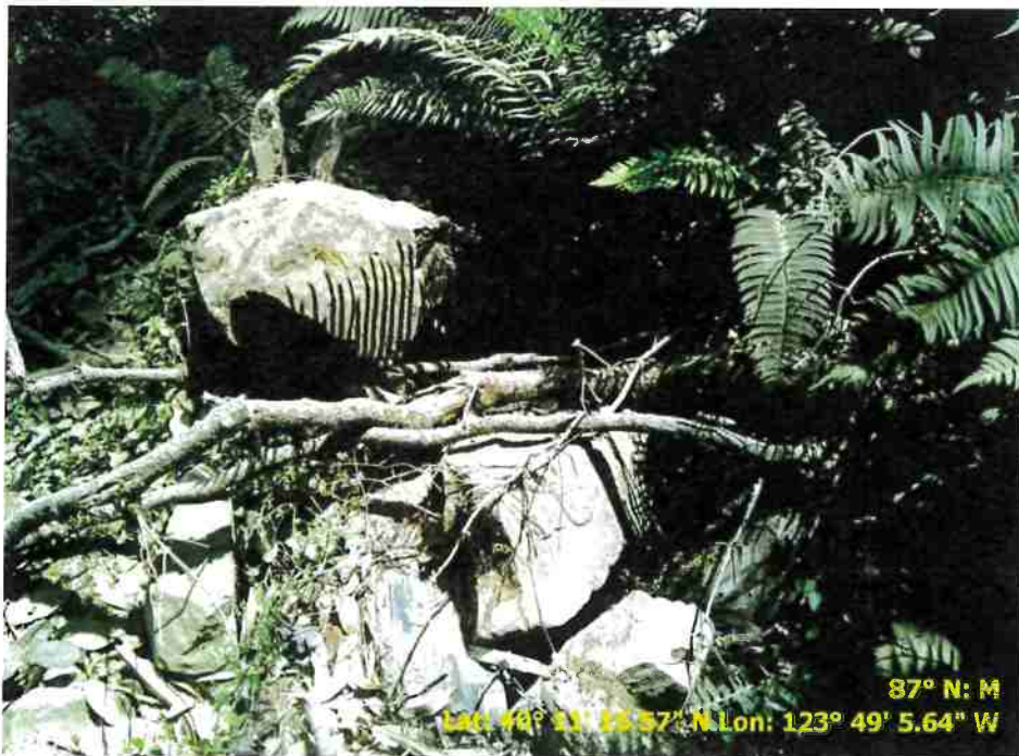
Figure 40. Photo of Road Point 132 showing the inlet of a 18" onstream culvert that needs the inlet cleared.
