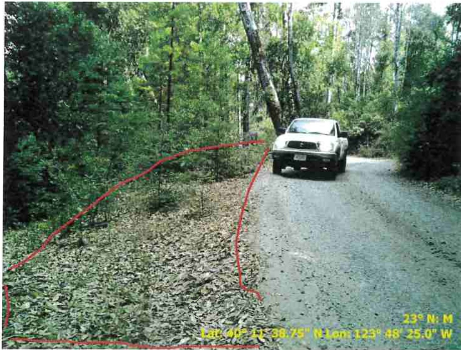
Figure 31. Photo of Road Point 104 showing a pullout that needs to be cleared of vegetation and regrading.
