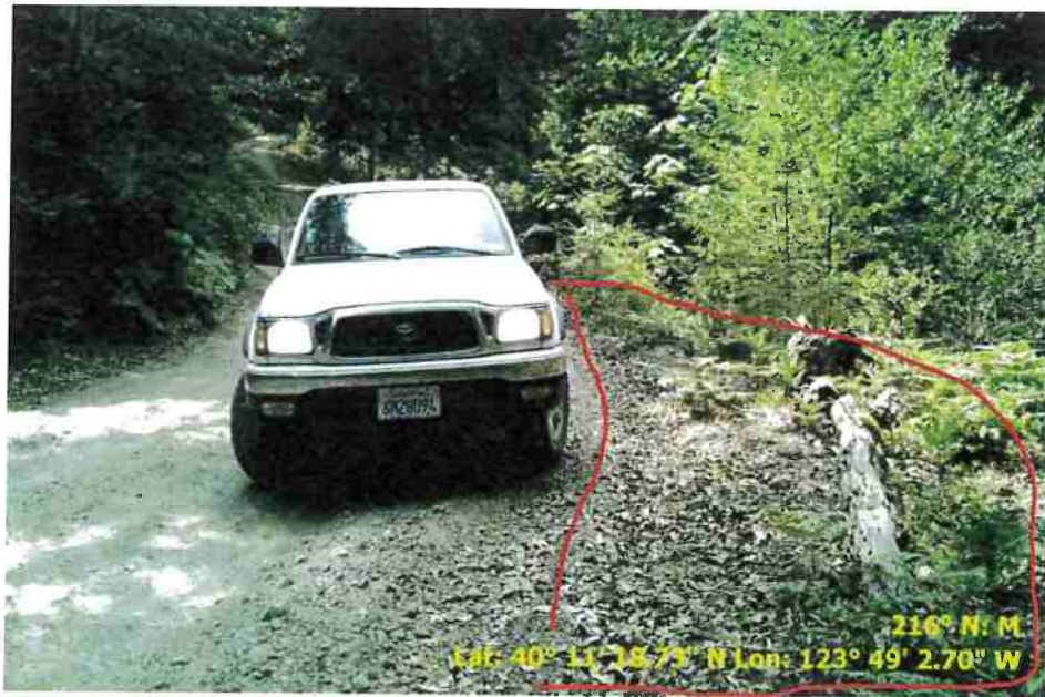
Figure 49. Photo of Road Point 162 showing a pullout that needs to be cleared of vegetation and regraded.
