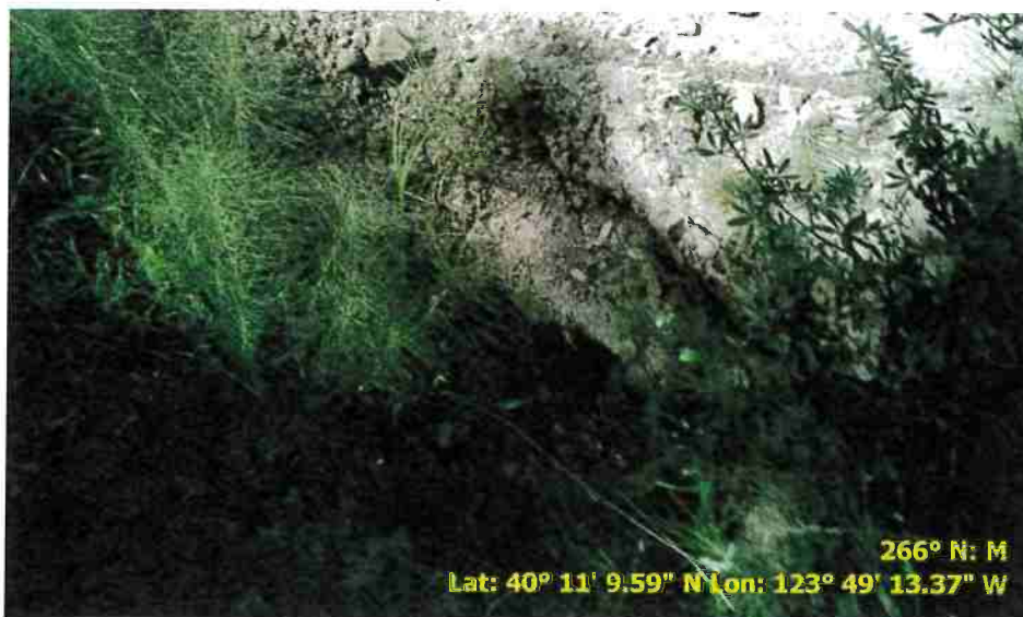
Figure 46. Photo of Road Point 148 showing the inlet of an 18" onstream culvert that needs the inlet cleared and the inlet needs rock slope protection above and around the inlet.
