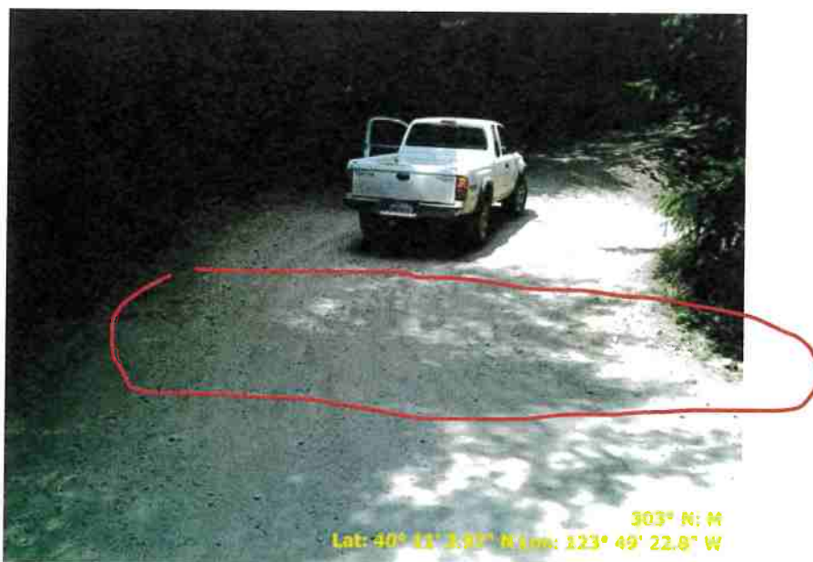
Figure 48. Photo of Road Point 159 showing a class three stream crossing that need a culvert or rock ford.
