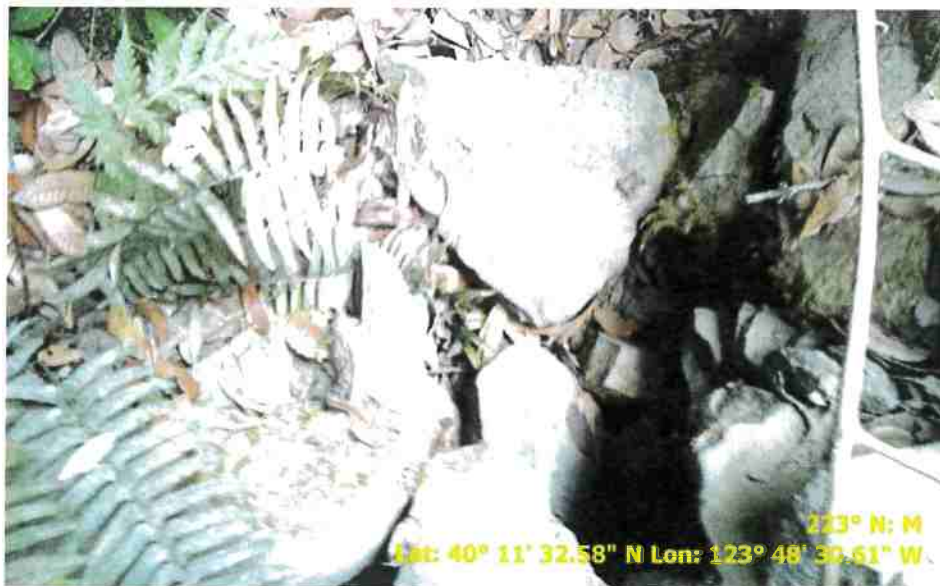
Figure 32. Photo of Road Point 190 showing the inlet of and 18" drainage relief culvert that needs to be cleared.
