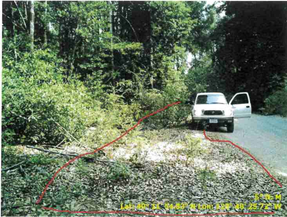
Figure 23. Photo of Road Point 80 showing a pullout that needs to be regraded and vegetation cleared.
