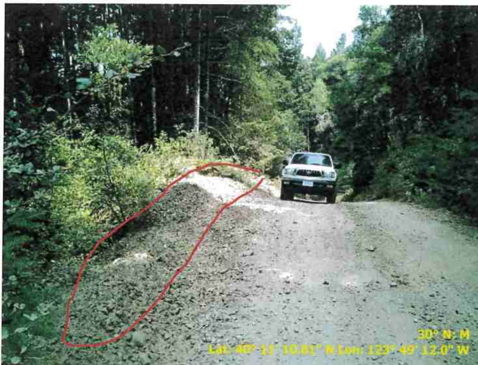
Figure 45. Photo of Road Point 145 showing a pullout that needs to be cleared of vegetation and regraded.
