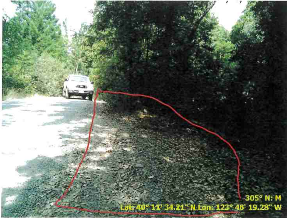
Figure 29. Photo showing a pullout that needs vegetation cleared and regrading.
