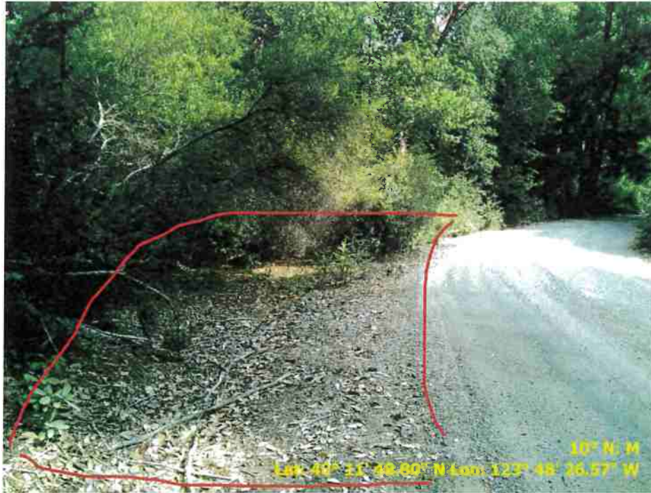
Figure 25. Photo of Road Point 91 showing a pullout that needs vegetation cleared and to be regraded.
