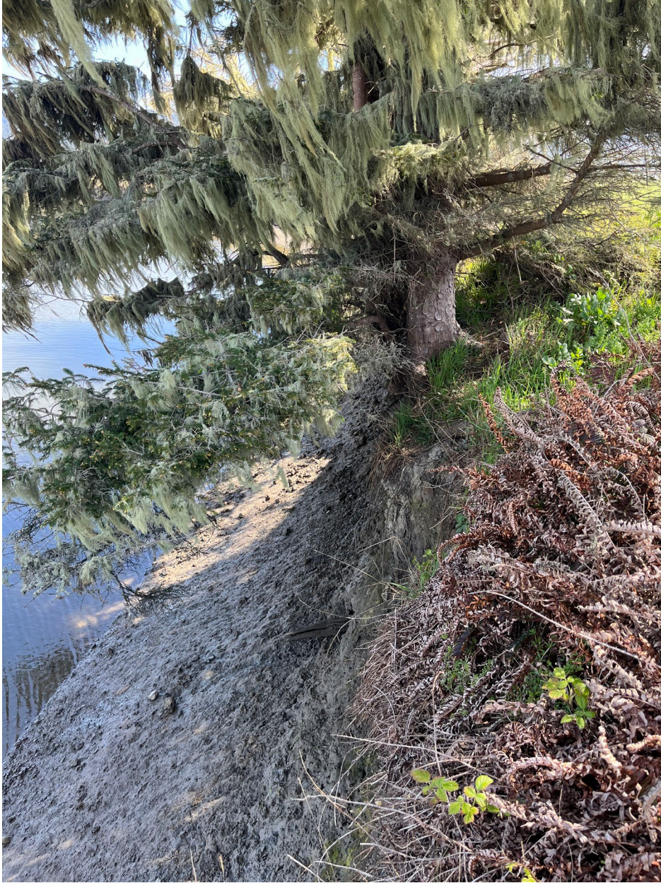
Photo 1. Example for project site conditions. All the trees, except one, are growing along the levee edge at the top of the slough bank.
