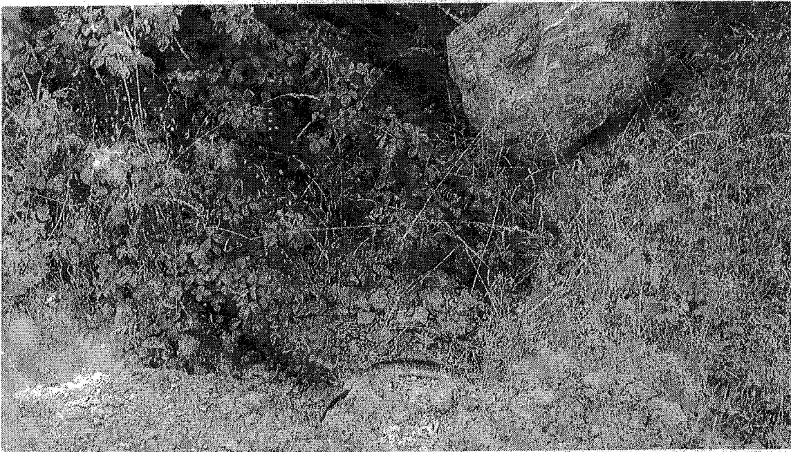
Site 02 – Class III watercourse crossing consisting of an 18” culvert. View of the inlet.
