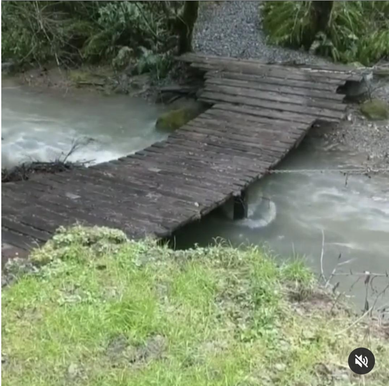
Figure 3. Bridge we are requesting to repair in it's current state, pictured here with the creek at it's highest flow. Fish and game has said that it's current height is not enough to allow down wood to pass through at high tides
