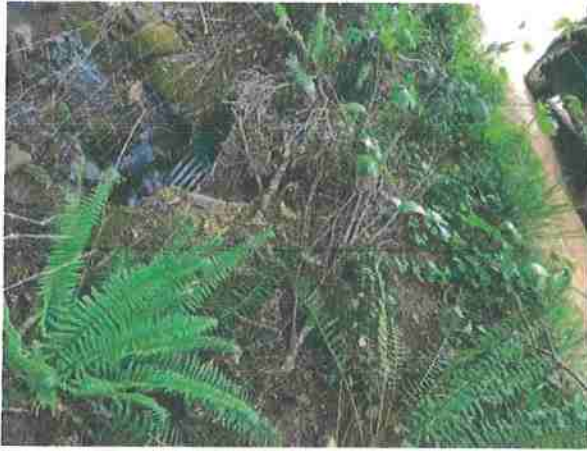
Photo #170, location 43 west 18" cmp inlet.
