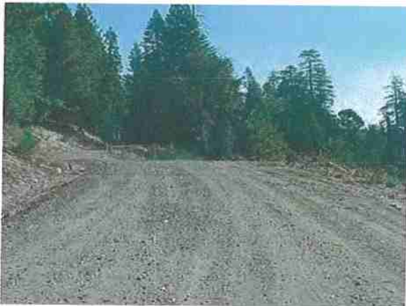
Figure 38. Pinchard Creek road immediately after project construction, 2002. Photo: Joe Hoffman, Plumas National Forest.
