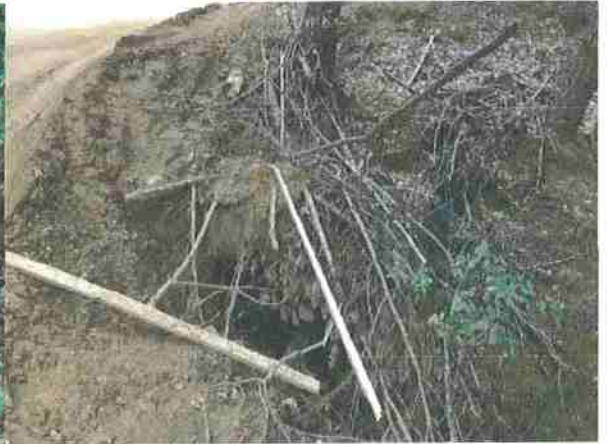
Photo #133, location 34 east side of road 18" cmp outlet.
