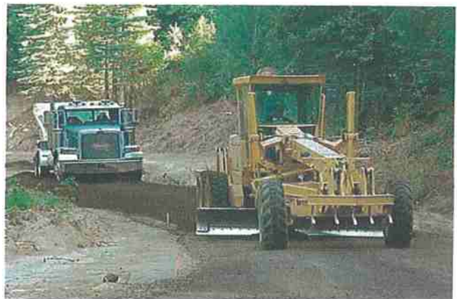
Figure 33. A grader spreading the gravel on the road surface placed by a dump truck. Source: Joe Hoffman, Plumas National Forest.
