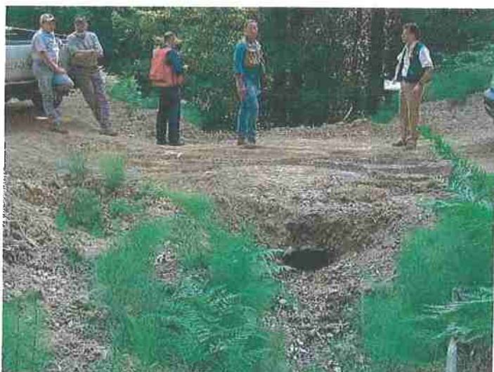
Figure 16. Culvert plugged with sediment at inlet. Photo: Angela Wilson, Central Valley Regional Water Quality Control Board.
