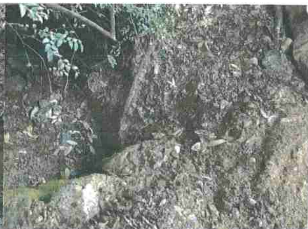
Photo #175, location 44 south 18" cmp outlet
