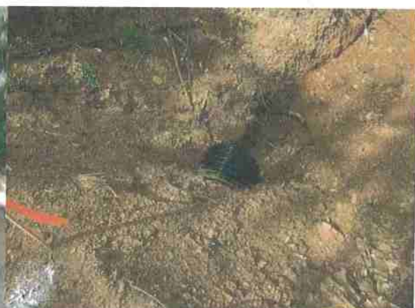
Photo #145, location 37 south side road 18" cpp outlet.
