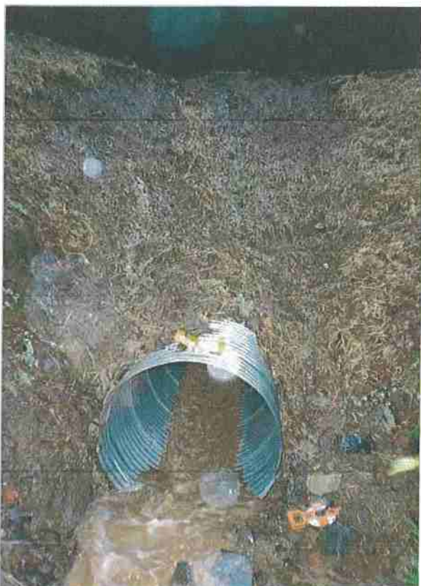
Figure 2. This cross drain delivers sediment from the roadside ditch under the road surface to a nearby stream. The road fill is also eroding. Photo: Jared Gerstein.
