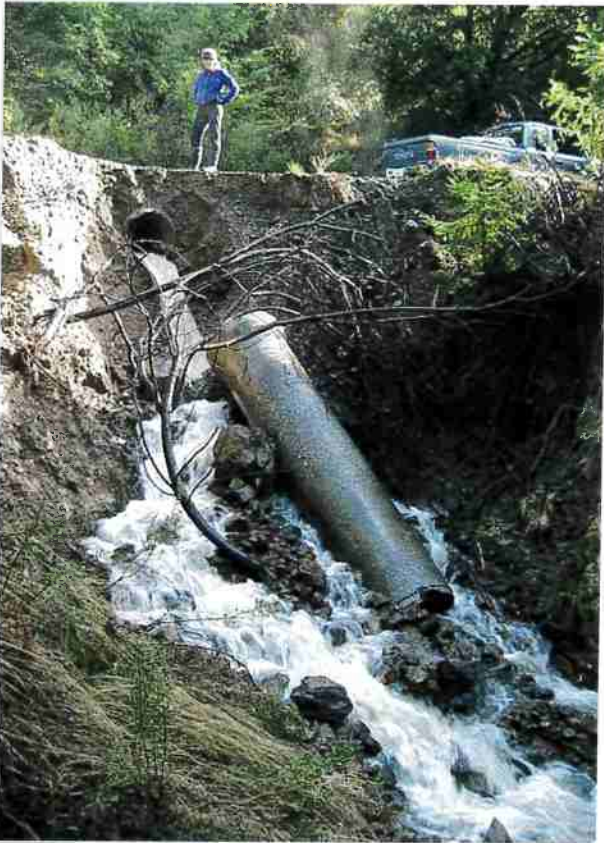
Figure 34. Outlet of a concrete culvert (30 inches in diameter) before the project. The culvert was placed too high in the fill, resulting in a 10-foot drop to the channel at the outlet. This caused erosion of the road fill and stream banks, eventually undermining the outer section of the culvert. Photo: Jared Gerstein.
