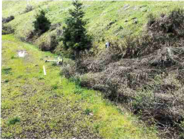
Photo #27 Access Road 12" Culvert Clogged Inlet
