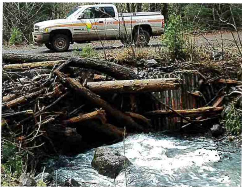
Figure 23. This culvert is nearly plugged by woody debris, endangering the road. Photo: Angela Wilson, Central Valley Regional Water Quality Control Board.
