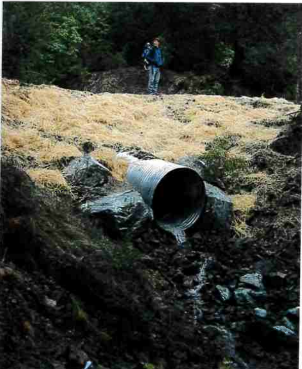
Figure 35. The culvert was replaced with a metal pipe (48 inches in diameter) at the correct slope. The road surface was lowered, reducing the fill volume by 100 cubic yards. The outlet and fill were armored to prevent future diversion. Photo: Jared Gerstein.
