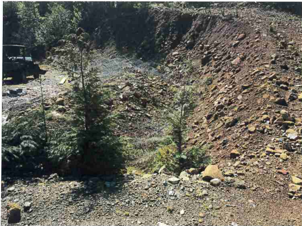
Photo 11. MP13 - Small channel and over-steepened slope.
