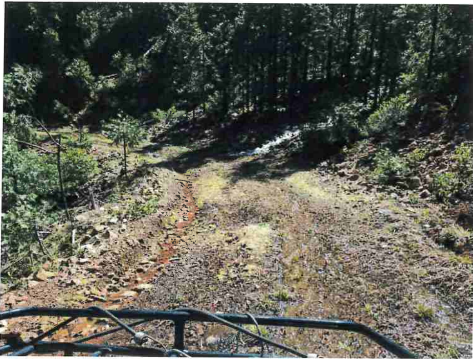
Photo 1. MP4 - Road surface at fill crossing.
