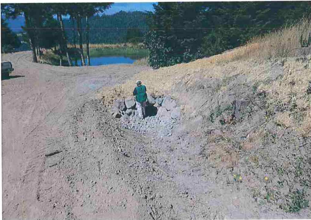
Photo 12: DRC inlet below cut bank slump. DRC inputs into pond.
