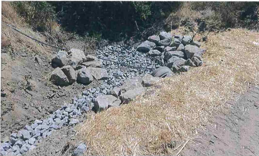
Photo 9: Ditch input (left) from road with connectivity to Garden #3; 24" culvert inlet on Class III.
