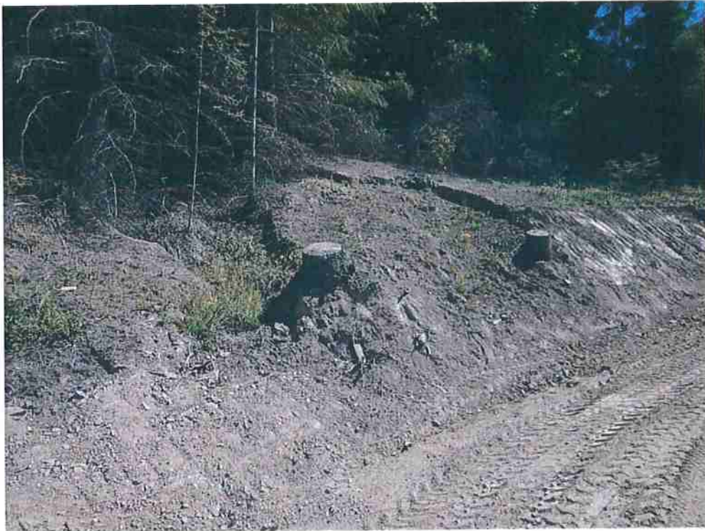
Photo 11: Cut bank slump on road above pond. Corrective Action 4.
