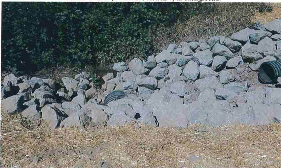
Photo 14: Looking downstream at 24" culvert outlet (center) of stream xing, and pond overflow culvert outlet (right).
