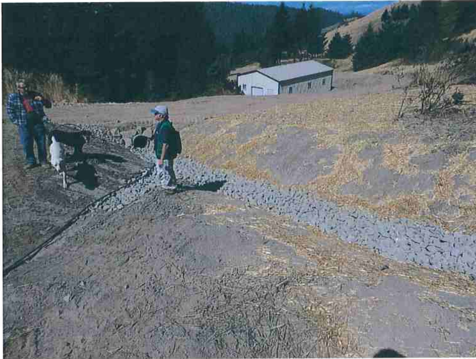
Photo 3: Looking downstream at 24” culvert inlet. Class III on right, drainage from flat (Garden #1) on left. Revegetate bare slopes here. Corrective Action #2.
