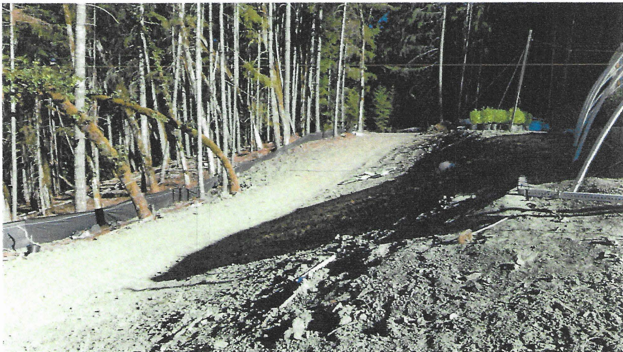
Picture 1 + 2: These are photographs of ECP #1. This exposed bare mineral earth occurs throughout Cultivation Site #1. This site will be straw mulched and seeded to mitigate potential erosion. Photo date: 08/11/2016
