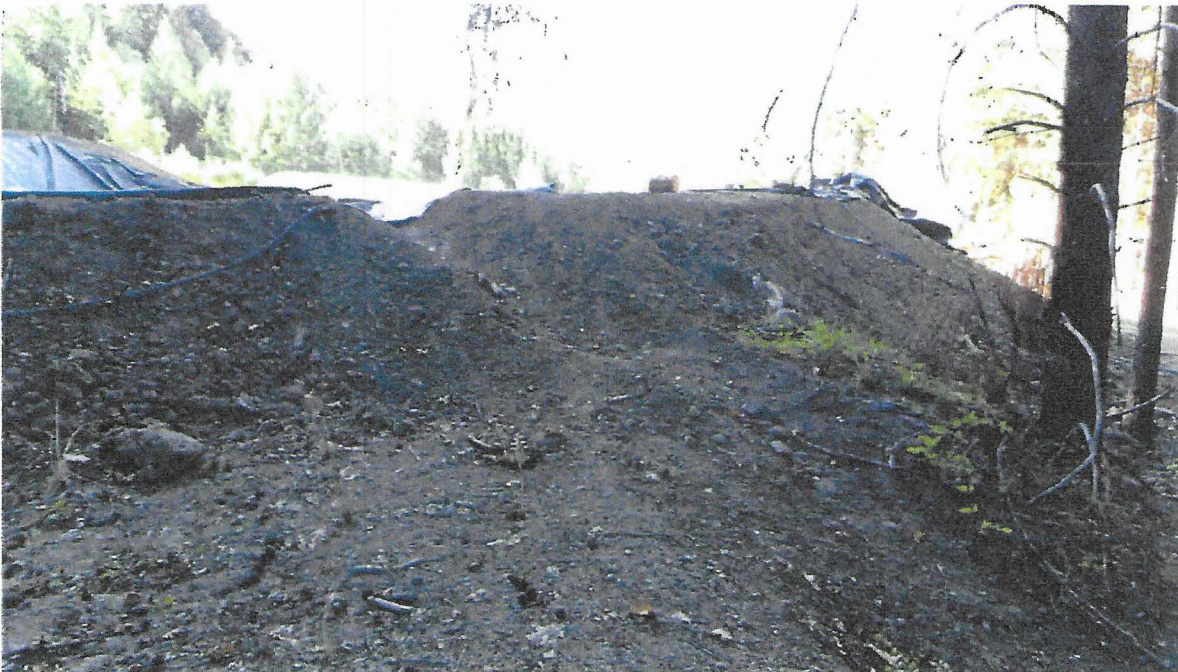
Picture 3 + 4: These are photographs of ECP #2. The Discharger will install an 8" diameter plastic flex pipe for the winter of 2016-17. Rock armoring shall be installed in 2017 when machine operations resume. Photo date: 08/11/2016
