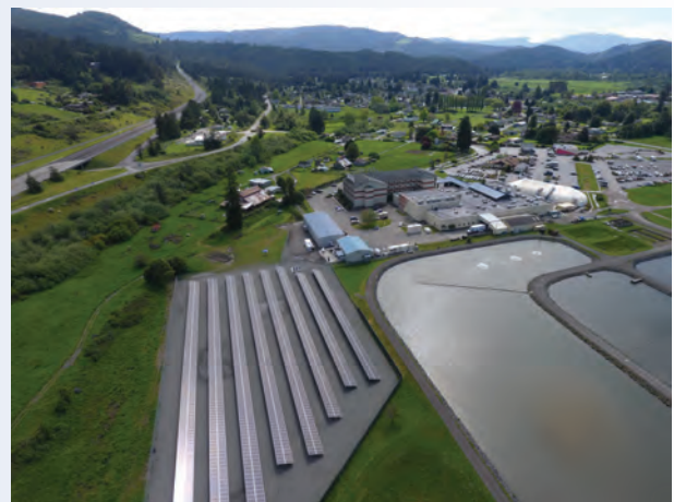
Aerial view of the Blue Lake Rancheria 500kW solar array within the Tribe's low-carbon community microgrid (Photo: Blue Lake Rancheria)
