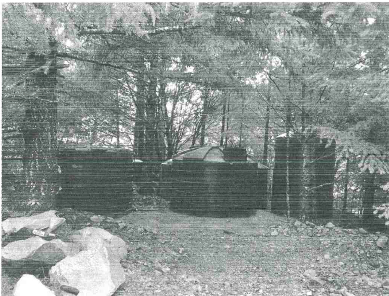
Picture 14: This is a photograph of four 5,000 gallon water tanks, which are plumbed to the shop's gutters. The landowner intends on adding additional storage tanks at this location to harvest rain water in order to comply with the forbearance requirements. Photo date 12-22-2015
