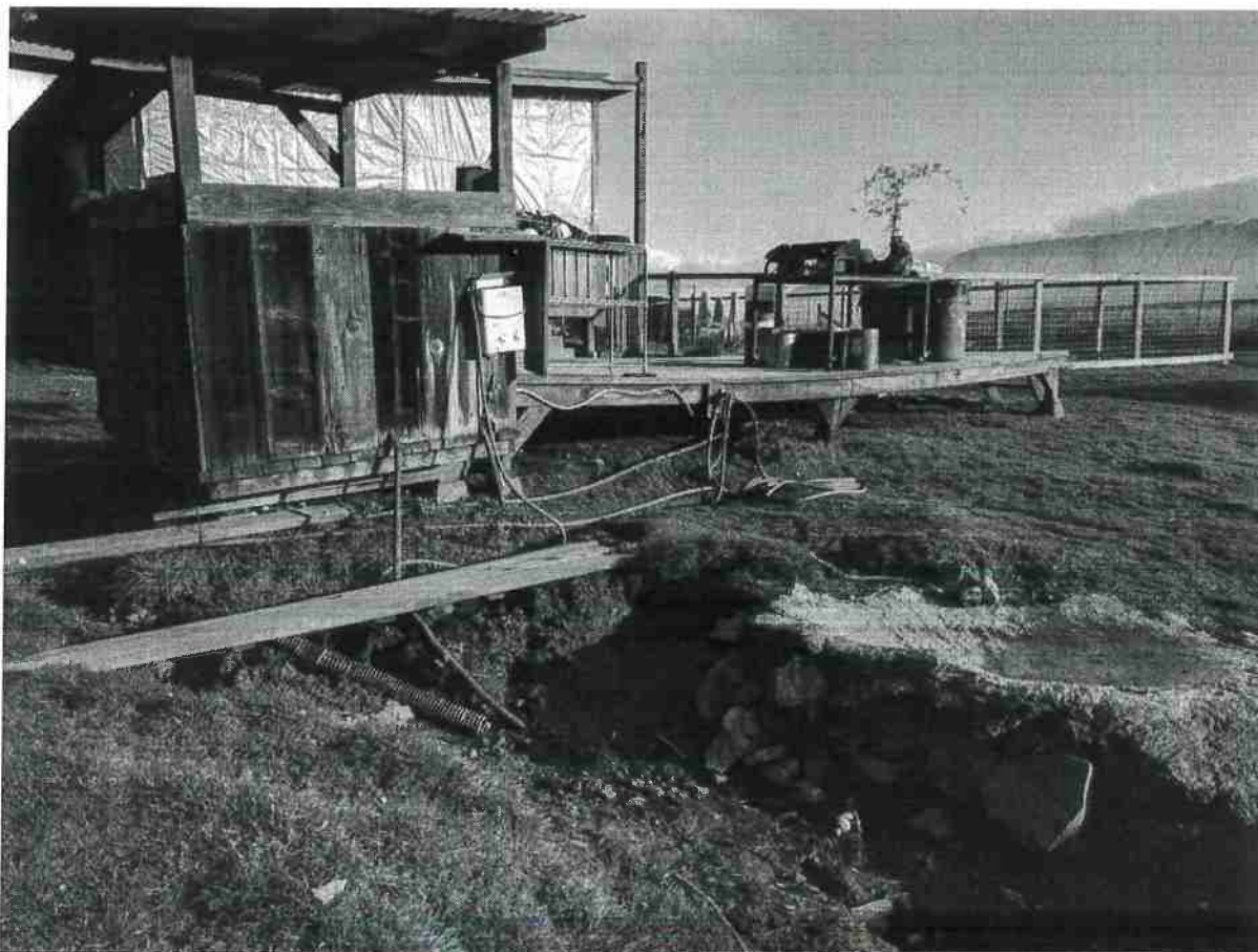
Photograph #45– Structure within Class III watercourse riparian area; Upstream of SC8; Further consultation with county and state agencies to determine variance options
