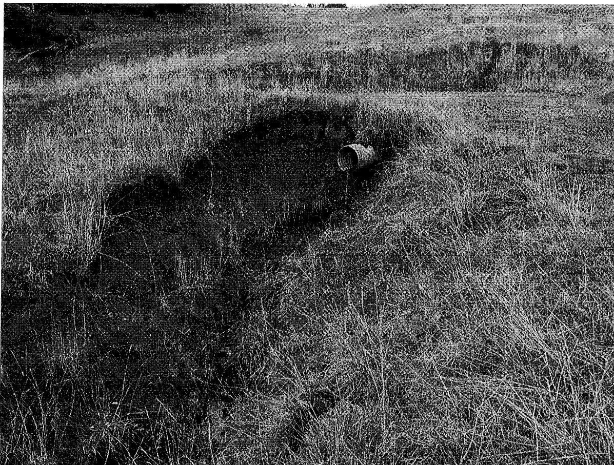
Photograph #24 – At Stream-Crossing #11 view-upstream; inboard ditch (spring) relief culvert that is hydrologically connected to watercourse associated with Stream Crossing #10
