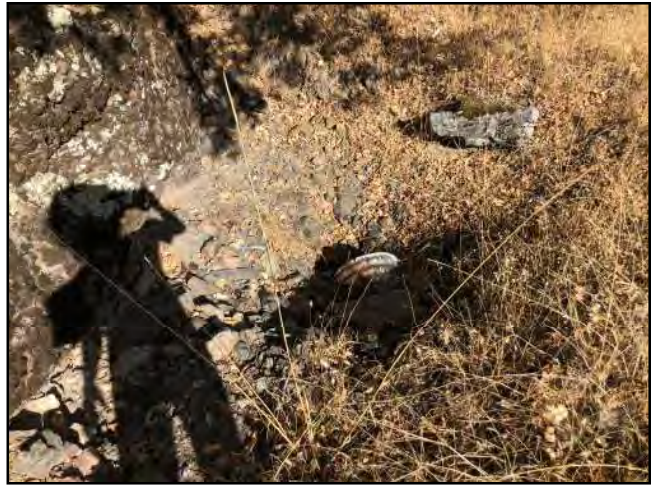
Photo #26 Unnamed Main Rd Looking @ Partially Clogged 18" Culvert In
