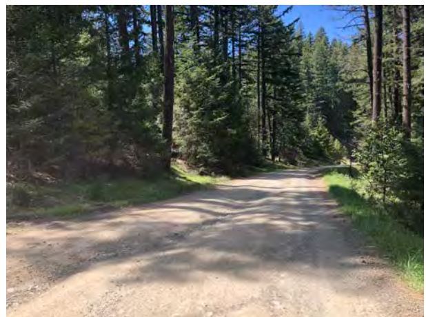
Photo #234 Access Road Looking SW w/ Erosion
