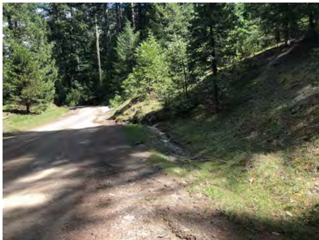
Photo #221 Access Road @ Curve w/ Erosion Issue
