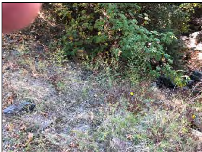
Photo #446 Unnamed Main Rd Looking @ Clogged Culvert Out (size was not identified)
