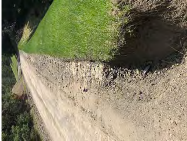
Photo #183 Access Road Looking SE w/ Drainage Issue
