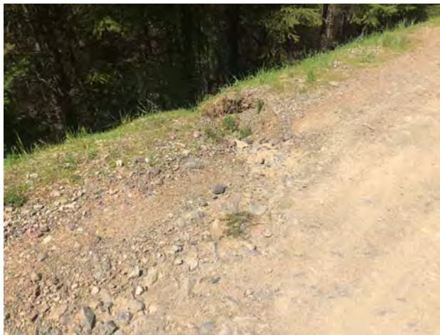
Photo #209 Access Road Erosion Issue
