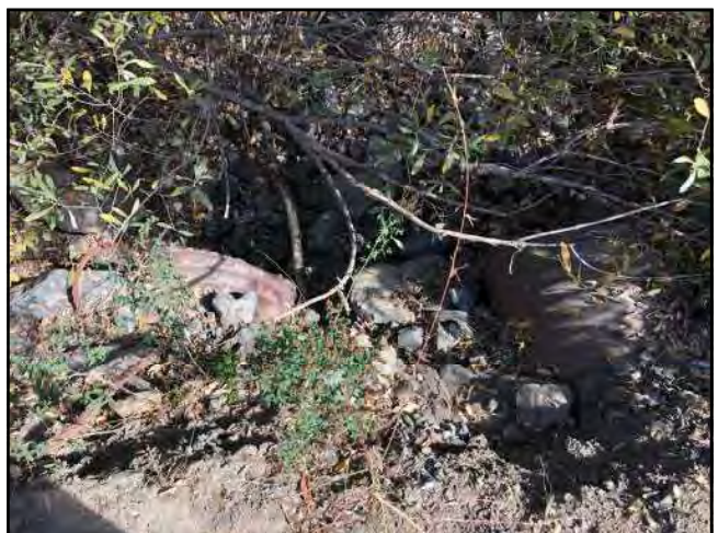
Photo #459 Unnamed Main Rd Looking @ Crushed Culvert In
