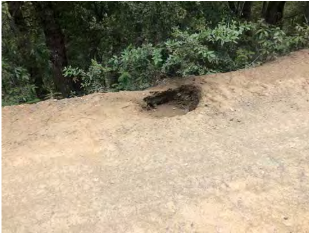
Photo #79 Access Road w/ Drainage & Erosion Issue
