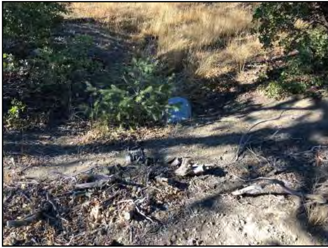
Photo #121 Unnamed Main Rd 18" Culvert Out
