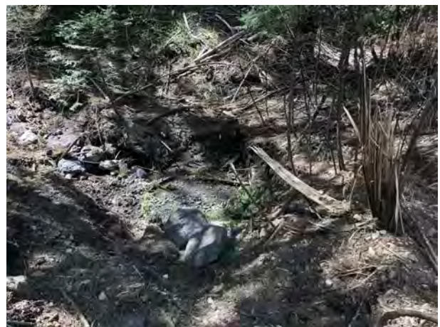
Photo #222 Access Road w/ Hillside Slide
