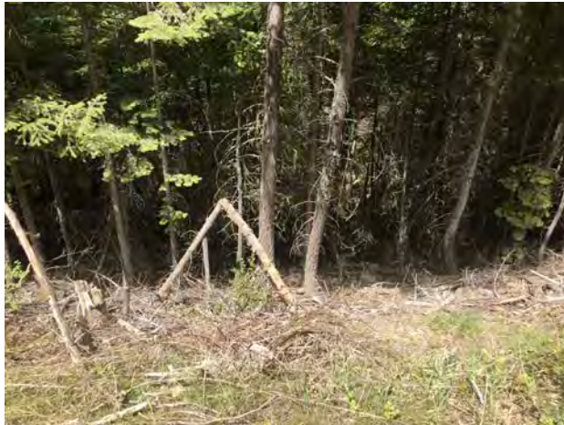
Photo #133 Access Road Culvert Out
