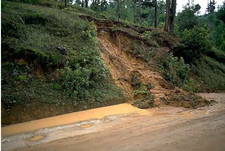
Figure 21. Cut bank failure blocking inboard ditch. Cut bank failures cause operational and maintenance problems, especially when chronic. Source: Keller and Sherar 2003.
