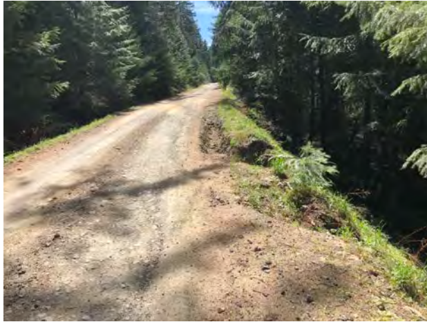
Photo #213 Access Road Looking SW w/ Erosion Issue
