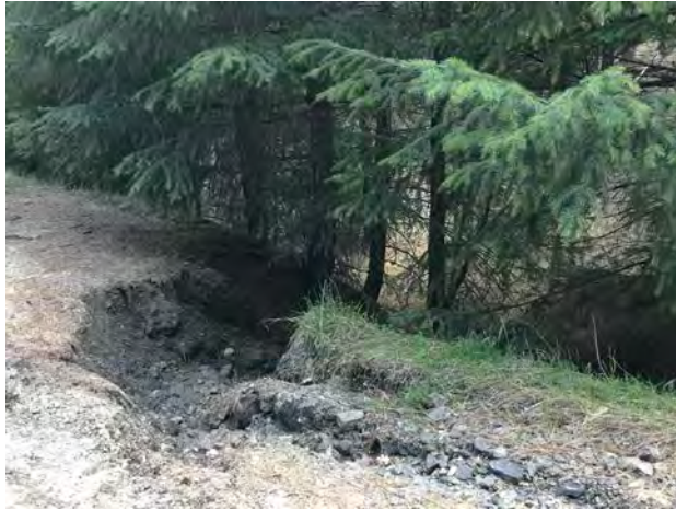
Photo #201 Access Road Erosion from Improper Drainage
