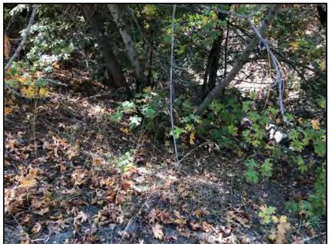
Photo #447 Unnamed Main Rd Looking @ Clogged Culvert In (Size was not identified)
