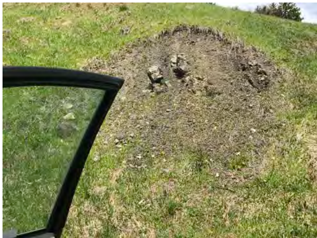
Photo #179 Access Road w/ Hillside Slide
