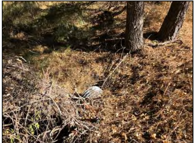
Photo #52 Unnamed Main Rd Looking @ Partially Clogged 18" Culvert In
