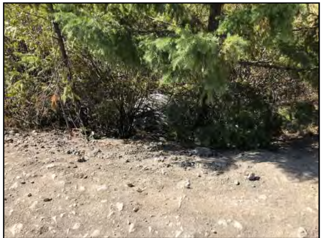
Photo #16 Unnamed Main Rd Looking @ Clogged 18" Culvert Out
