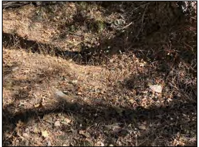
Photo #46 Unnamed Main Rd Looking @ Partially Clogged 18" Culvert In
