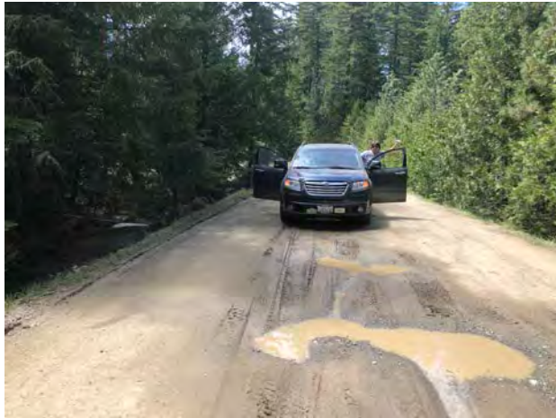
Photo #163 Access Road Looking W w/ Drainage Issues
