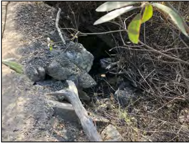
Photo #460 Unnamed Main Rd Looking @ Culvert Out Undermining Road Bed
