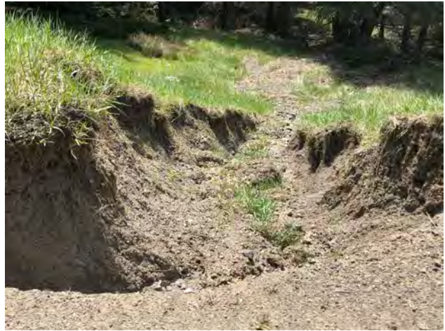
Photo #182 Access Road w/ Drainage Issue
