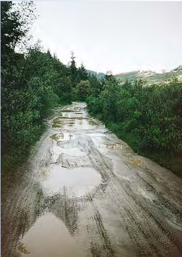
Figure 18. Water collecting on a forest road because of poor drainage. Photo: Jared Gerstein.
