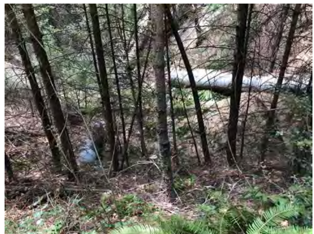
Photo #72 Access Road Looking at Culvert Out
