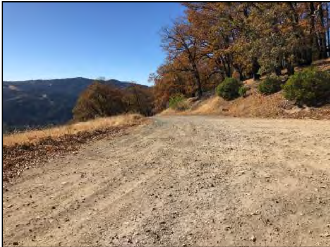
Photo #39 Unnamed Main Rd @ Intersection of Private Access Rd Looking NW @ Curve
