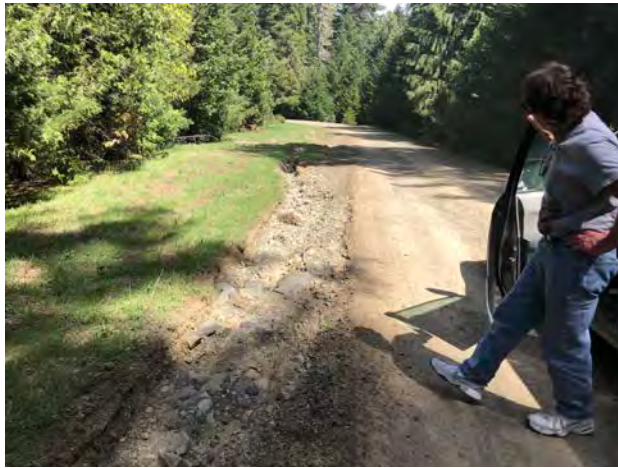
Photo #225 Access Road @ Curve Looking E w/ Clogged Ditch
