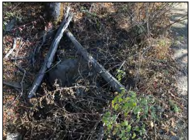
Photo #6 Unnamed Main Rd Looking @ Clogged 18" Culvert In
