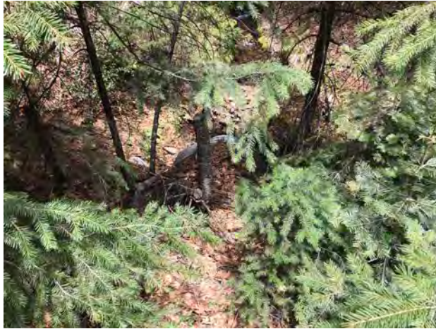
Photo #75 Access Road w/ Culvert Out
