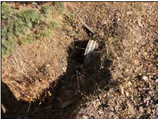
Photo #93 Unnamed Main Rd Looking @ Partially Clogged 18" Culvert In
