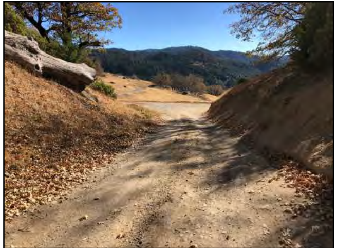
Photo #40 Unnamed Main Rd N/O Intersection of Private Access Rd Looking SE @ Pvt Access Rd
