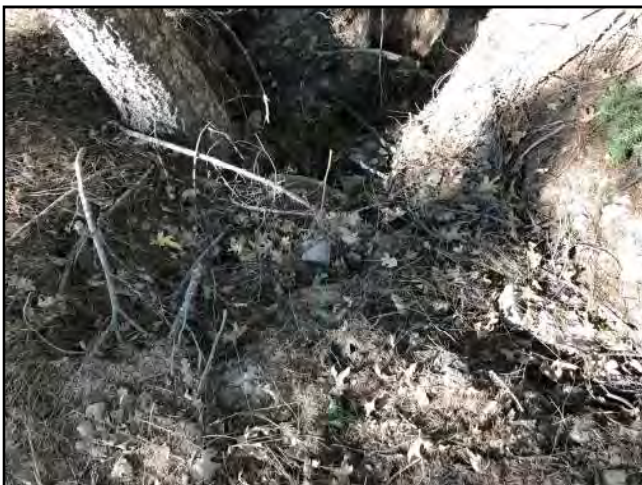
Photo #47 Unnamed Main Rd Looking @ Partially Clogged 18" Culvert Out
