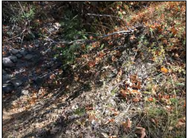
Photo #445 Unnamed Main Rd Looking @ Clogged Culvert In (culvert out wasn't identified)
