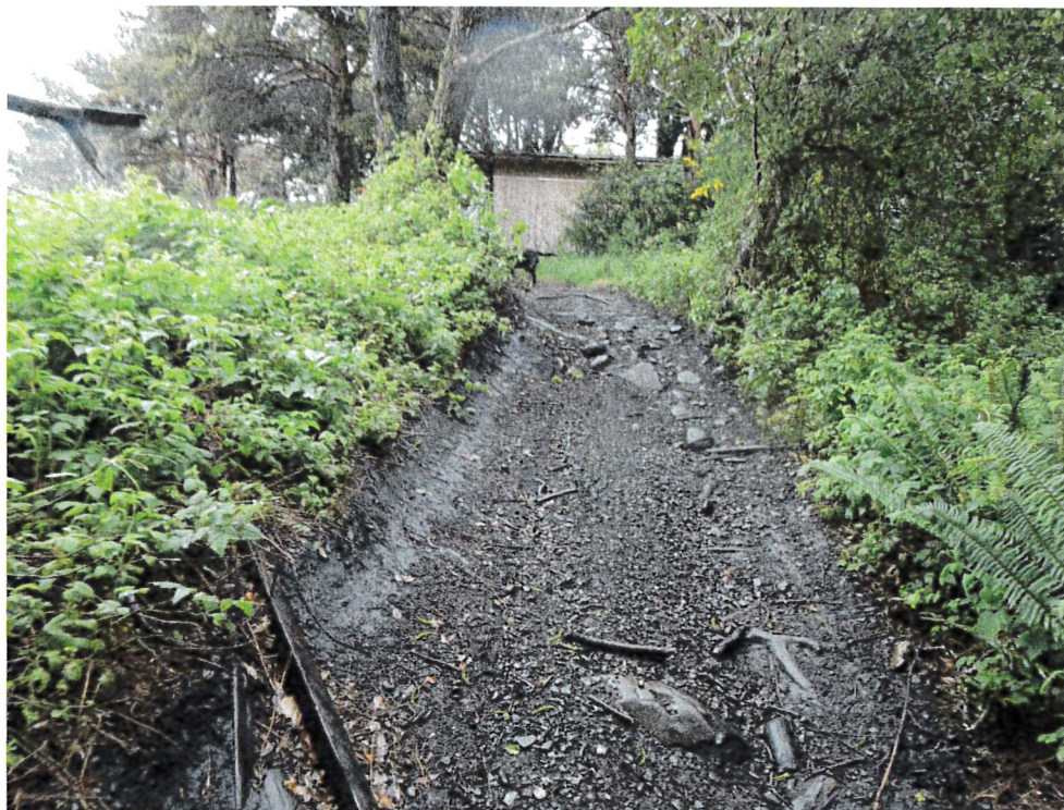
Photo 1 – Surface erosion on a steep section of the Quad Trail.
