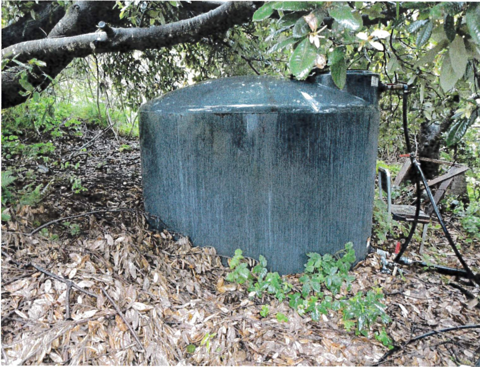
Photo 7 – 1,500-gallon water storage tank near Greenhouse #1.
