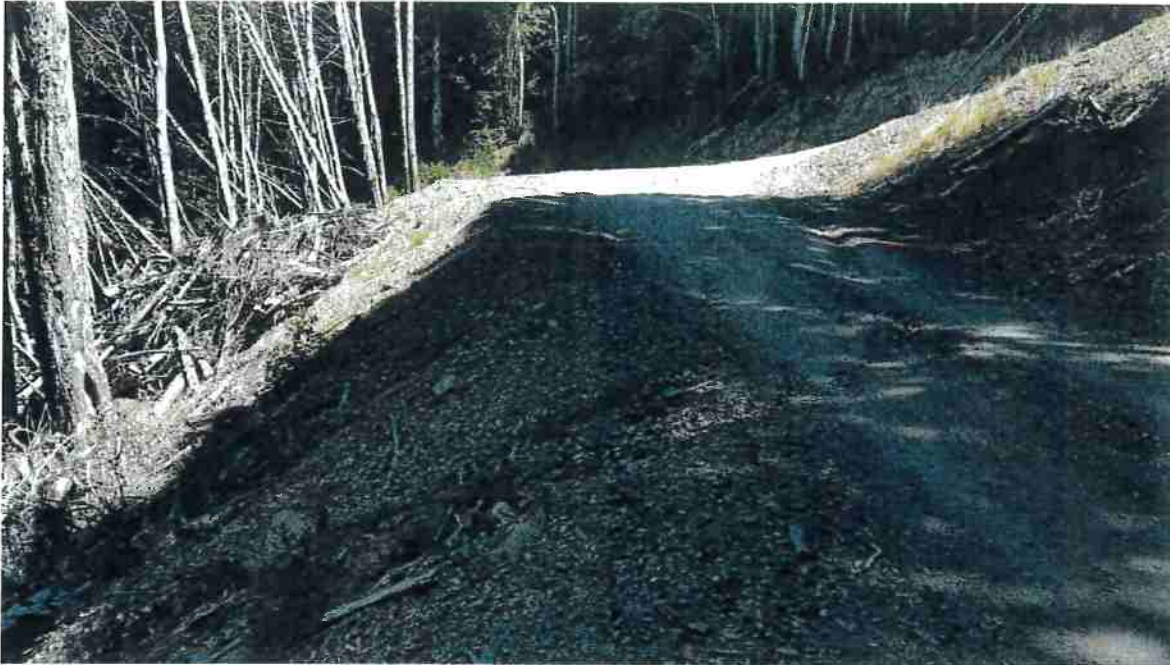
Picture 7: Road Point 5, the Discharger will apply road rock to the three-way intersection to secure the roads surface and slope.
