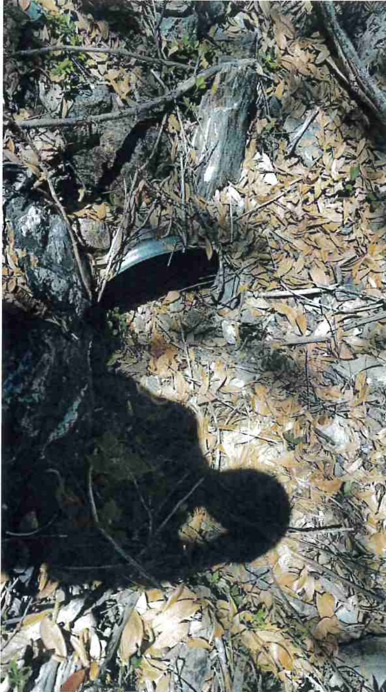
Picture 13: Road Point 12, Class III watercourse crossing with a 24-inch diameter corrugated metal pipe. This culvert is beginning to plug with native rock material from around the inlet. Removal of this debris is recommended before winter to prevent further accumulation of debris resulting in severe plugging of the culvert.
