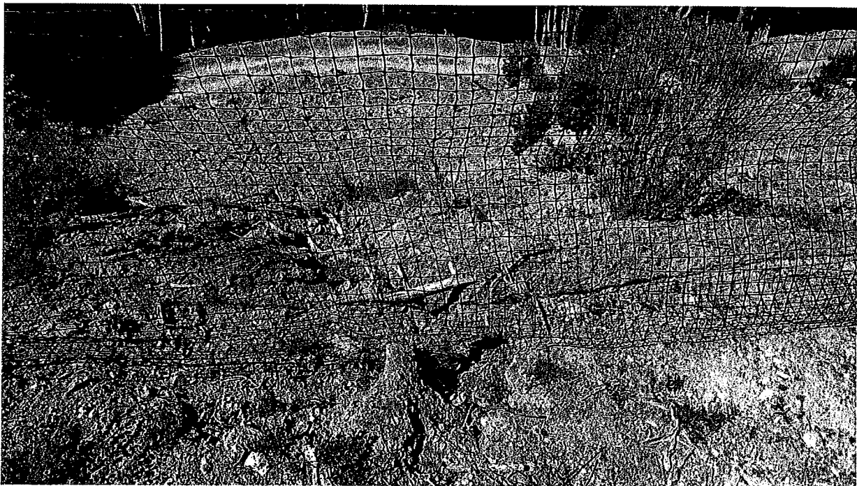
Picture 11: Looking down the fill slope from Map Point 1 showing the beginning of erosion rilling and gullyng.
