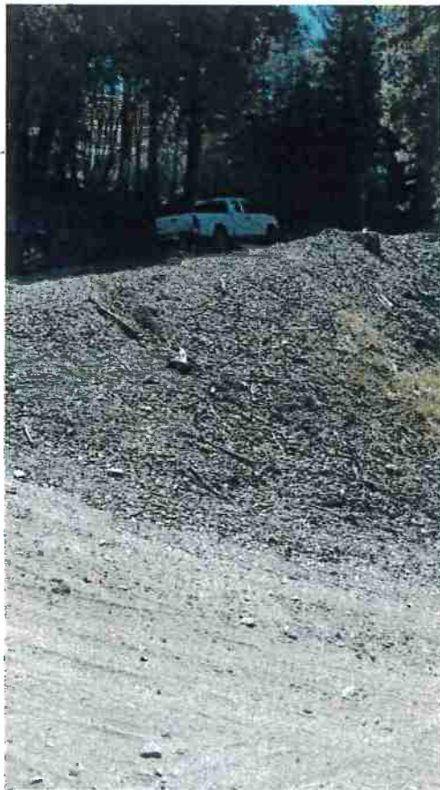
Picture 6: Road Point 4, the fill slope will be stabilized by placing rock on the inside corner and spreading seed to vegetate the rest of the fill slope.
