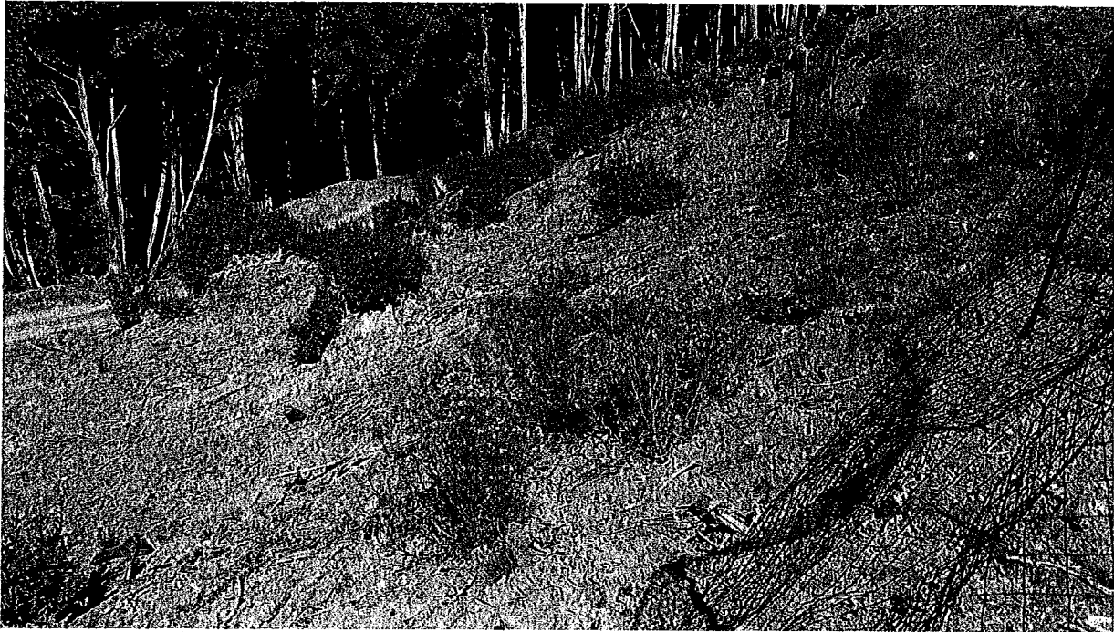
Picture 10: Looking down at the eroding fill slope below Map Point 1.
