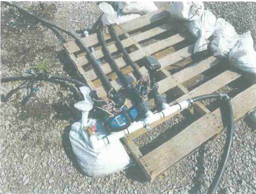
Timed irrigation valves and wasted water.
