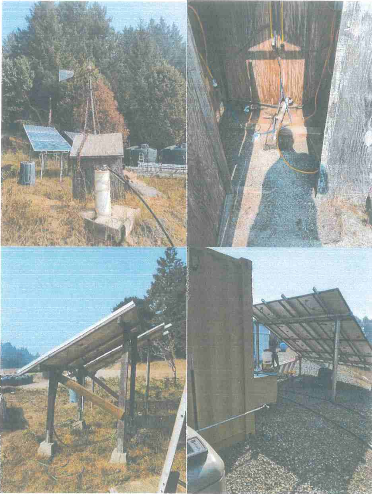
Both wells and two of the solar arrays that provide primary power to the project.
