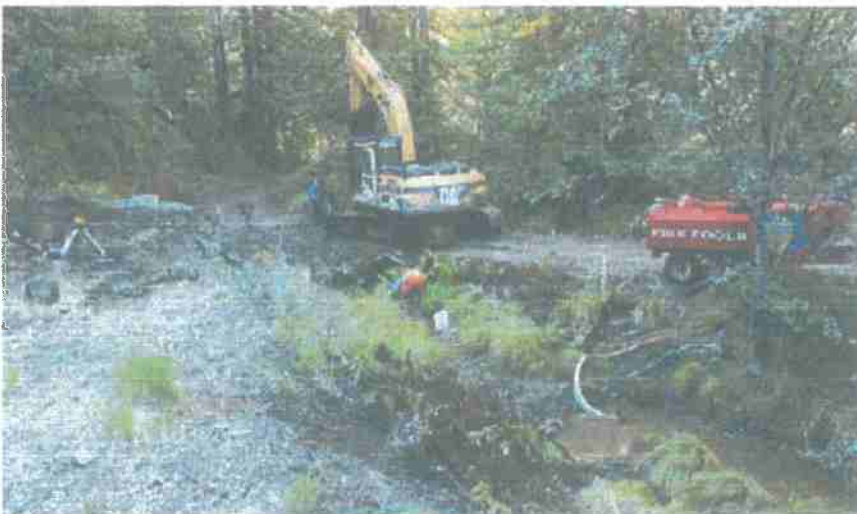
FIGURE 199. For larger streams, pump trucks, large pumps or multiple small pumps can be used to pump streamflow around project work sites. Here, a pump truck is used to temporarily divert flow in a fish bearing stream where dual culverts are being replaced with a raised bridge. Young fish were removed from this fish bearing stream before project work started.
