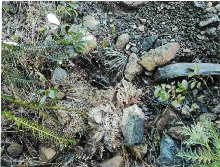
Partially clogged inlet, still functional
