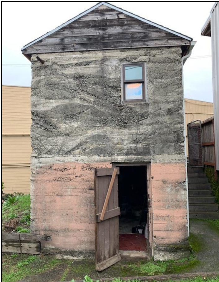
Figure 2: Old 12'x16' Two-Story Ice House to be Replaced with 12'x16' One-Story Modern Ethanol Lab in Same Footprint
