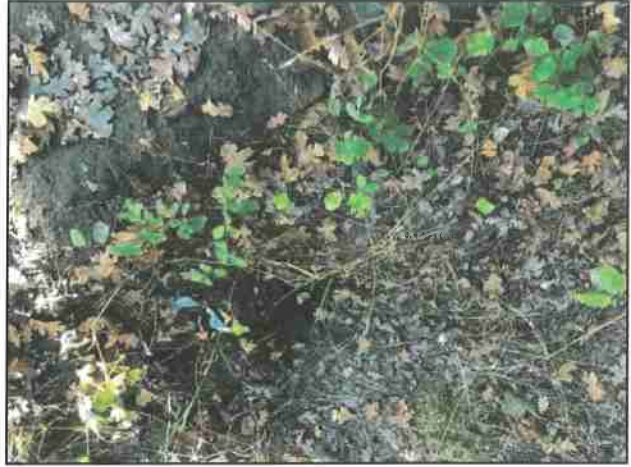
Photo #26 River Rd Looking @ Clogged 12" Culvert Out
