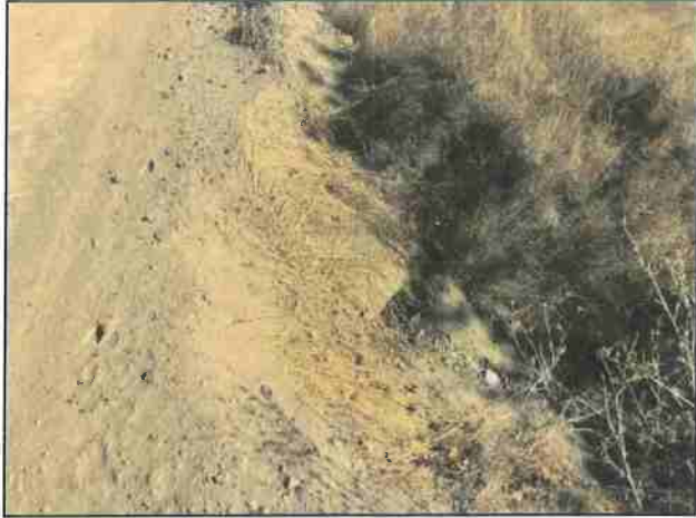
Photo #31 River Rd Looking SE Closeup @ Erosion
