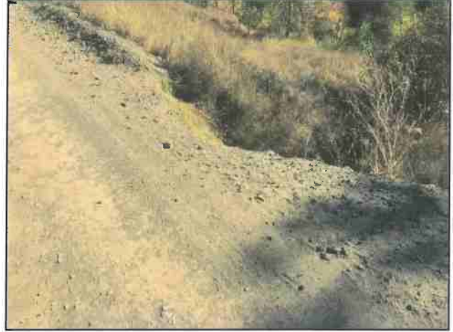
Photo #32 River Rd Looking SE @ Tire Tracks @ Erosion Area
