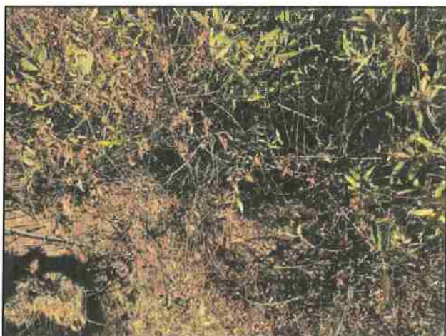
Photo #35 Ridge Rd Looking @ Partially Clogged Culvert In
