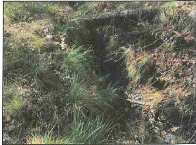
Photo #58 Ridge Rd Partially Clogged Culvert In (Size Unknown)
