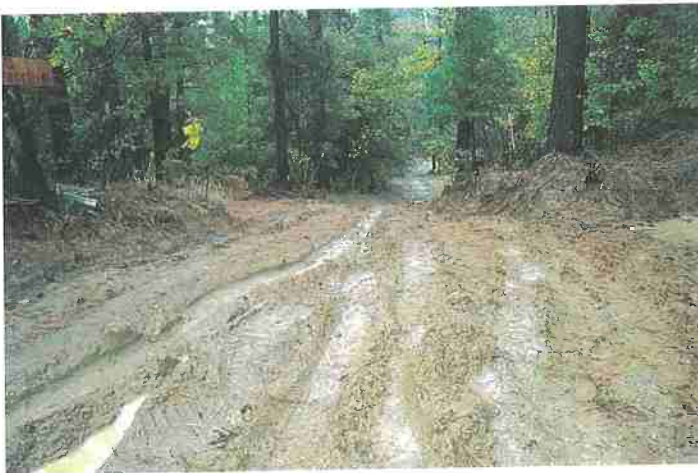
Figure 10. These ruts were created by wet-weather use of an unsurfaced, poorly drained road. Photo: Angela Wilson, Central Valley Regional Water Quality Control Board.
