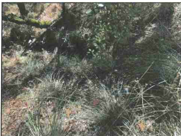
Photo #59 Ridge Rd Partially Clogged Culv Out(- Size Unknown)
