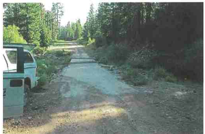
Figure 7. Concreted low-water crossing placed on bedrock outcrop in intermittent stream. Photo: Angela Wilson, Central Valley Regional Water Quality Control Board.
