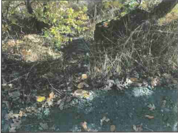
Photo #49 River Rd 12" Culvert Out
