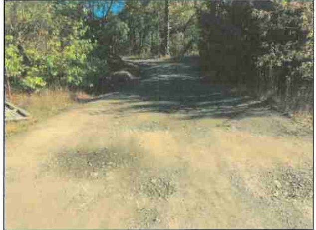
Photo #14 River Rd Looking SE @ Potholing Caused by Poor Drainage
