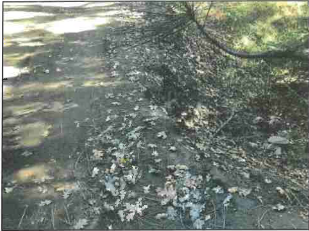
Photo #25 River Rd Looking @ Clogged 12" Culvert In
