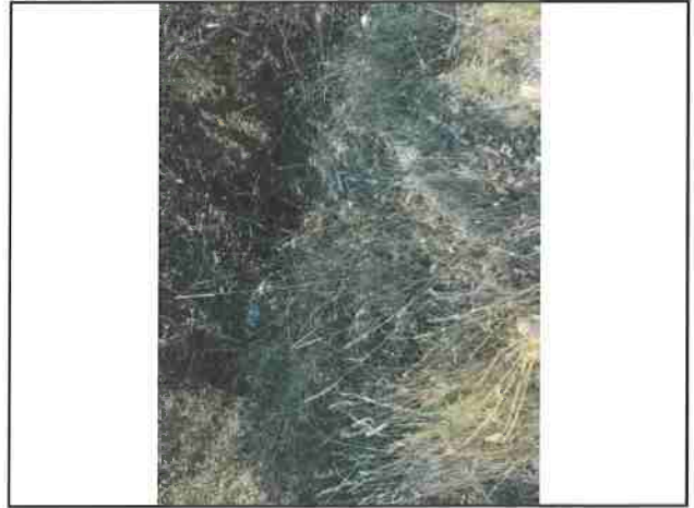
Photo #28 River Rd 12" Clogged 12" Culvert Out
