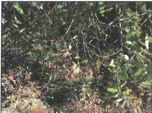
Photo #41 Ridge Rd Looking @ Partially Clogged 18" Culvert In
