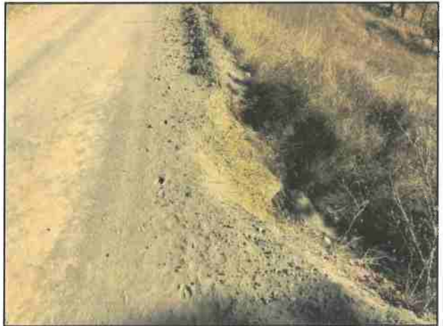
Photo #30 River Rd Looking SE @ Erosion
