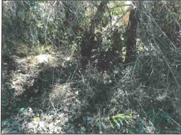
Photo #61 River Rd Looking @ Clogged Culvert In
