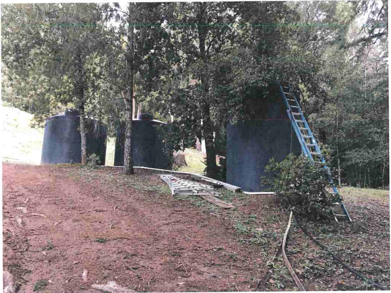
Picture 22: Three five thousand gallon tanks located 150 feet east-northeast from residence. Photo date 12-2-2016.
