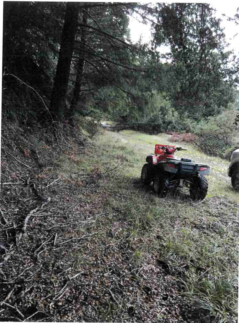
Picture 14: Map Point #3. Picture taken from outlet of Crossing #2 looking southerly to the inlet of Crossing #4. The rock-lined ditch shall be constructed east (photo left) of the access road shown above. Photo date 12-2-2016.
