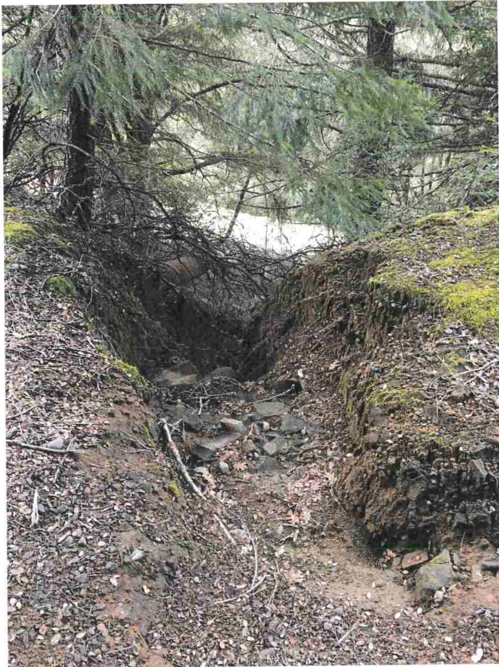
Picture 15: Crossing #4 with the shot-gunned culvert outlet in upper left corner. The erosion is primarily from the Class III watercourse located below Crossing #2, which is diverting onto the access road and discharging across the fill. Photo date 12-2-2016.
