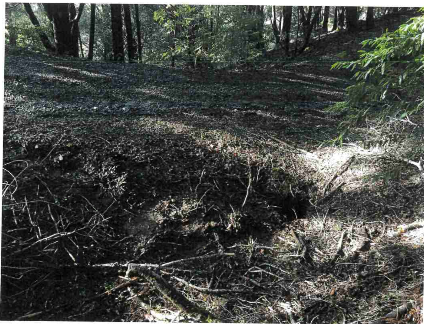
Picture 18: Crossing #5 inlet, which is nearly plugged with organic debris. Photo date 12-16-2016.
