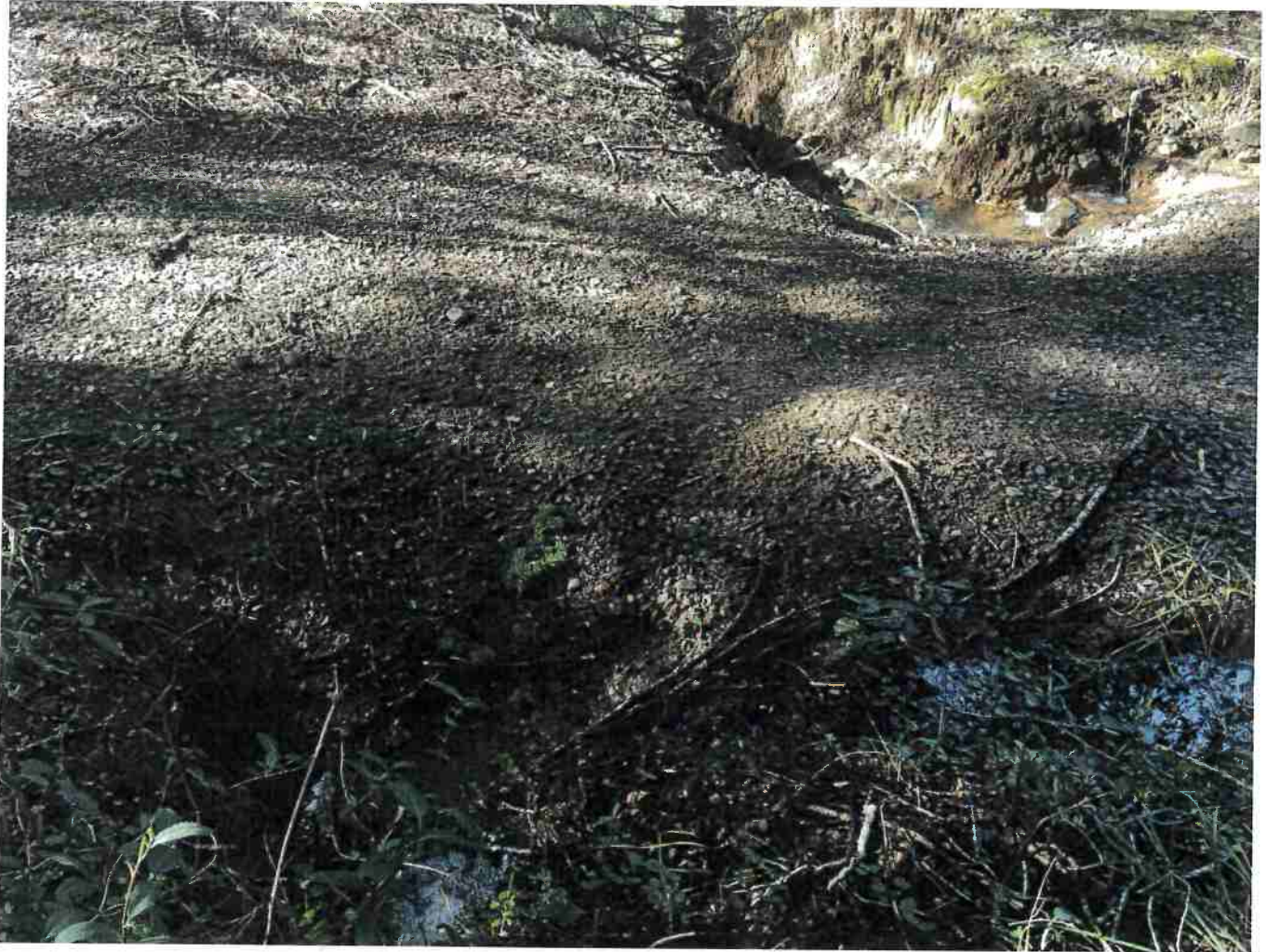
Picture 16: Crossing #4 inlet. The inlet of the 12-inch diameter metal culvert is partially buried and in nearly indiscernible in the lower left hand corner of photo. Photo date 12-16-2016.
