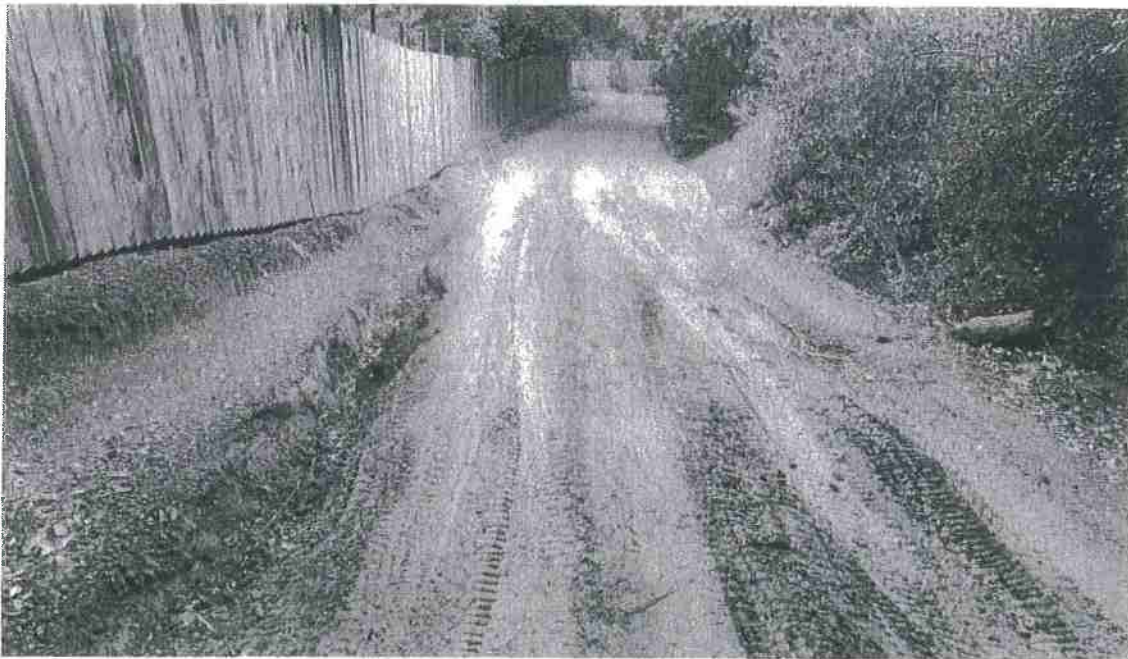
Site 05 looking down grade. Some concentrated road surface runoff is draining off of the road under the gate to the left and contributing to road surface erosion and discharge at Sites 10 and 15.
