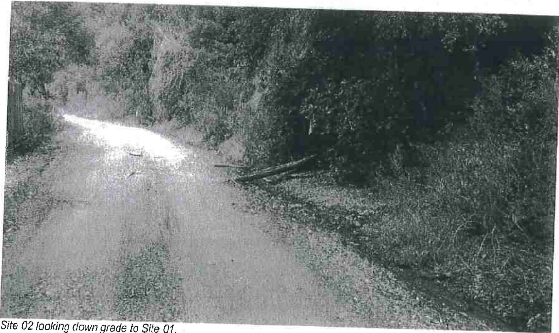
Site 02 looking at the Class III watercourse intercepting the road inside ditch.
