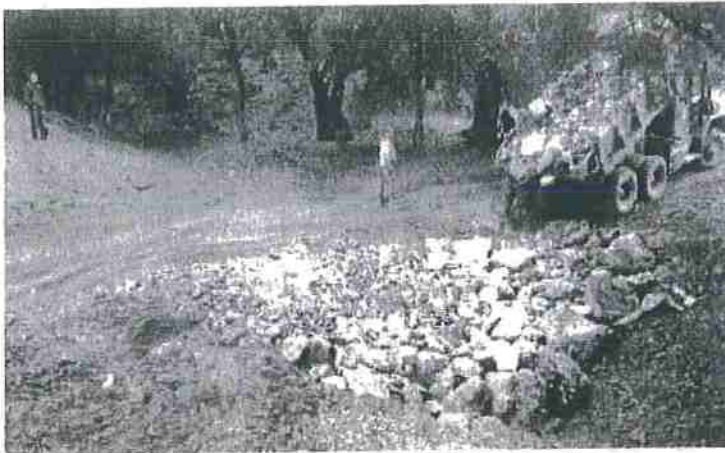
FIGURE 121D. Well graded rock armor is then hauled into the structure and spread across the breadth of the U-shaped stream crossing, and about one-third the way up the roadbed, so that streamflow will only flow over or come in contact with resistant armor material. The armor must be spread and compacted across the design width of the expected flood flow channel width so peak flows will not bank the armored structure.
