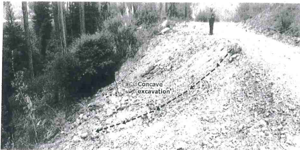
FIGURE 230. The most cost-effective treatment for unstable fills along the outside of a forest, ranch or rural road is simply the direct excavation of the unstable material. If road width is too narrow, additional width can often be derived from cutting into the bank. The excavation should encompass the unstable fill materials, beginning at the inside crack or scarp, and extending out and down the fill slope as far as possible. For proper surface drainage, and to retrieve most of the unstable fill, the excavation should have a concave profile when completed. Typically, the bulk of the fill is within 20 to 25 feet of the outside edge of the road and is easily reached by a midsized excavator. Any remaining fill is likely to be small enough that it will not fail or travel far enough to reach the stream.
