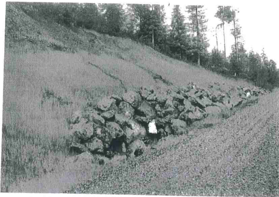
FIGURE 52. This wet and potentially unstable cut slope on a newly constructed road was stabilized using a buttress of large rock armor. To assure their effectiveness, rock buttresses and other retaining structures should be designed by a qualified engineer or engineering geologist.
